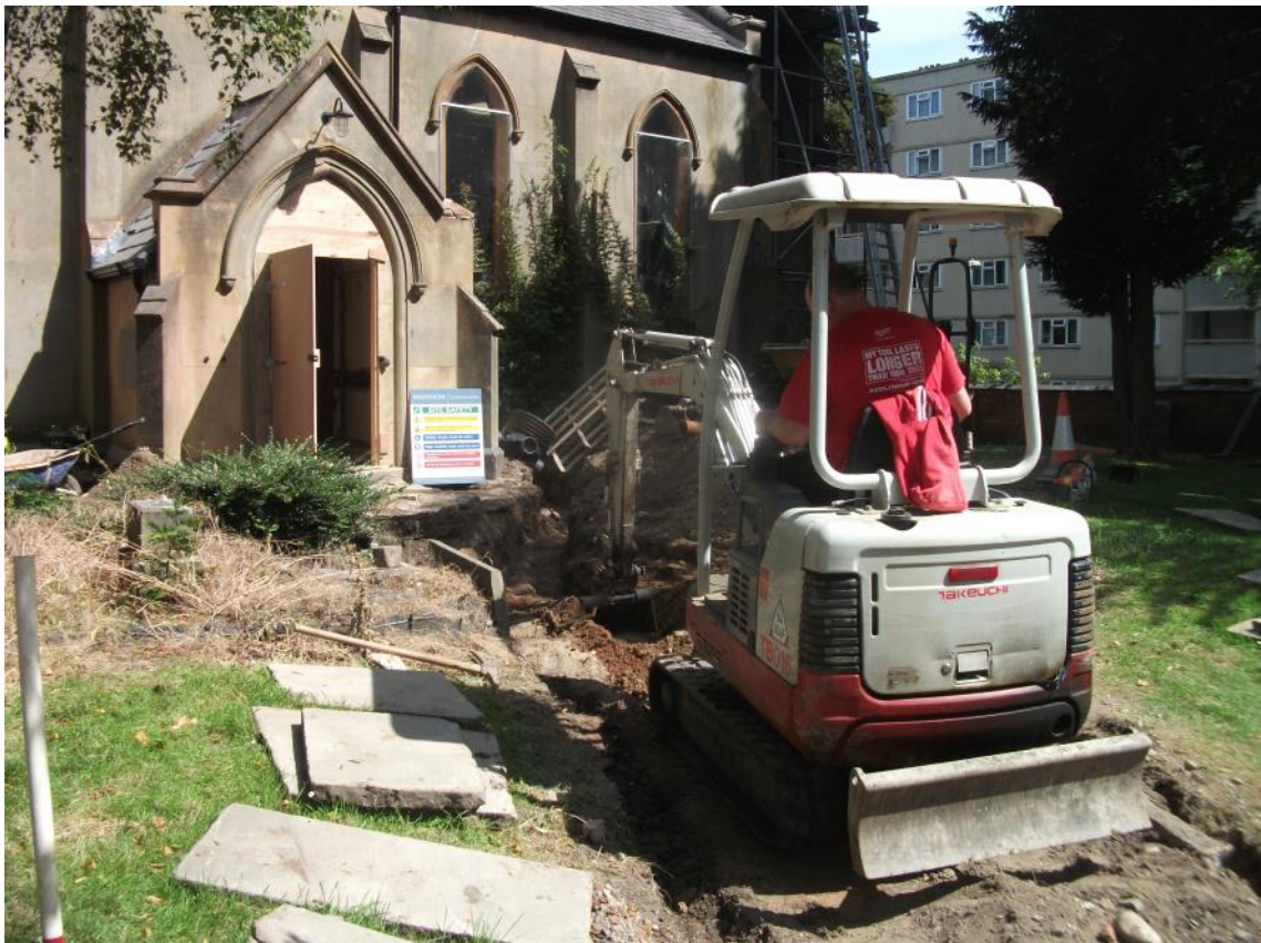
General view of the excavation of the service trenches, looking north Fig 8
