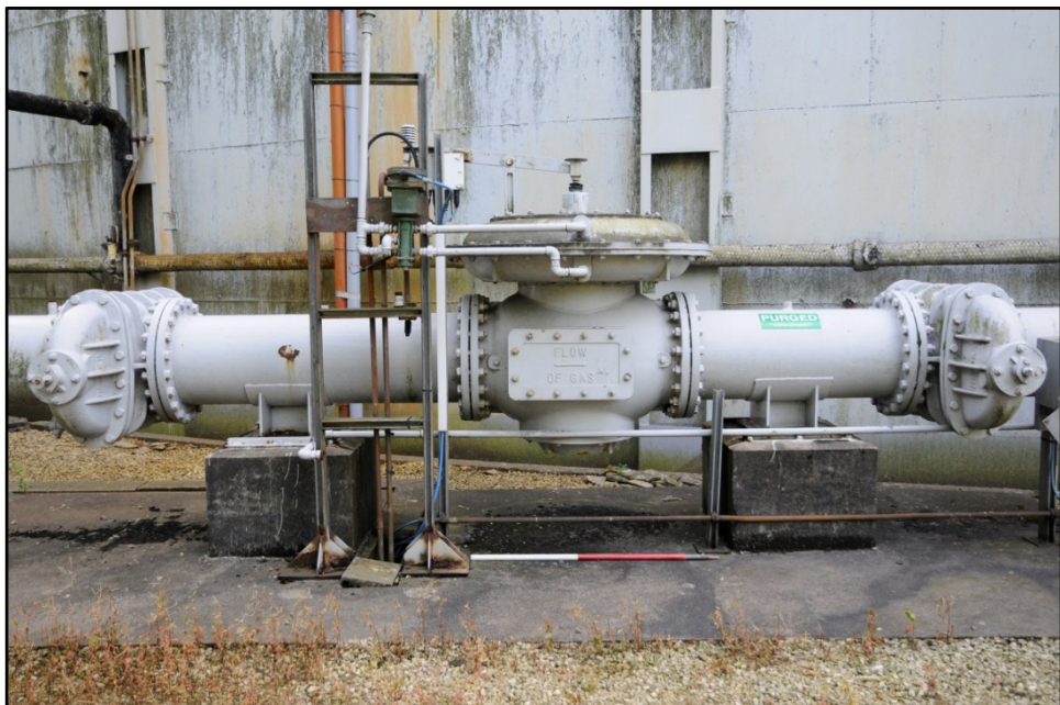
Pipework with flow valves Fig 26
