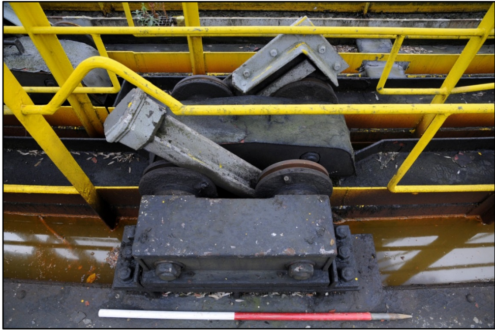
Gear mechanism for the lifting and lowering of the lift tanks Fig 23
