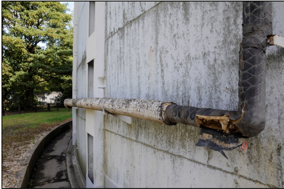
Lagged pipework Fig 15
