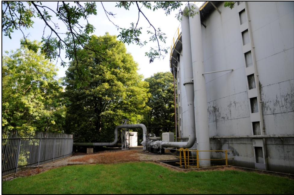
View of external pipework of the western side of the gasholder Fig 29
