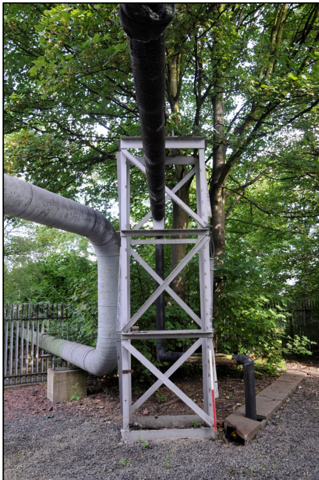
Inlet/outlet pipework and gantry leading over the River Dearne Fig 28
