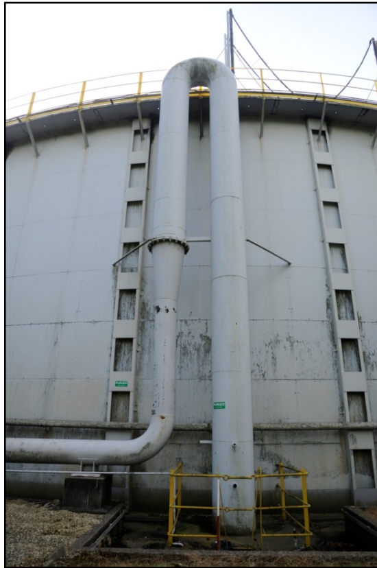
Inlet/outlet pipework on the west of the gasholder Fig 25
