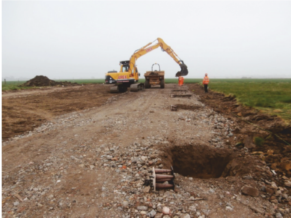
Excavation in progress of the stanchion bases on the south-western side Fig 6
