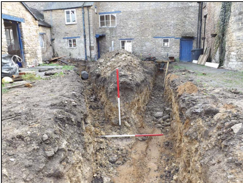
The service trenches at the east of the site, looking east Fig 13
