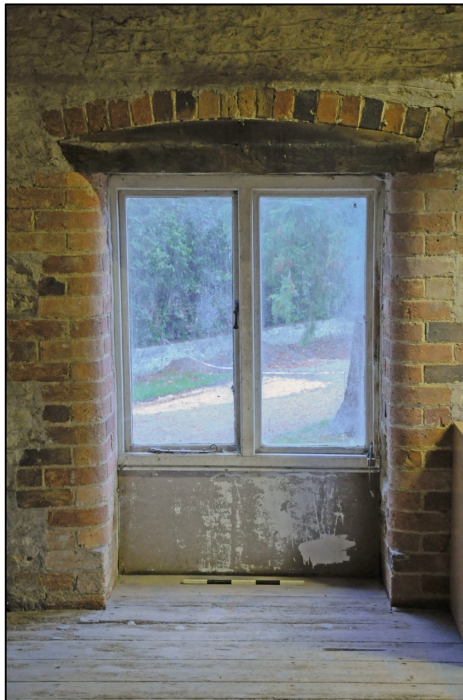
Room F1, former door Fig 18
