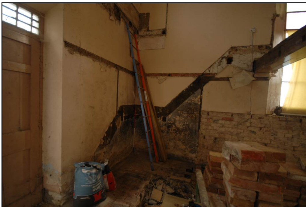
After removal of gallery showing the location of the staircase, looking south Fig 18
