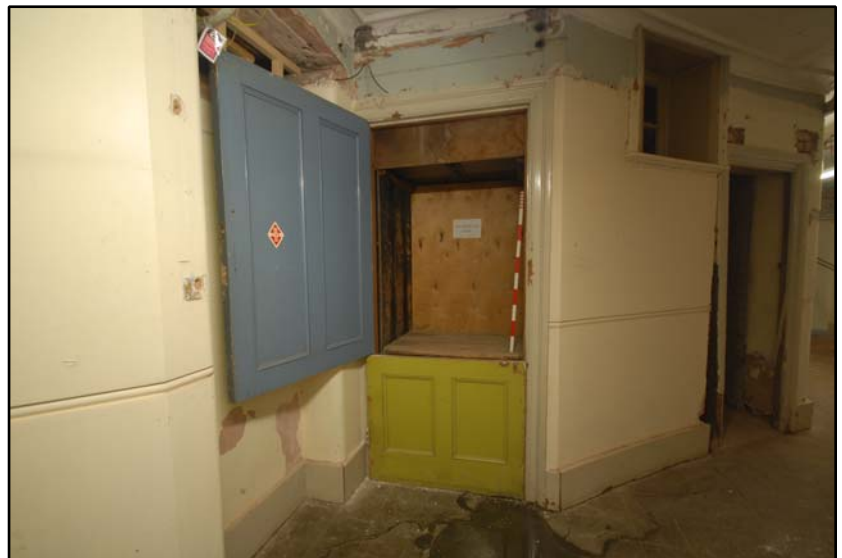
Dumbwaiter elevator adjacent to cellar landing Fig 4.2.2
