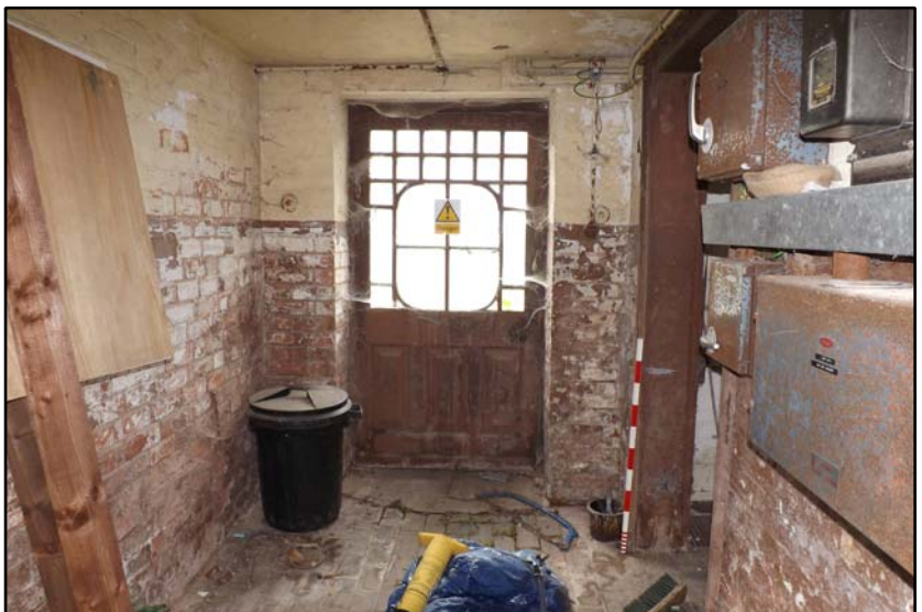
Entrance hall of the Bothy with door to the Peach House Fig 5.7.9
