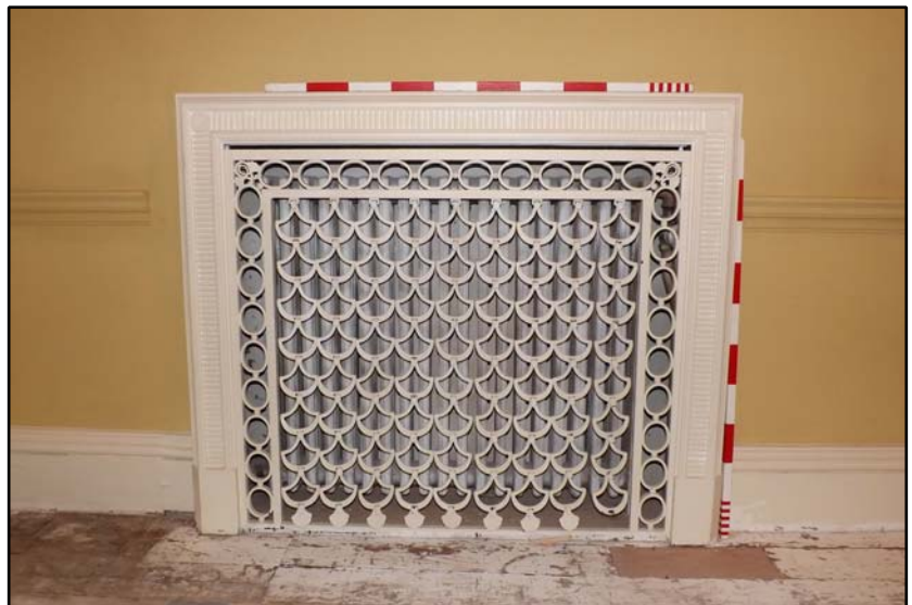
Detail of first floor radiators with decorative coverings Fig 4.5.46
