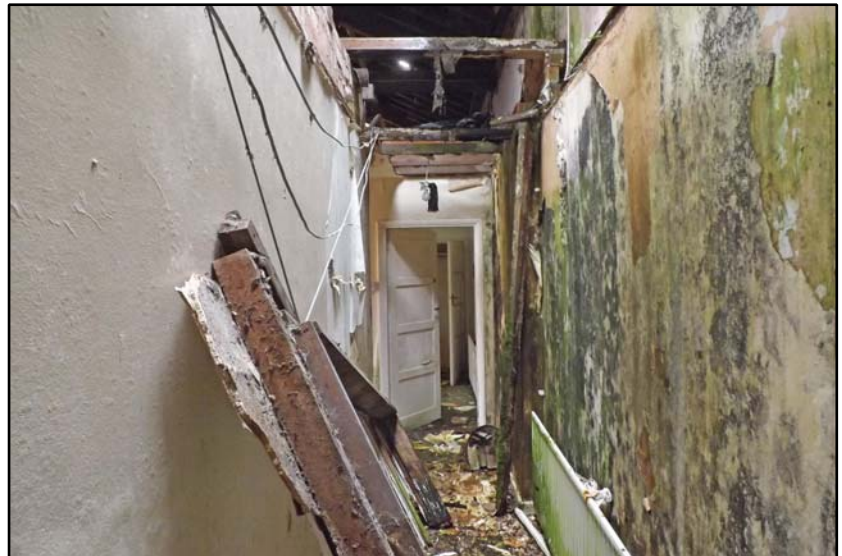
Interior of the 1950's extension, showing its poor condition Fig 5.1.20
