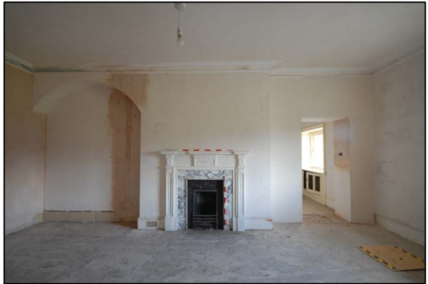
Room S7, the west elevation Fig 4.6.16
