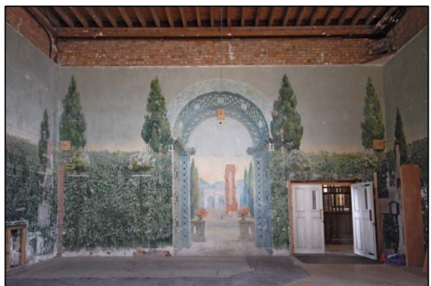
The trompe l'oeil painting on the east wall of the badminton court Fig 4.3.3
