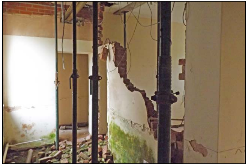
Interior of the south wing, showing the poor condition of the building Fig 5.1.13
