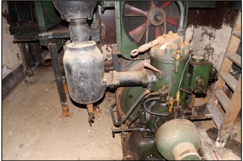
Diesel generator in the air raid shelter Fig 4.4.38
