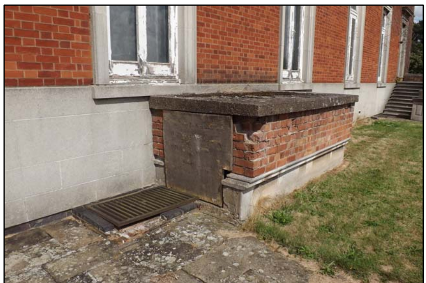
Former stair to the air raid shelter below the theatre wing Fig 4.1.27
