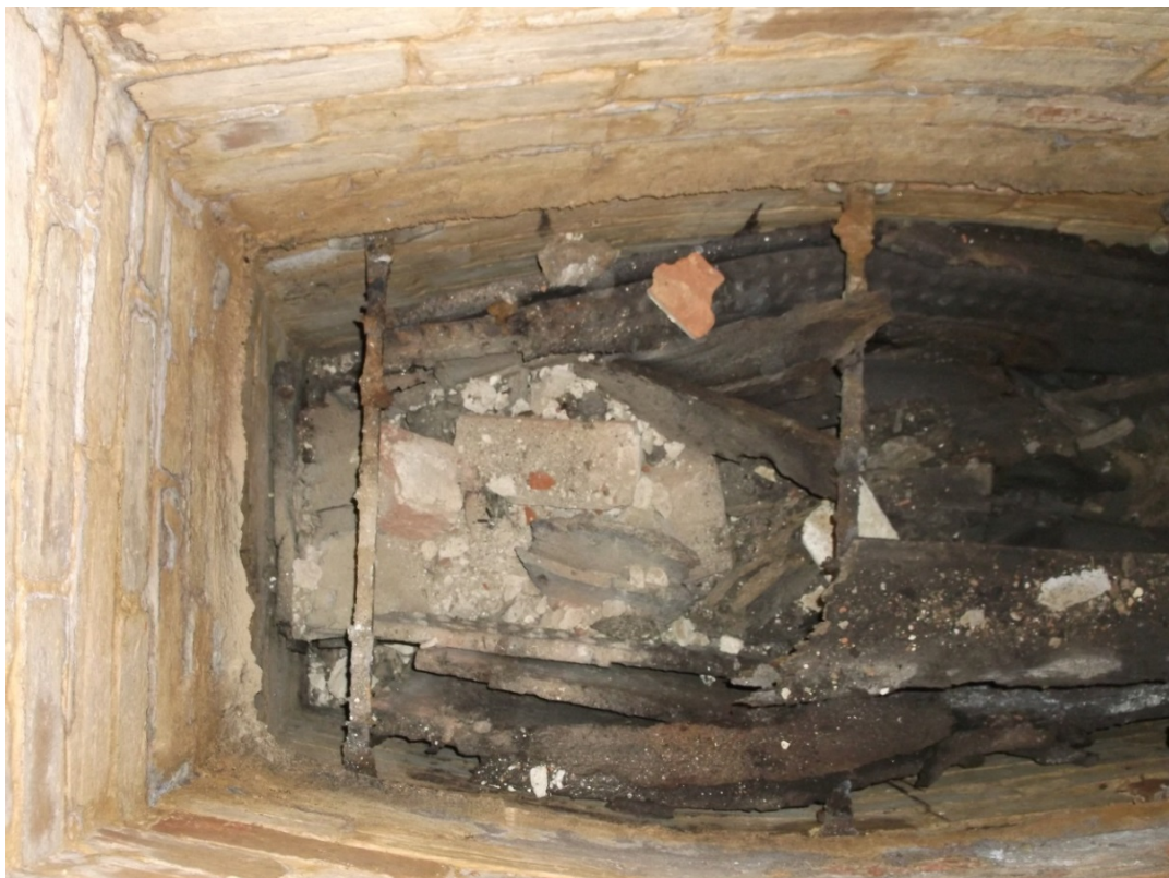
Vault (303), west end of interior showing debris from damaged vault roof Fig 8
