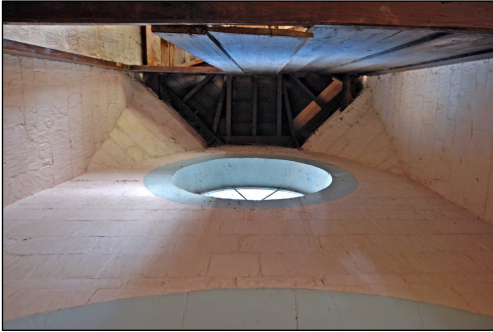
The interior, south face of the lantern, showing the central clock window and stone supporting piers Fig 35
