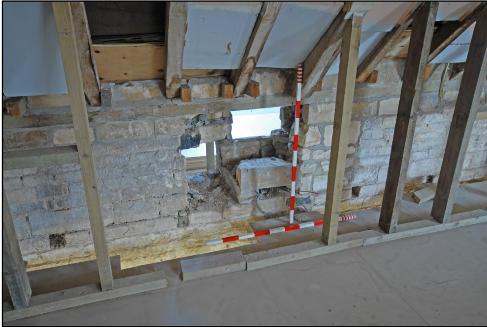
Detail of blocking opposite to the tie beam, also showing defunct joist slots, looking north Fig 49
