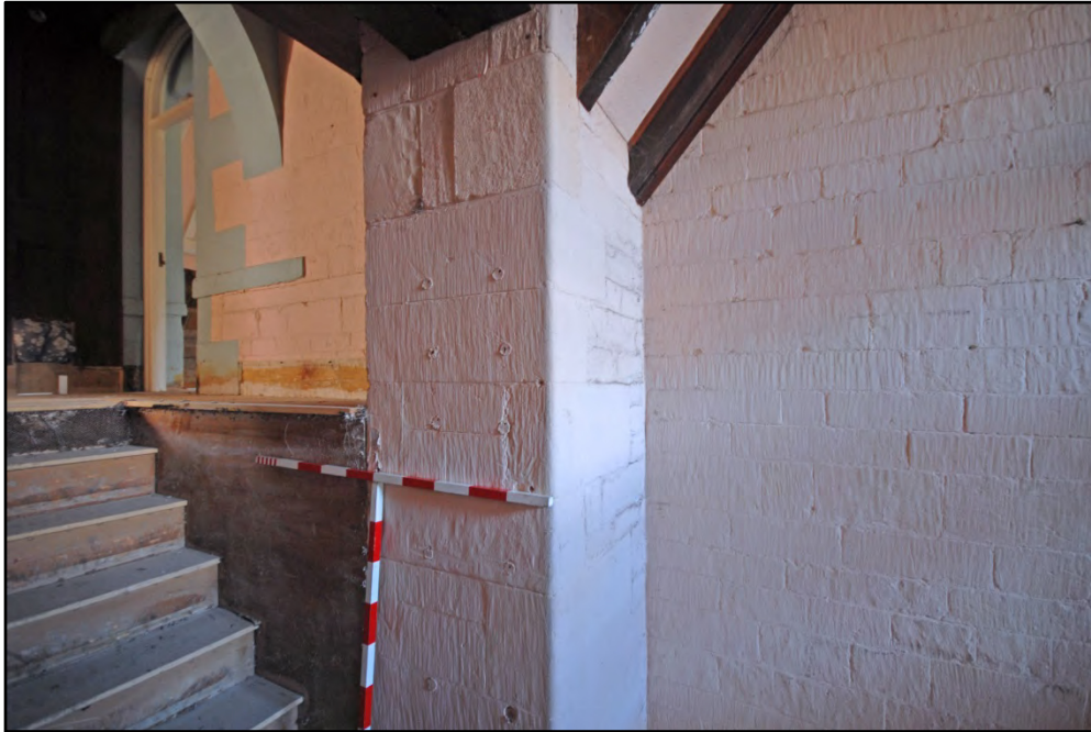
The intermediate landing, showing the quoins of a former door or window opening in the central dividing wall, looking south-west Fig 33
