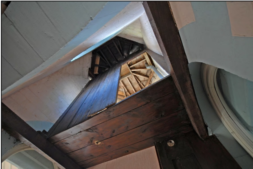
The interior of the lantern with partitioned area over the landing, looking north-west Fig 36
