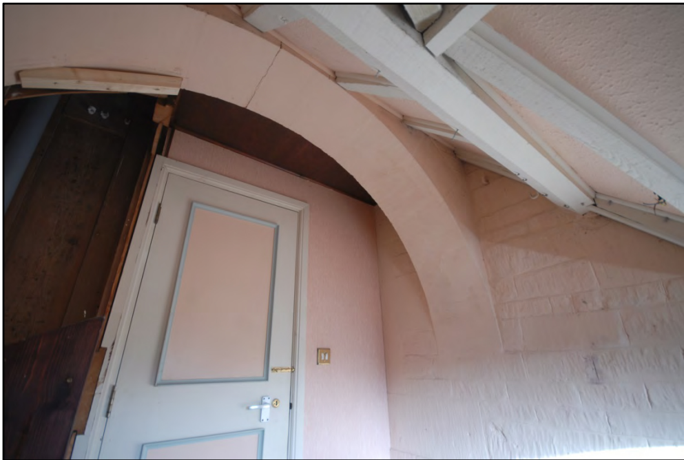
The stone arch supporting the south face of the arch, as seen from within the WC Fig 38
