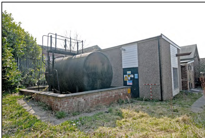
Generator and tank, looking south-east Fig 53
