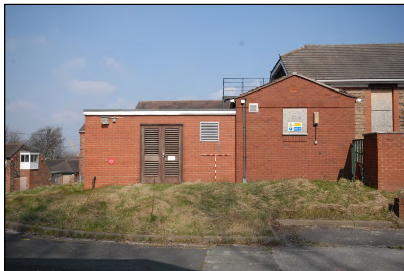
Ward Block 3, boiler house, looking north Fig 11
