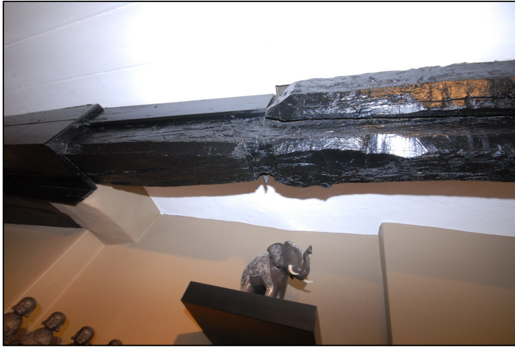
Section of beam on the ground floor at location of reinstatement of stairs Fig 5
