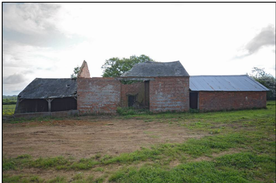
The west elevations of the Cart shed, Barn and Stable, looking north-east Fig 9
