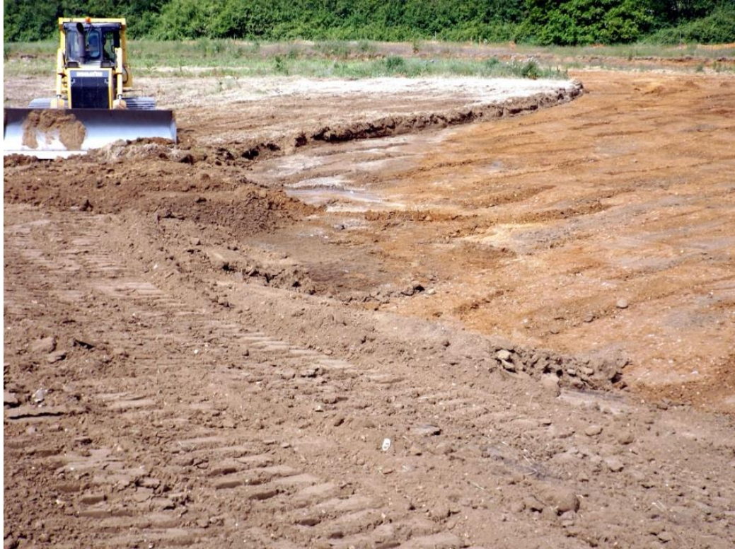
The northern edge of the former extraction pit with the D6 Dozer forming the bund, looking west Fig 11
