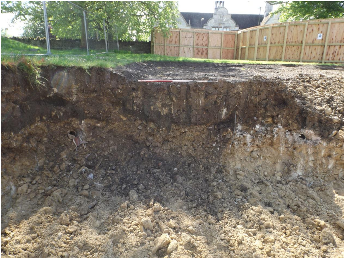
Section of the wall cutting for the Palmer building, looking south-west Fig 3
