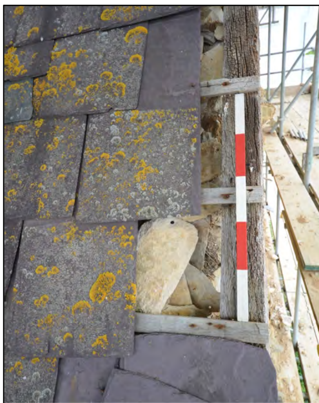
Detail of roof slatework at the south-east gable, showing phases of roof materials Fig 5
