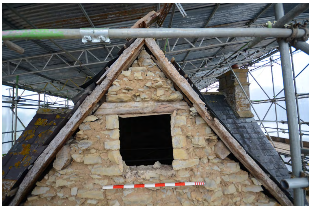
The upper portion of the external face of the south-east gable, looking west Fig 9
