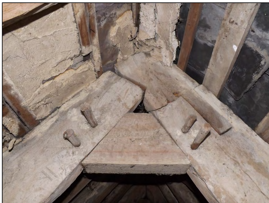
Detail of joinery at the upper portion of the cruck truss with a carpenter's mark visible at the lower left of the image Fig 33
