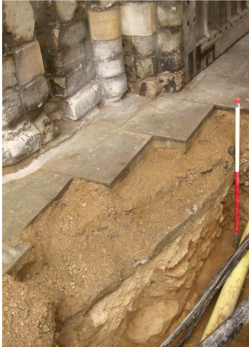
Gas trench at the Cathedral West Gate, showing stone foundations of the 12th to 14th centuries, looking north-east Fig 3.4
