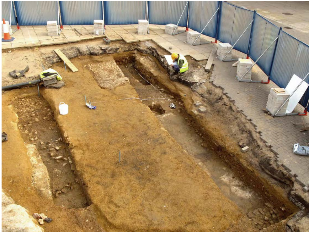
The fountain array area with the two deeper trenches containing walls and floors of Building 3, looking north-east Fig 3.16
