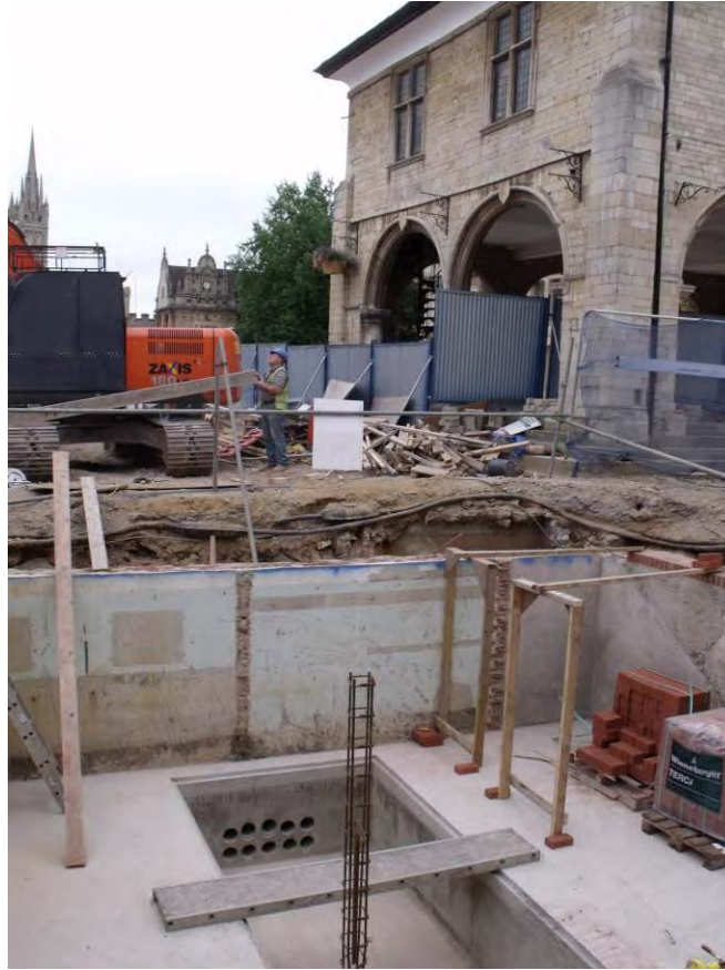
Underground toilets, during conversion into the electricity sub-station; the floor deepened to accommodate the transformer, looking south-east Fig A3.14
