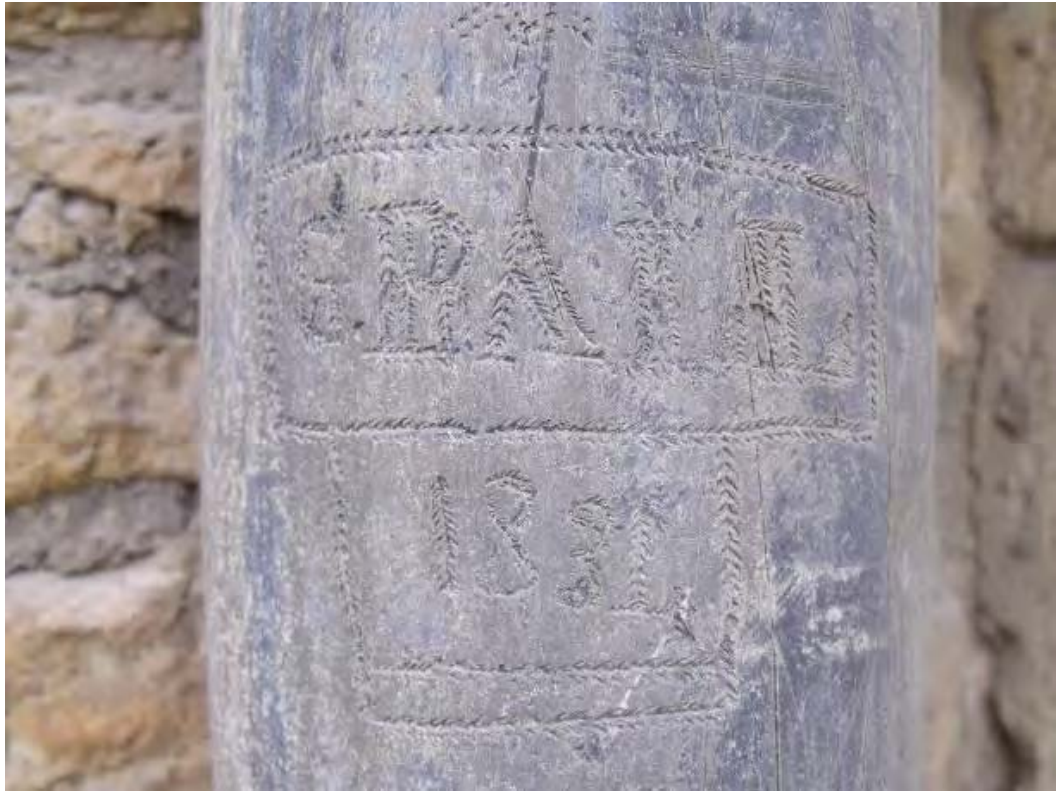
Graffiti on 19th-century lead piping on the church, with name Grail and a date of 1831 Fig A5.14
