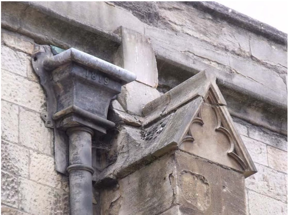
One of the 1819 lead rainwater chute outlets, located along the south side of the church, looking north-east
