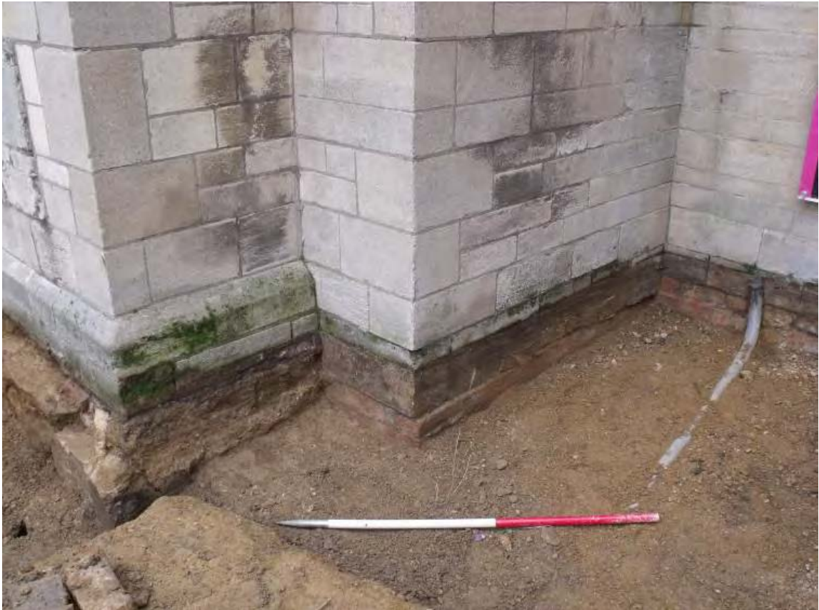
South turret of the 14th-century gateway, showing 1930s refurbishment, with brick and concrete foundations (1595), looking north-east Fig A1.14
