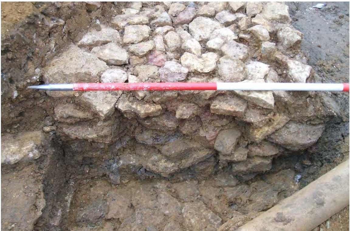
Section through building wall [1055], aligned east-west, in construction trench [1120], Trench 56 looking east Fig A2.16
