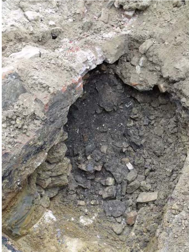
Brick cellar wall [1786] undermined by quarry cut [1785]; wall is supported on the natural gravels and clay, but also by a column of quarried limestone blocks (1787). Building 7, Cellar 3, Trench 55, looking north-east Fig A3.11
