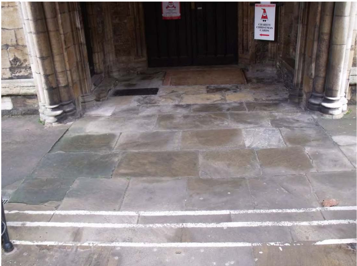
The steps from Church Street on to the flagstone surface, below the south church porch, looking north Fig A5.12
