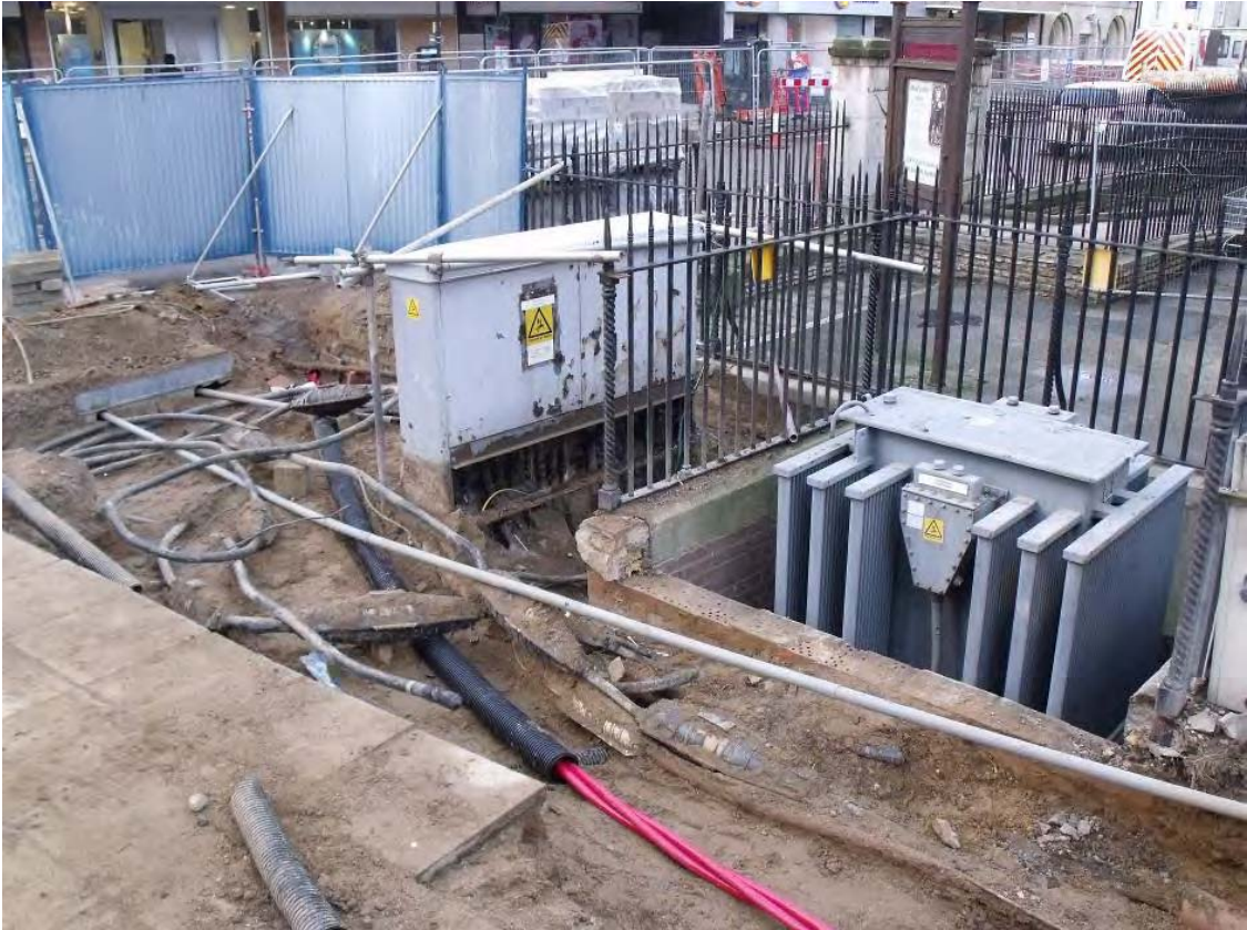
Sunken electricity transformer, before its relocation to the converted toilet block, looking south-west Fig A3.15
