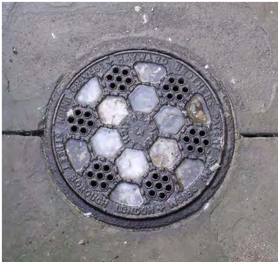
The 19th-century cast iron coal chute cover, located to the east side of the church Fig A5.17
