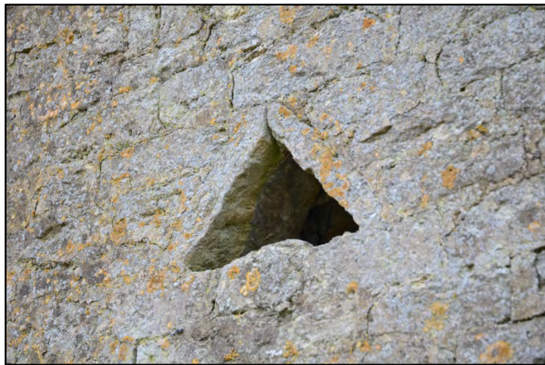
Detail of triangular vent on the east elevation of the north range Fig 12
