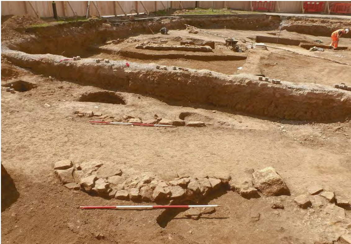
Remnants of a curving and a linear wall, looking west, towards the 12th-century building Fig 15
