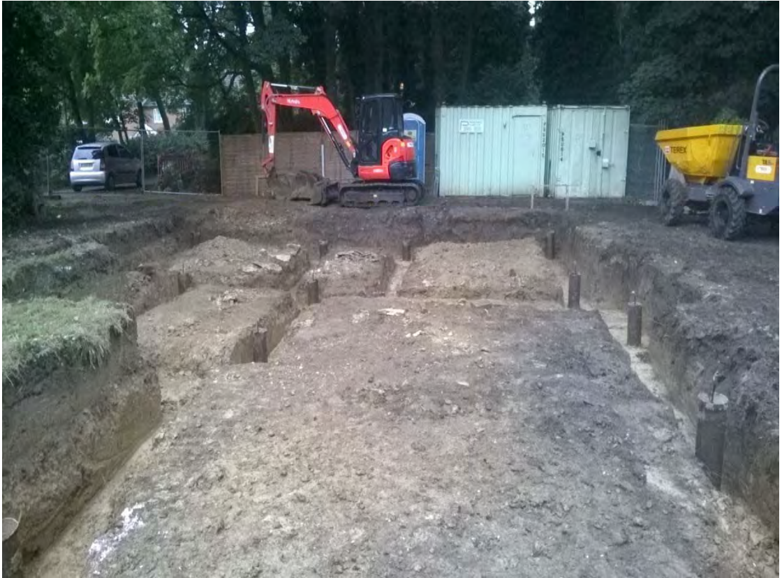
The area of the house and car-port after the soil strip, looking north Fig 6
