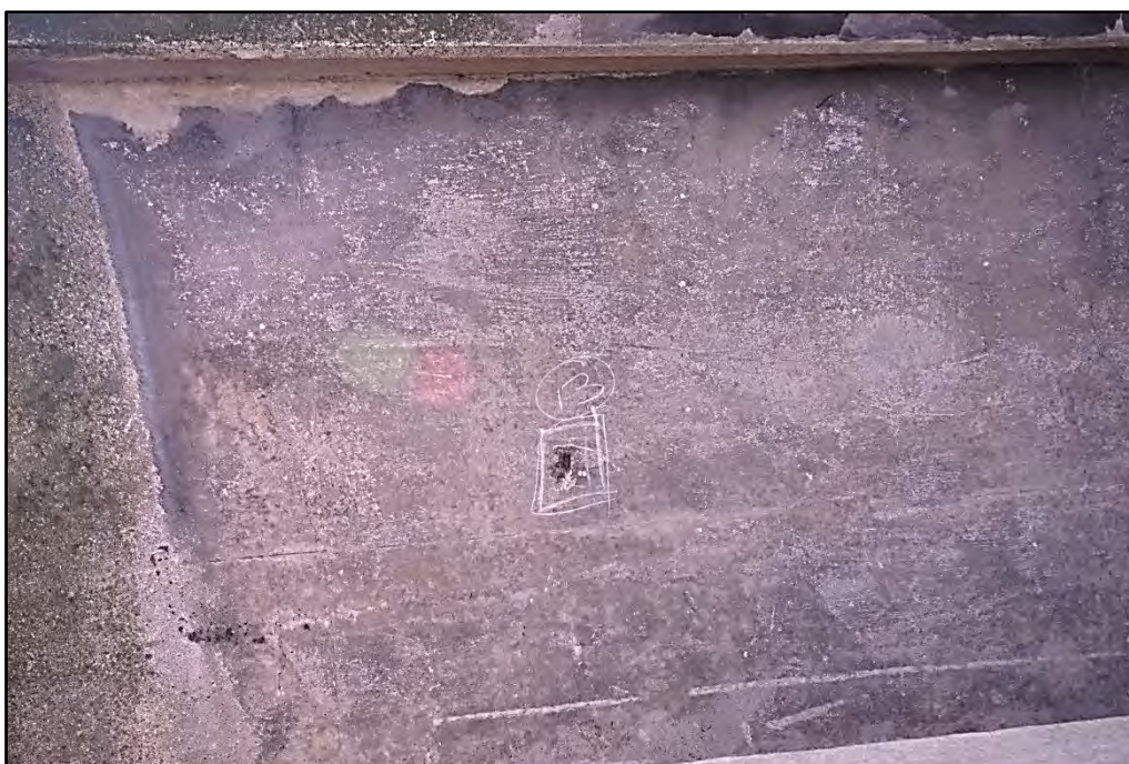
Blown concrete showing the steel reinforcement and scratches on west abutment wall Fig 52
