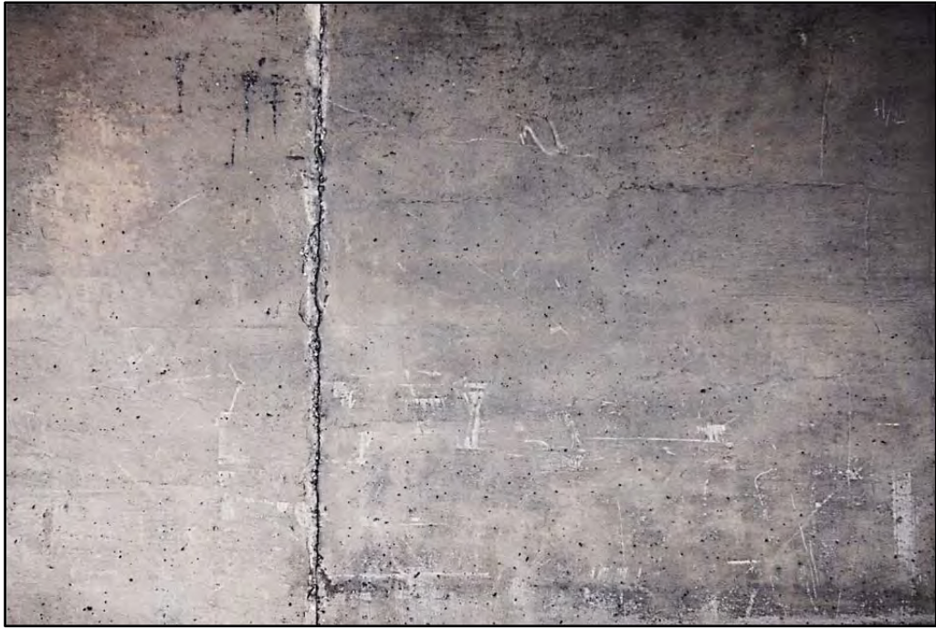
Wear and markings on the east abutment wall Fig 80
