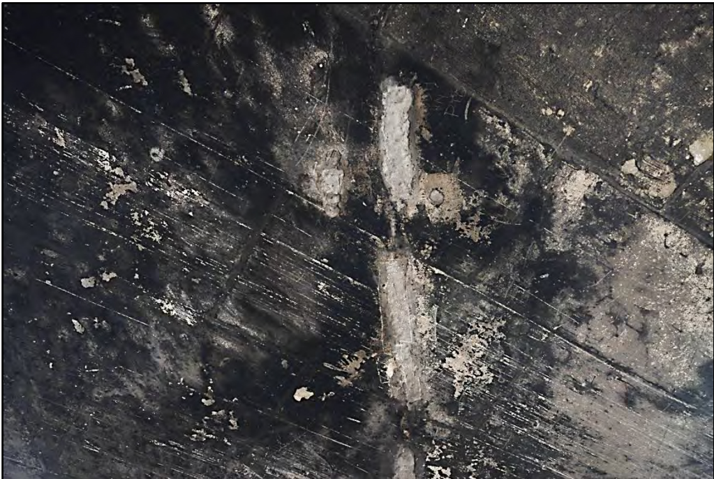
Scratches and damage on the underside of deck, northbound Fig 50
