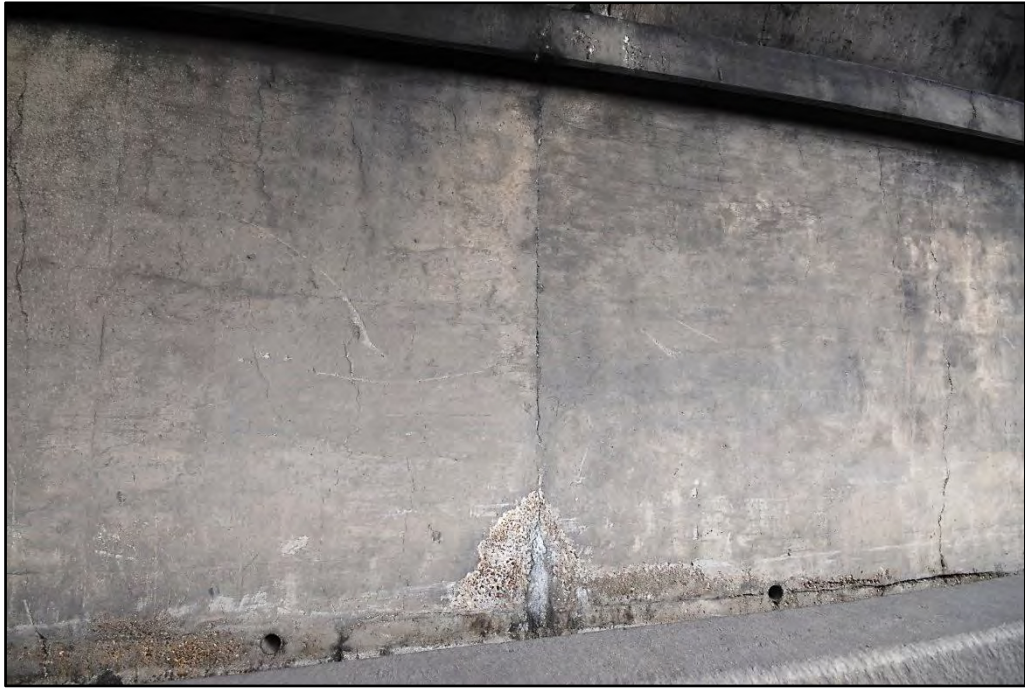
Scratches, cracks and water seepage on east abutment wall Fig 53
