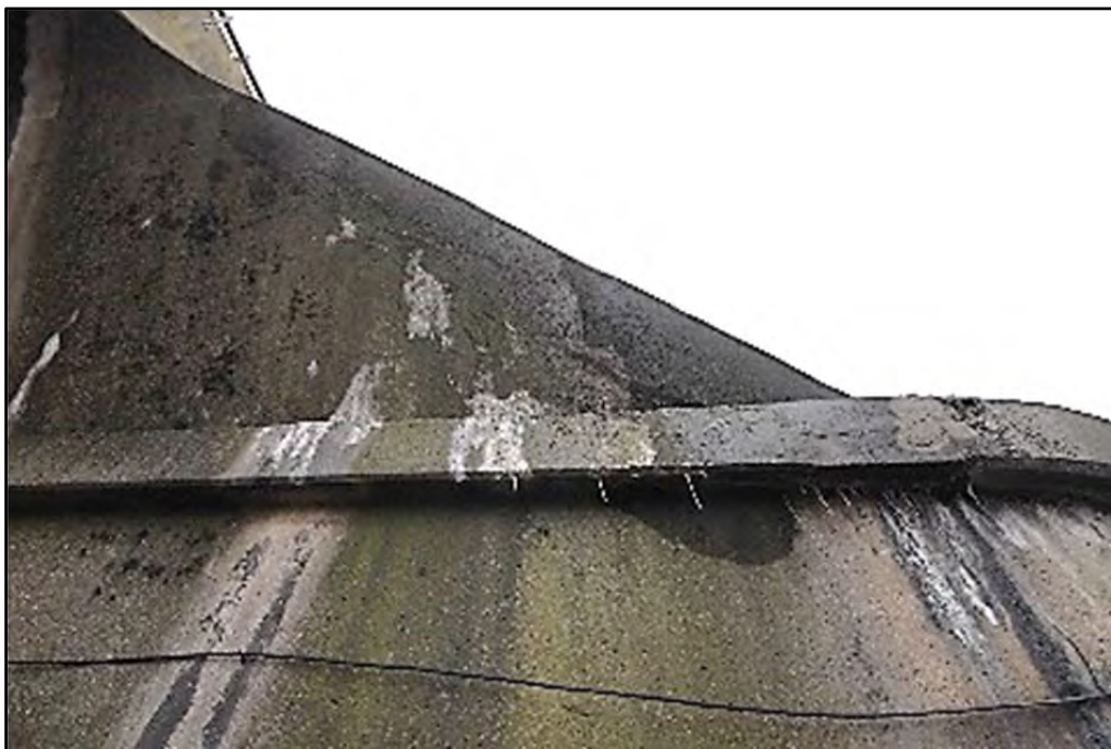
Water issues on north-west scroll Fig 77
