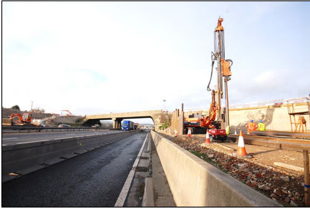
Construction of the new bridge by the Chalton Bridge, looking north-west Fig 13
