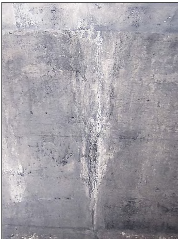
Decay of the concrete Fig 79
