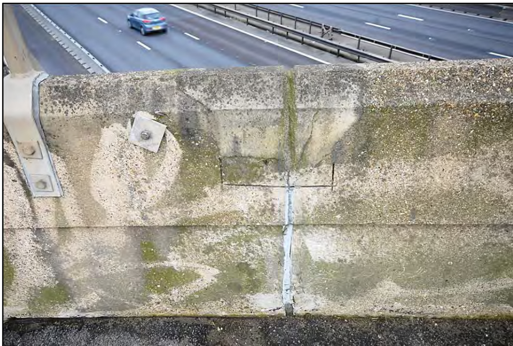
Damage and repair on north parapet Fig 48
