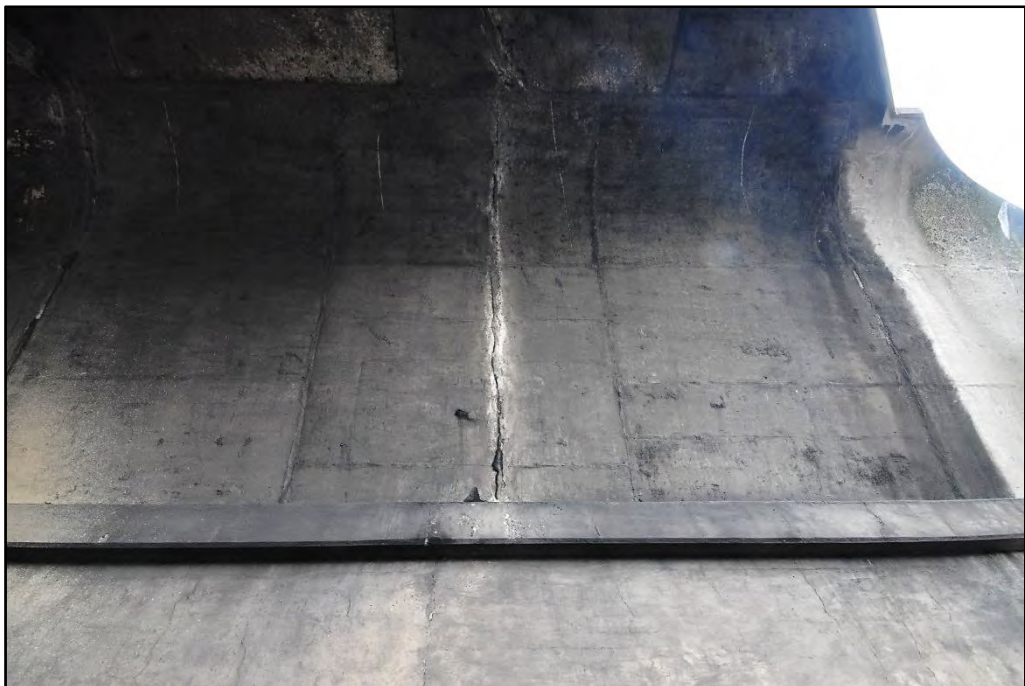
Crack with water deposit Fig 54
