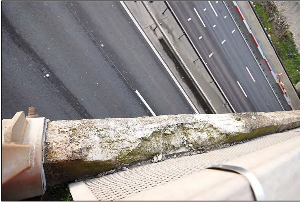
Damage on south parapet Fig 47
