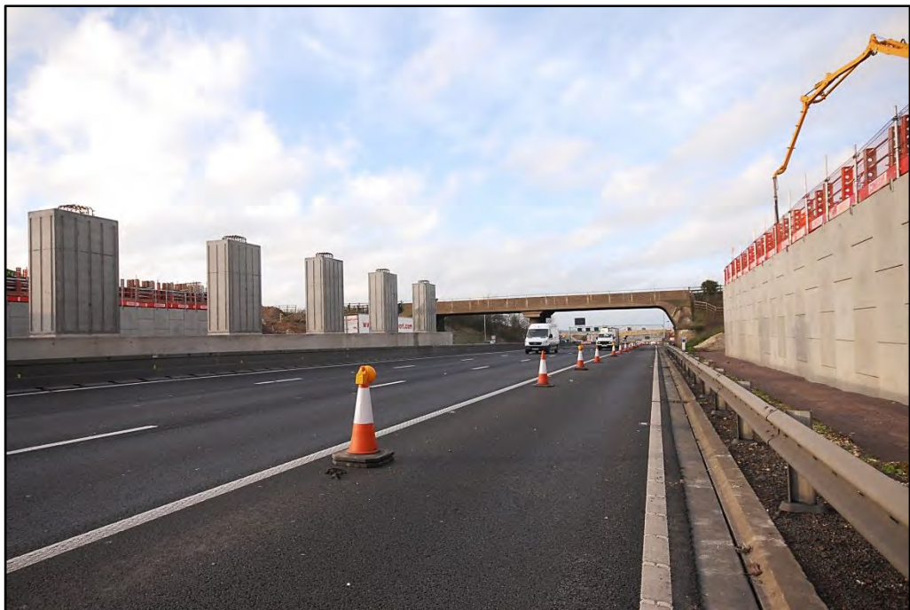
Construction of the new bridge by the Houghton Regis Bridge, looking north-west Fig 14
