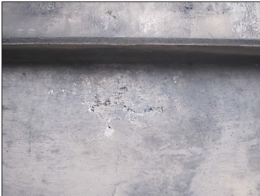
Pitting on the structure Fig 78
