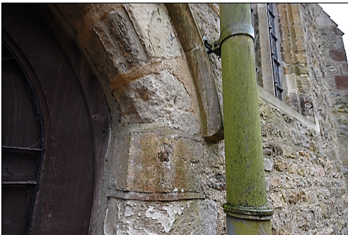
The replaced jamb stone under the spring line with an iron bolt Fig 14
