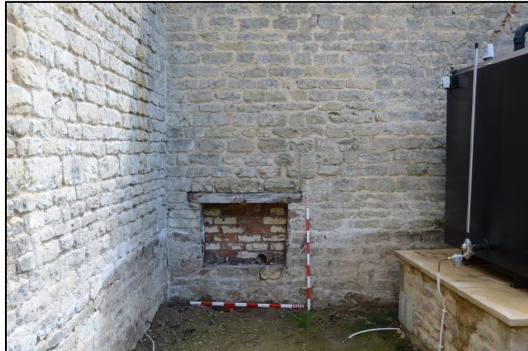
Blocked window to Brewhouse cellar Fig 71
