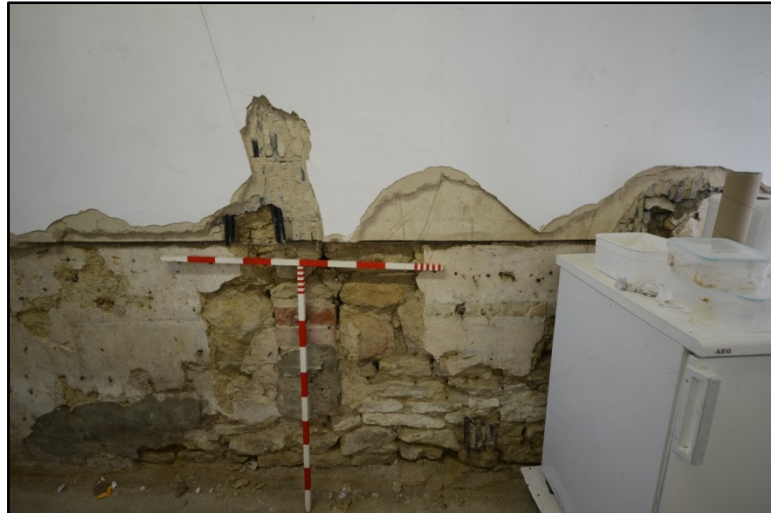
Detail of construction and alteration to the east wall of Room 2 Fig 173
