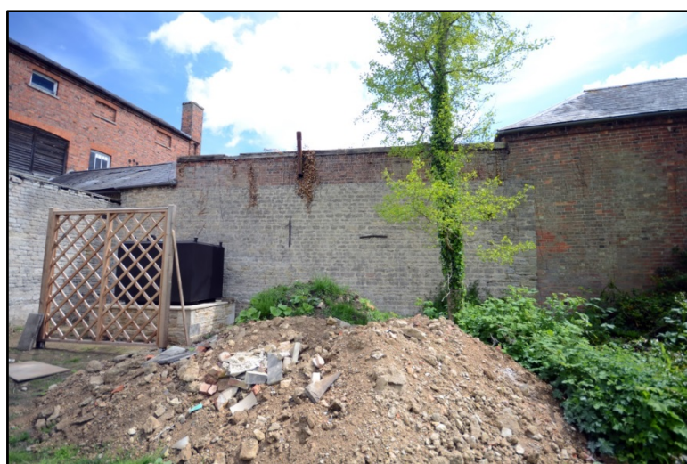
The west elevation of the Tack Room, showing brick over earlier stone wall, and join with the Stables Fig 80
