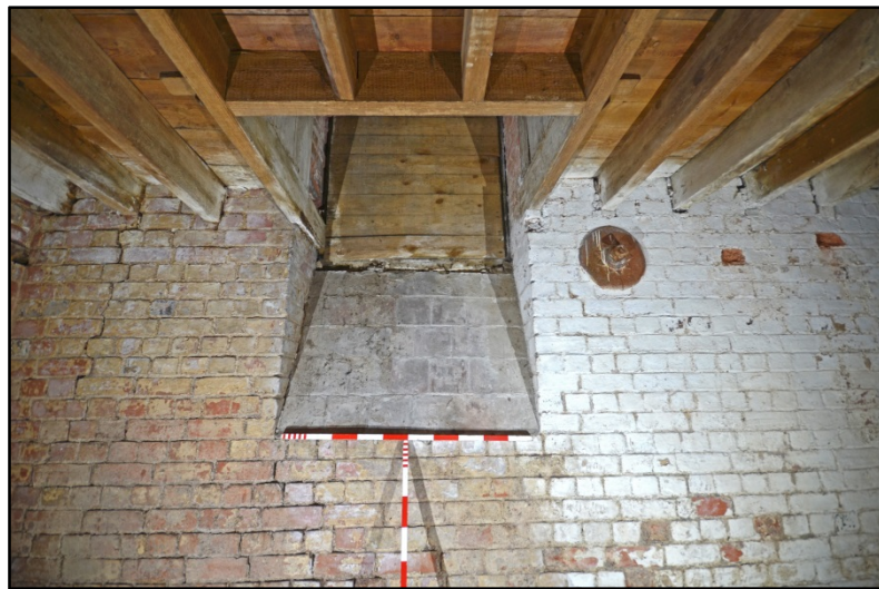
Hatch to drying room Fig 133
