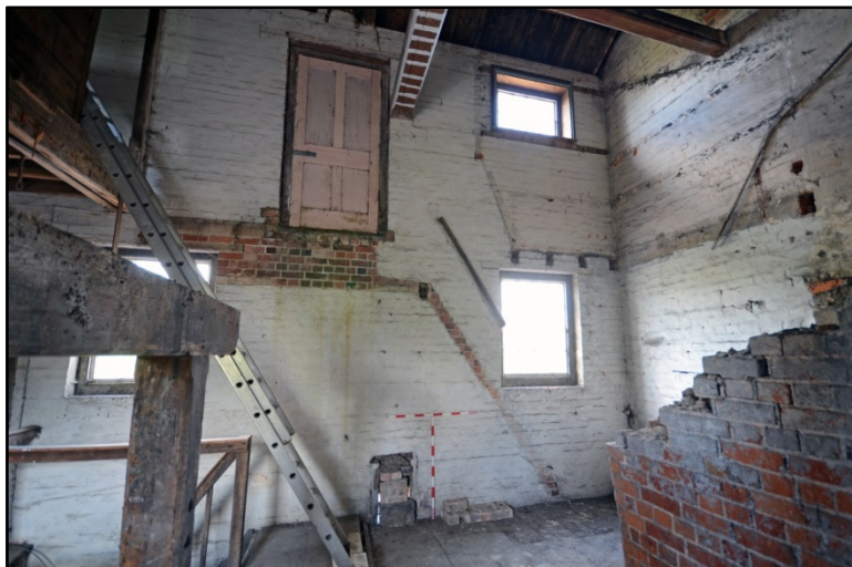
The north-east corner of the first floor following removal of the office level Fig 46
