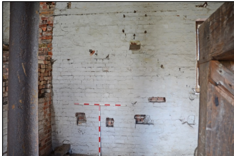
Empty beam slots and bolts for former equipment Fig 45
