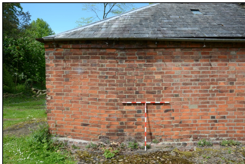
Stable 4, detail of subsidence in the brickwork Fig 88
