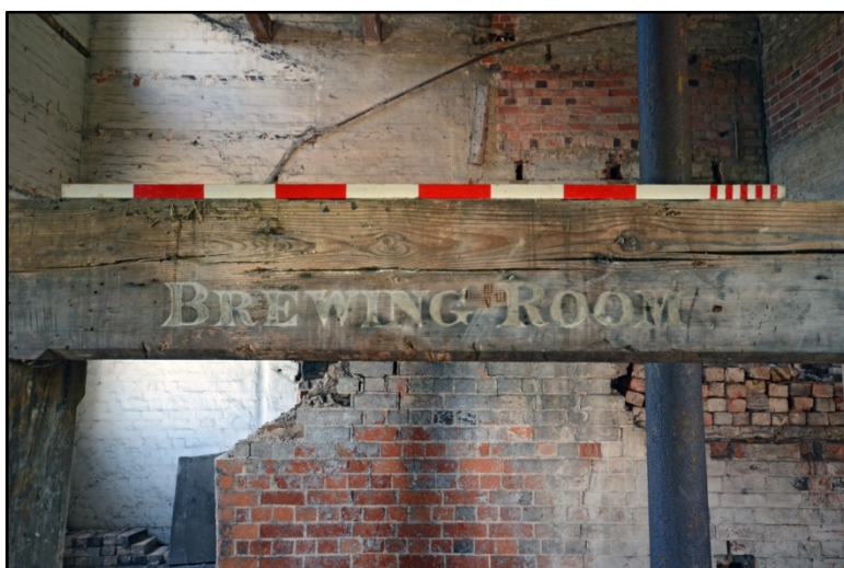
Painted notation on supporting beam Fig 40
