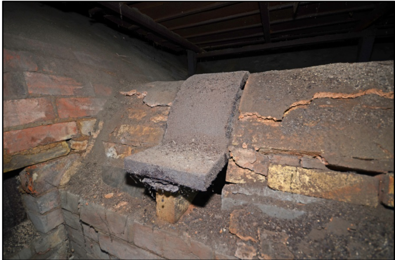
Detail of cast iron collar and remnant plaster on the kiln Fig 146
