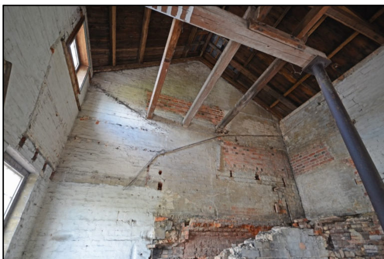
The east elevation with empty joist slots and scars of former water tanks Fig 47
