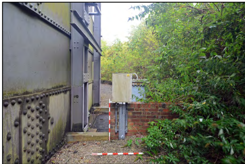
Sump with sump pump controls, looking south Fig 22
