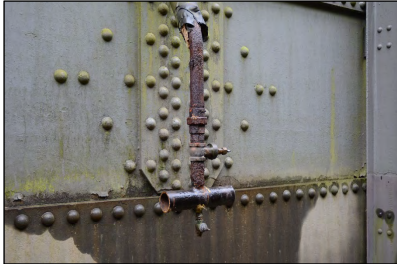
Remnant anti-freeze pipe Fig 21
