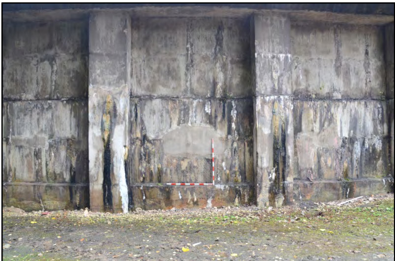
Detail of surface damage and repairs Fig 61
