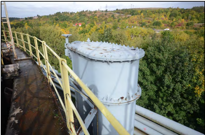
The top of the inlet / outlet pipes Fig 19
