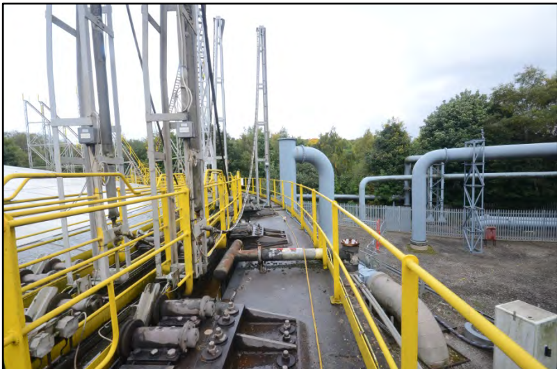
Anti-freeze pipes and supports Fig 74
