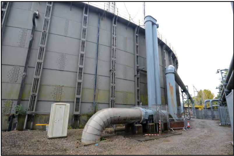
Inlet / outlet pipes and kiosk Fig 16
