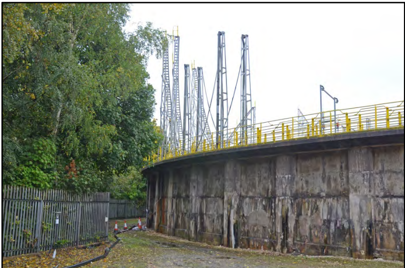
The east side of the tank, also showing anti-freeze supports Fig 63
