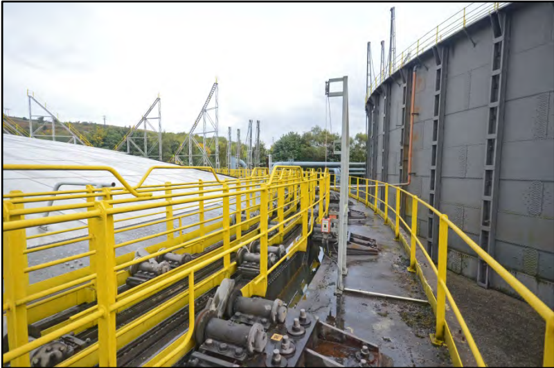
Operational equipment Fig 76
