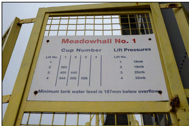
Signage on stair gate Fig 32
