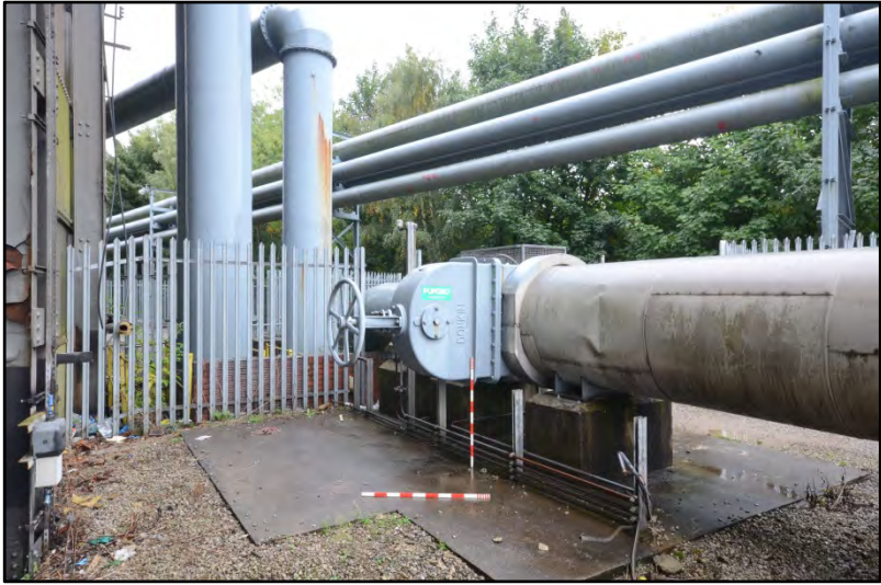
Detail of flow valves Fig 17
