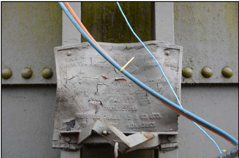
Damaged commemorative plaque Fig 28
