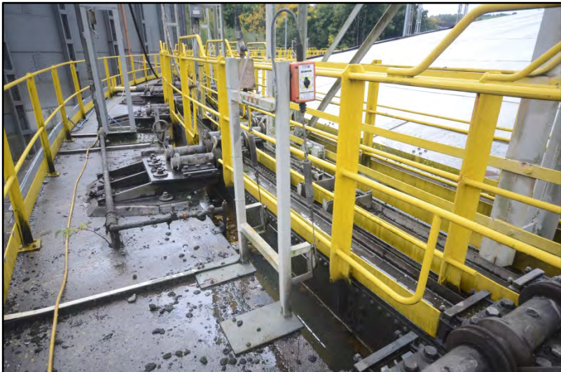
Operational equipment Fig 73
