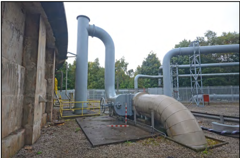
Inlet / outlet pipes and flow valves, looking north-east Fig 54
