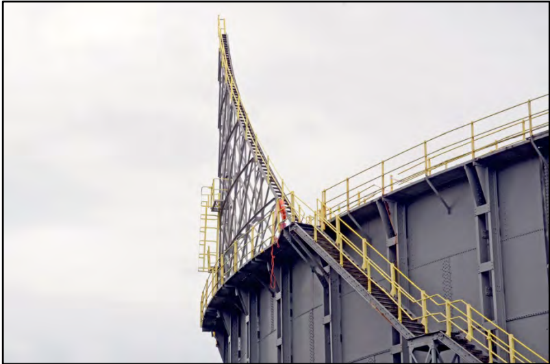
The upper part of the base-tank stair, also showing lift-tank stair Fig 33
