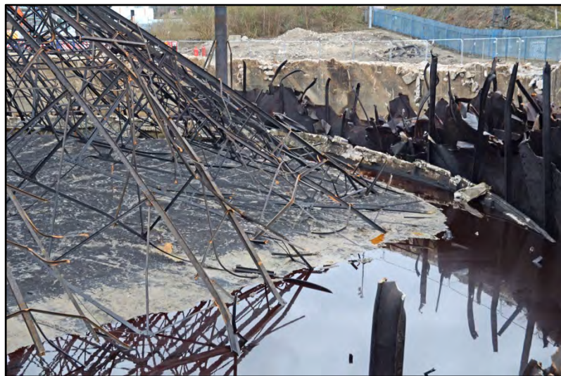
The inner concrete ring and subsidence of the dumping Fig 87
