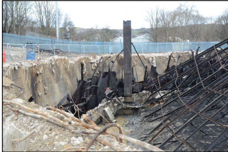
The dumping edge and pipe leading to the former western sump Fig 86
