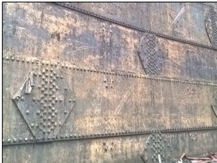
The inner face of the base-tank Fig 51
