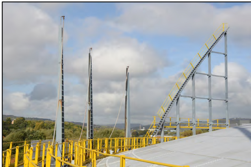
Anti-freeze pipe supports, looking south-west Fig 39
