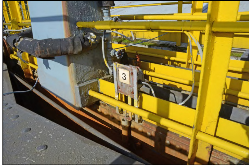
Detail of the anti-freeze pipes and valves leading to the supports Fig 40
