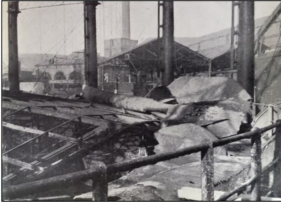
Bomb damage to No.4 Holder, with No.5 holder in background (Hird 1944) Fig 4
