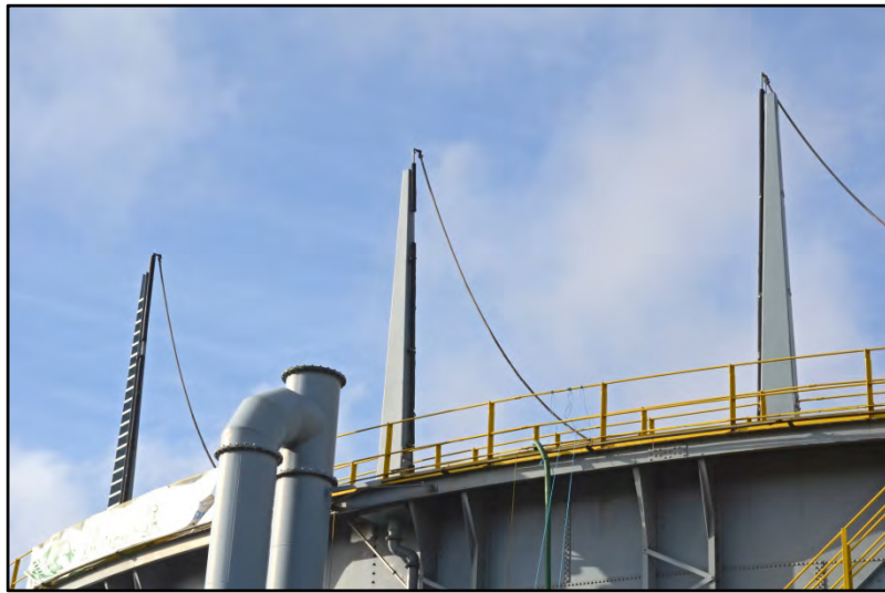
Anti-freeze pipe supports Fig 38
