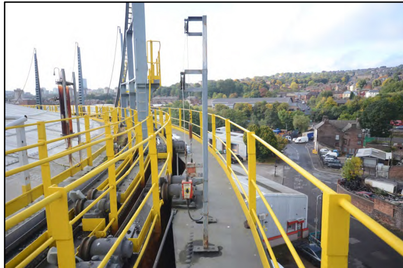
Operational equipment Fig 43
