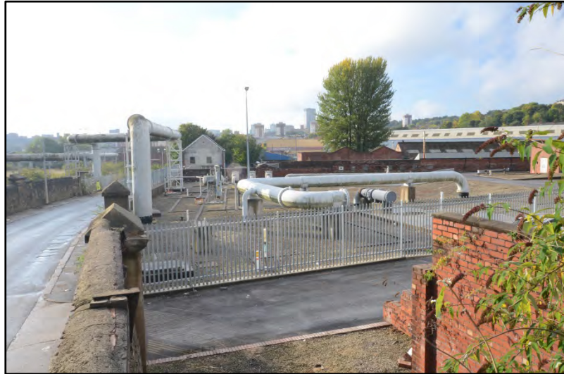
The National Grid compound, looking south Fig 12
