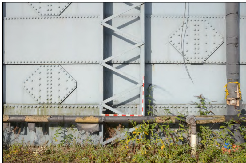
Detail of base-tank column, also showing lagged anti-freeze pipes Fig 20
