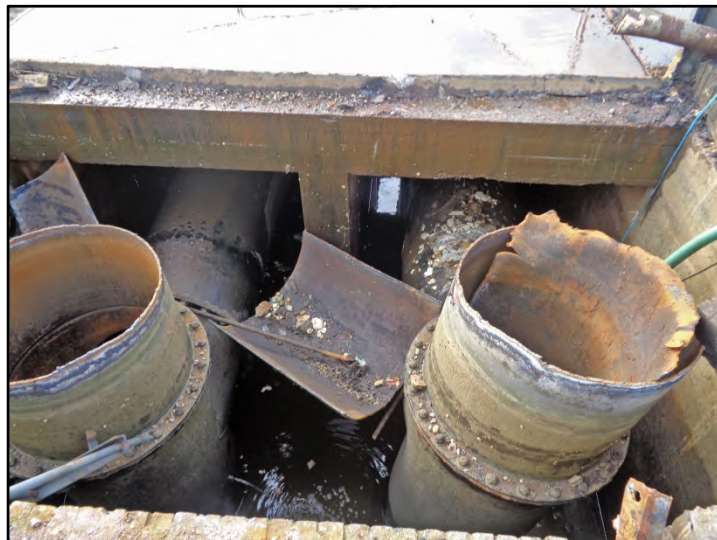
The inlet / outlet pipes and pipe pit Fig 55
