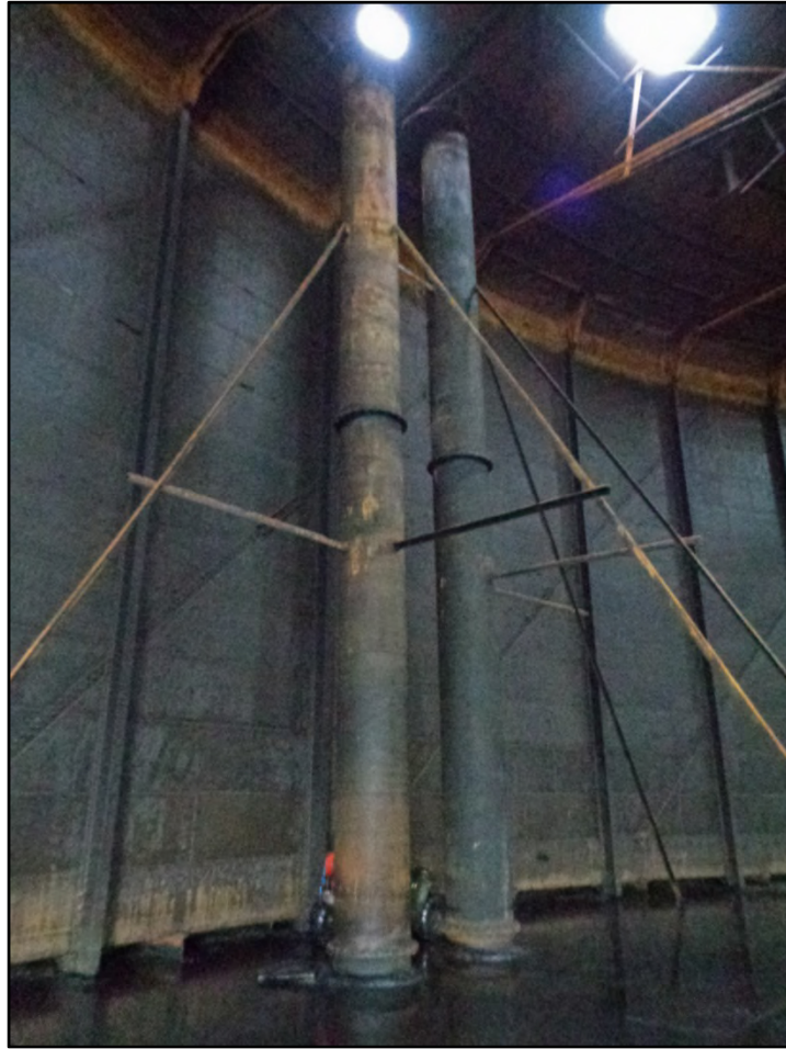
The inner inlet / outlet pipes Fig 54
