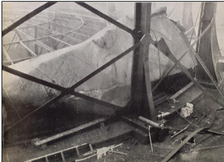
Bomb damaged gasholder (Hird 1944) Fig 5
