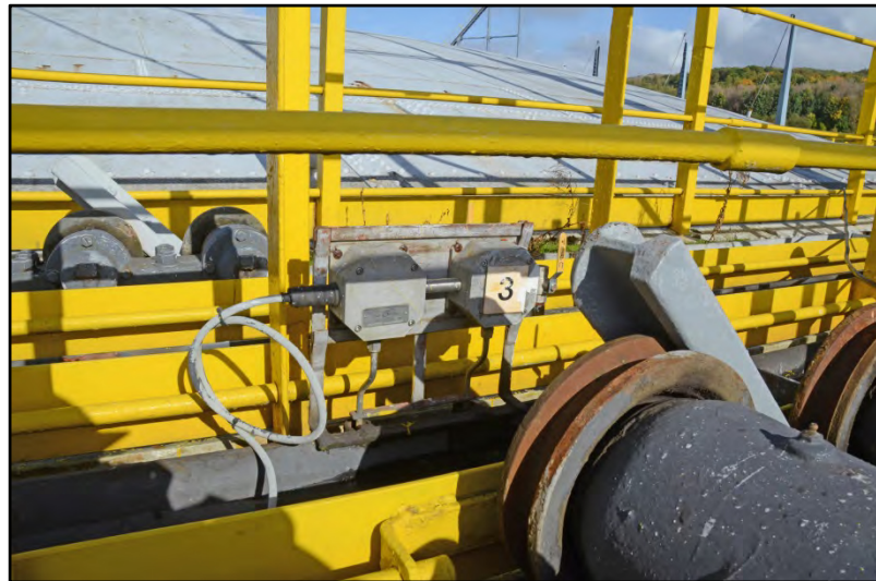
Detail of electrical fittings Fig 41
