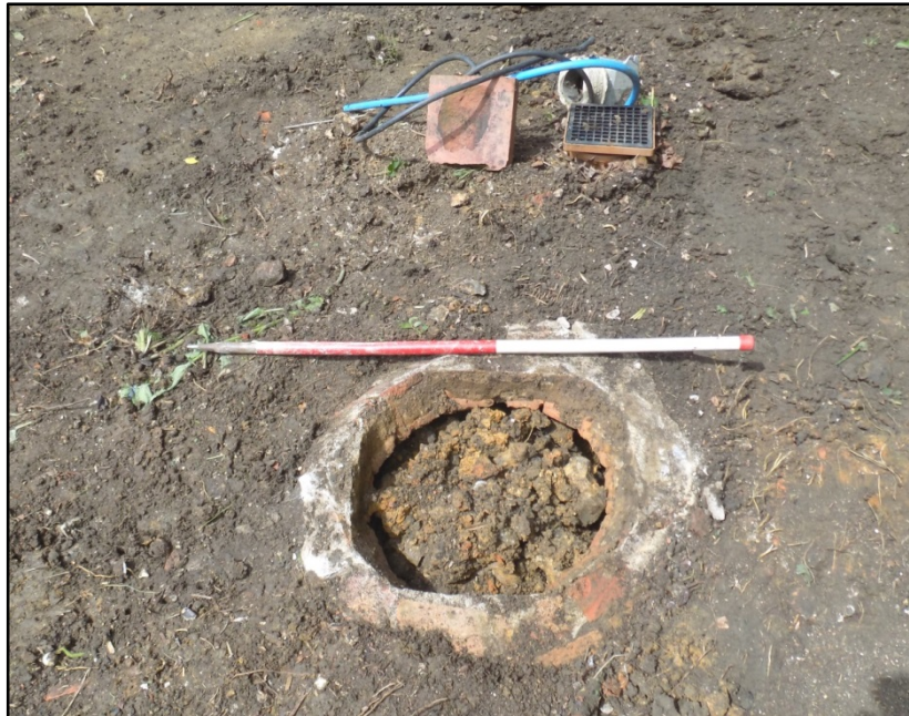
The plugged septic tank [4] inspection chamber and vent pipe, looking west Fig 5
