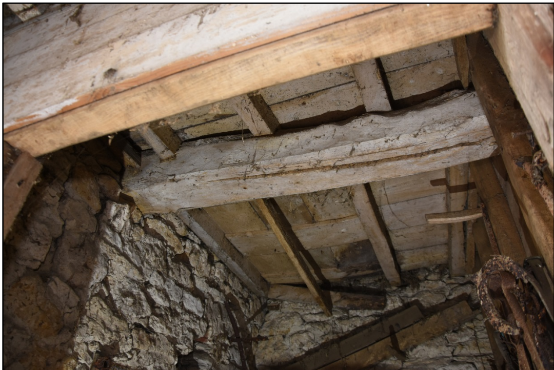
Detail of the beam and remaining floor as seen within the store room Fig 25
