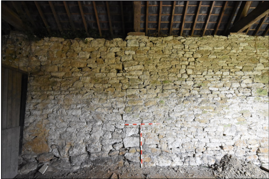
The vertical joint on the inner face of the western wall Fig 30
