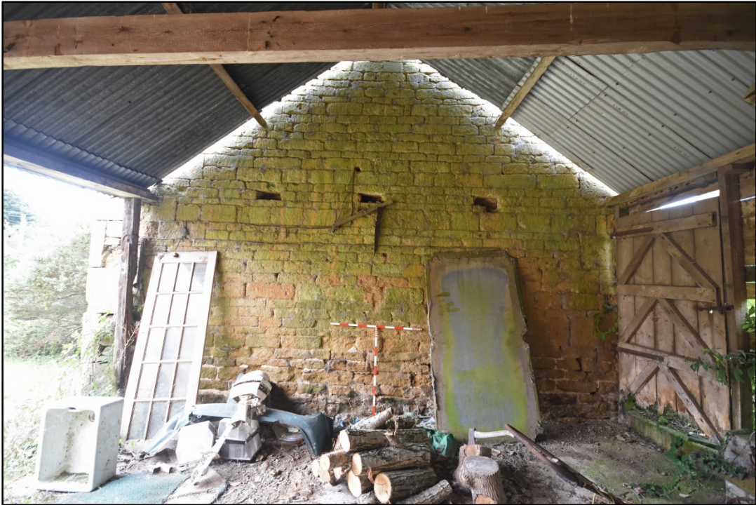
The north elevation of the barn, viewed from the extension, looking south-west Fig 38
