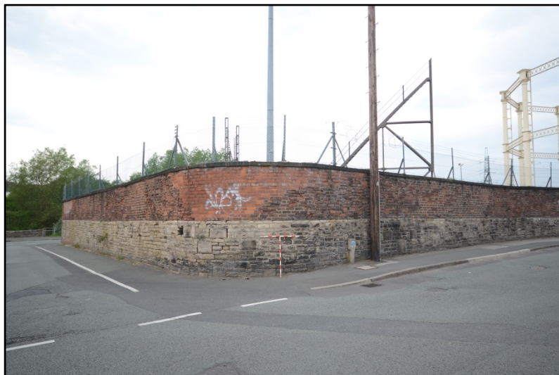
The site boundary, seen from the junction of Garden Street and Black Lane Fig 13
