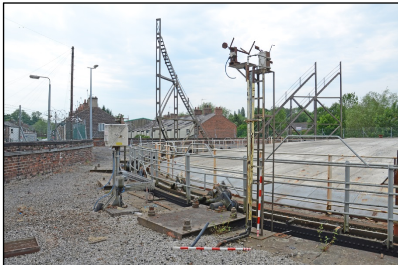
Telemetry and electrical fittings at the north-east side of the gasholder Fig 23
