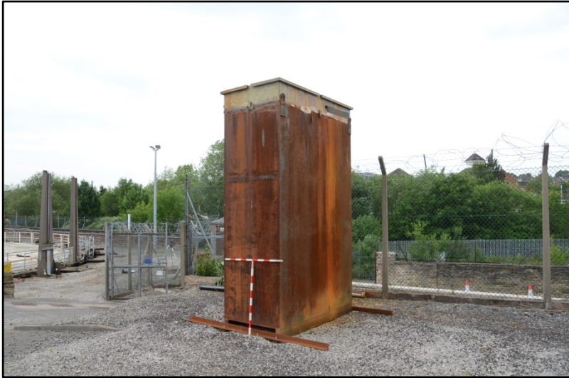
Methane sparge unit adjacent to Gasholder 2 Fig 60
