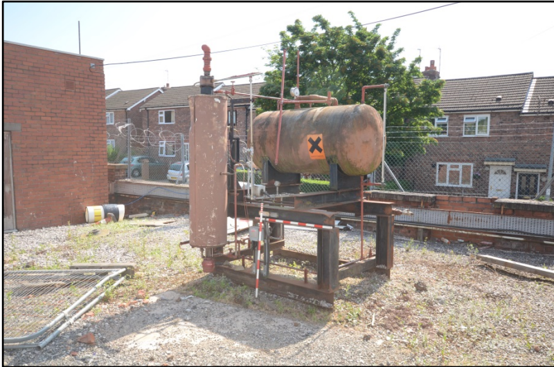
Propane tank adjacent to the Governor House Fig 58
