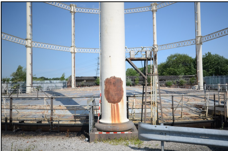
Column base, showing scar of removed plaque Fig 32
