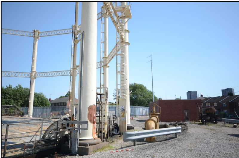
View of siphon pit and ladder at the south-east side of the gasholder Fig 40
