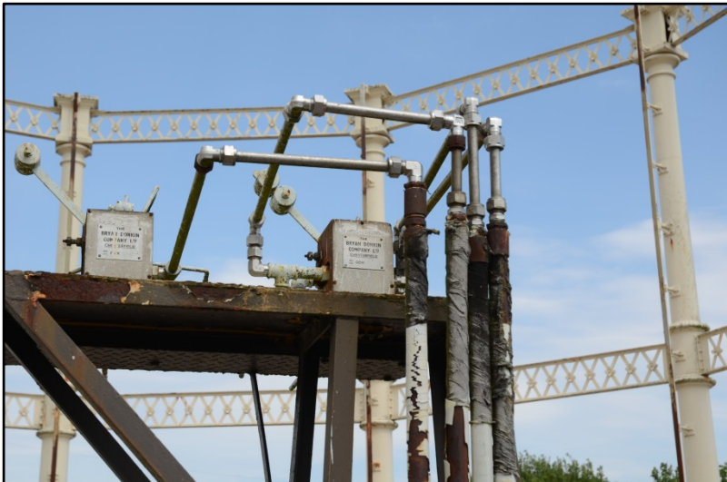
Detail of anti-freeze pipes and controls Fig 45
