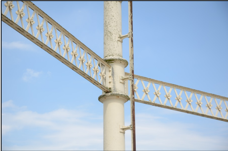
Detail of first tier junction box, with roller guide Fig 37
