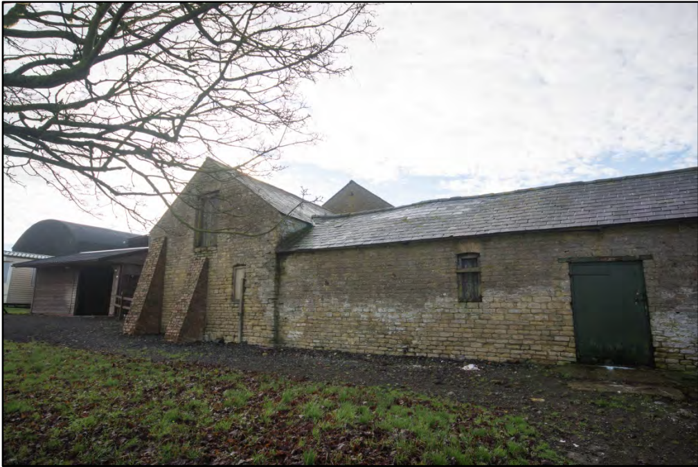
The north elevation of the Stable range and the eastern range Fig 25
