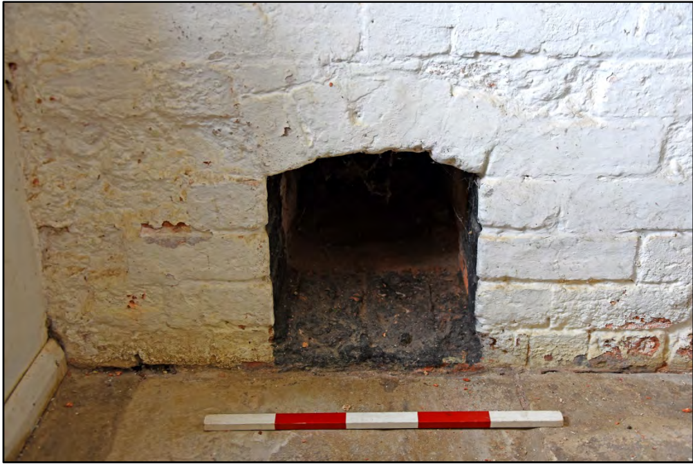
The flue below the oven Fig 18
