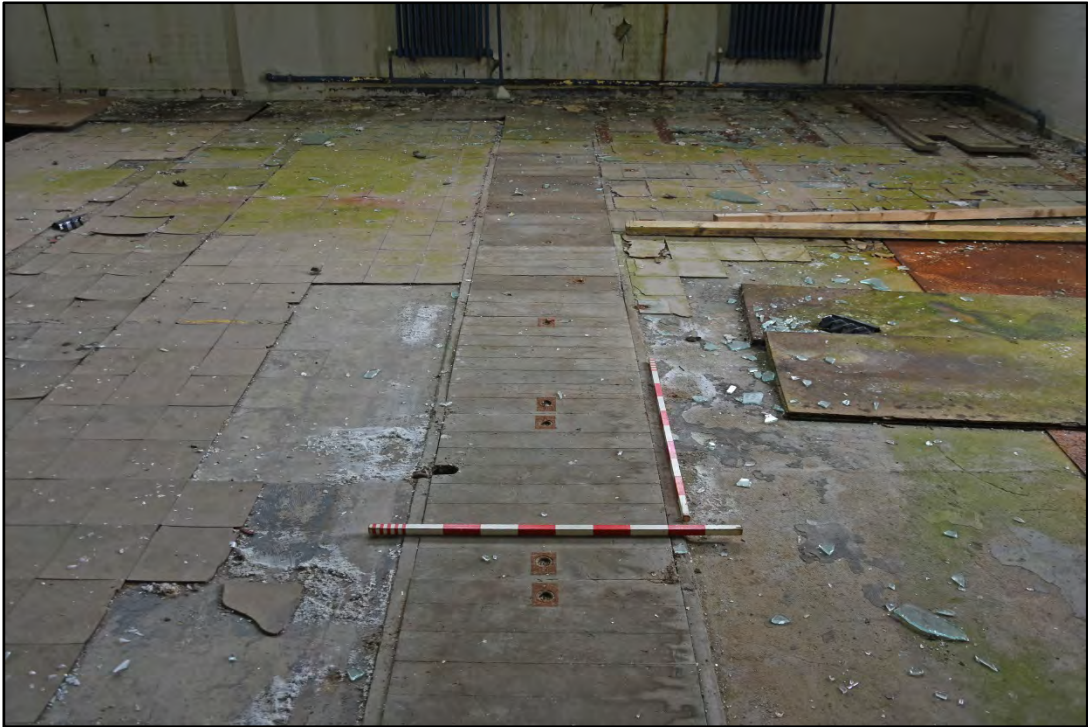
The covered cable and pipe trenches Fig 45
