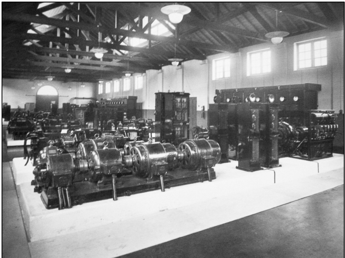
View of the Machine Room, showing Motor Generator sets, dated 1934 (E8911) Fig 12
