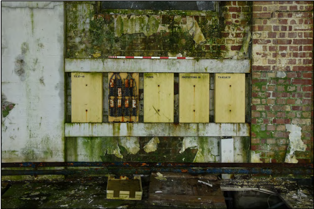
Detail of electrical boxes Fig 59
