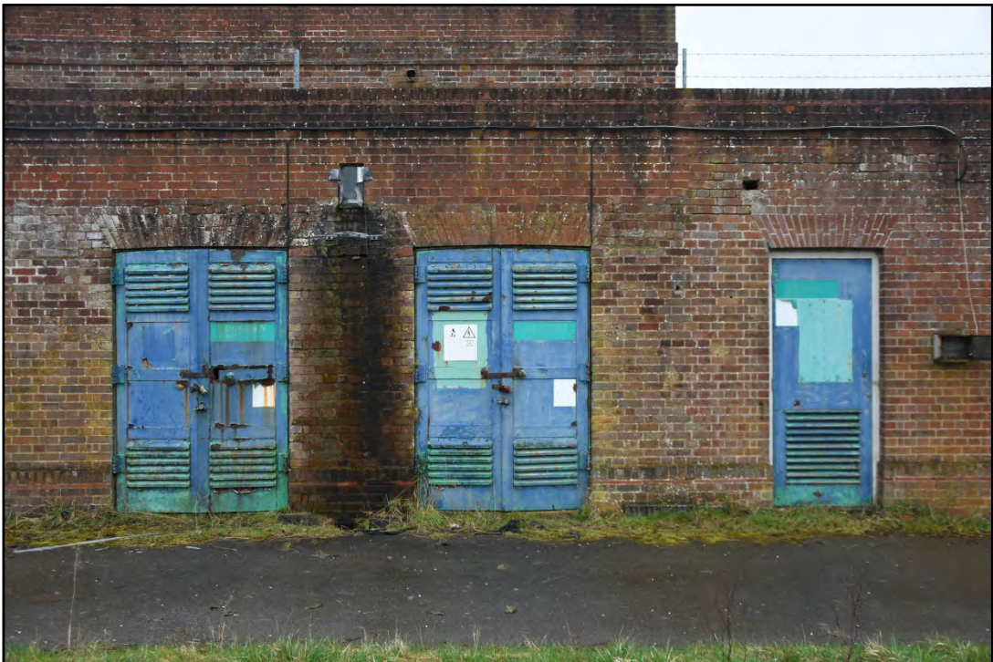
Doors to transformer rooms and switch room. Note change of brickwork between. Fig 18
