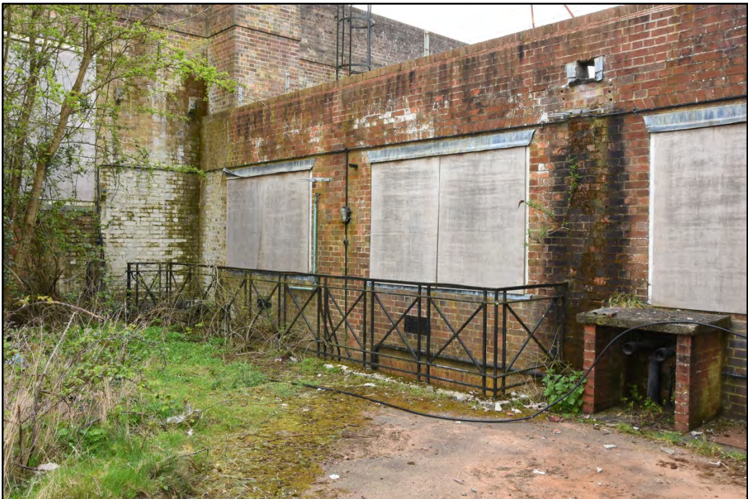
Railings and stair to the basement. Note fuel pipes adjacent to railings Fig 24
