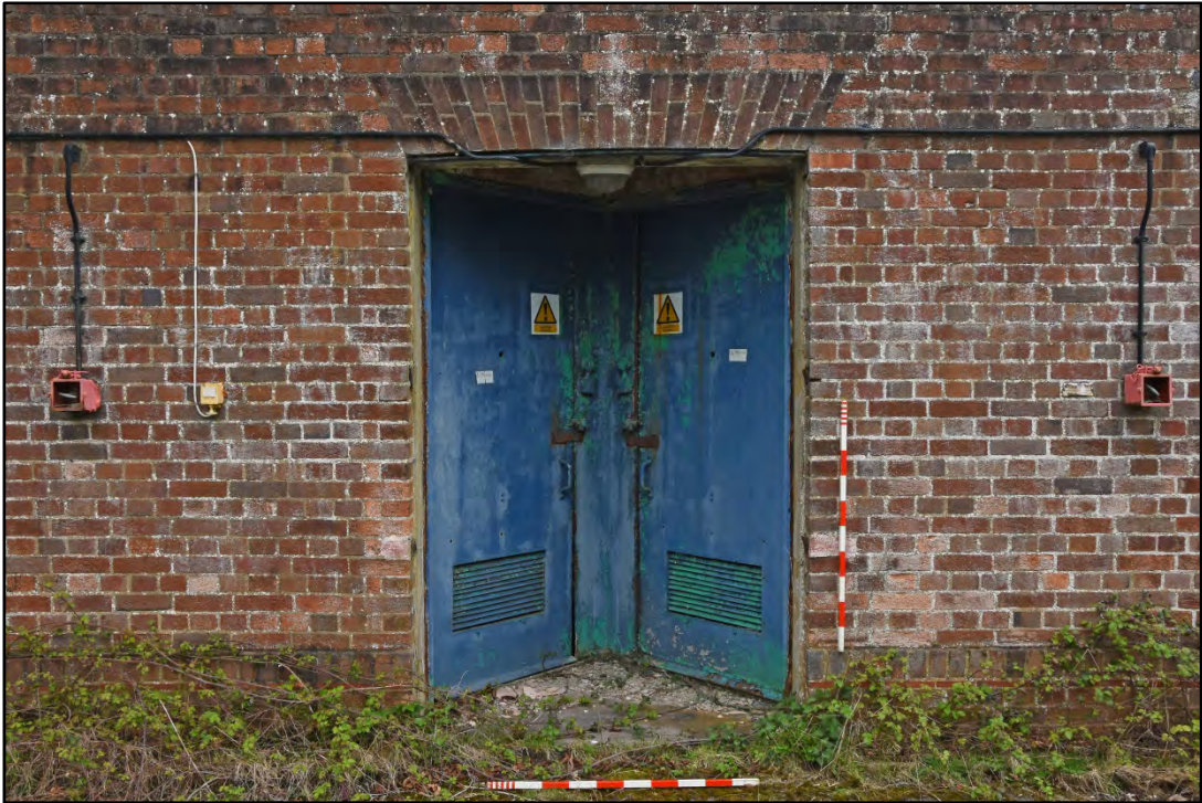
Entrance to transformer rooms showing the double-door arrangement Fig 29
