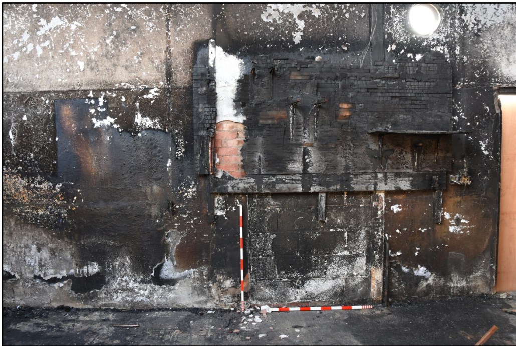
Breeze block and brick blocking of former door in the south elevation Fig 28
