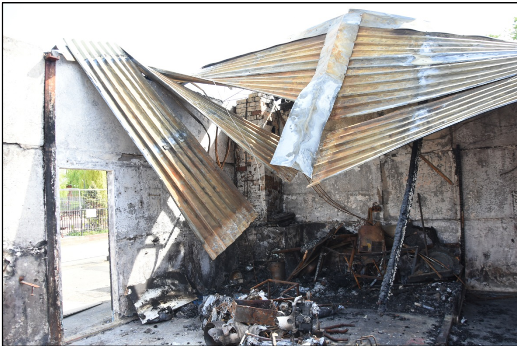
The north-east area of the boathouse, with chimney stack in the corner Fig 18
