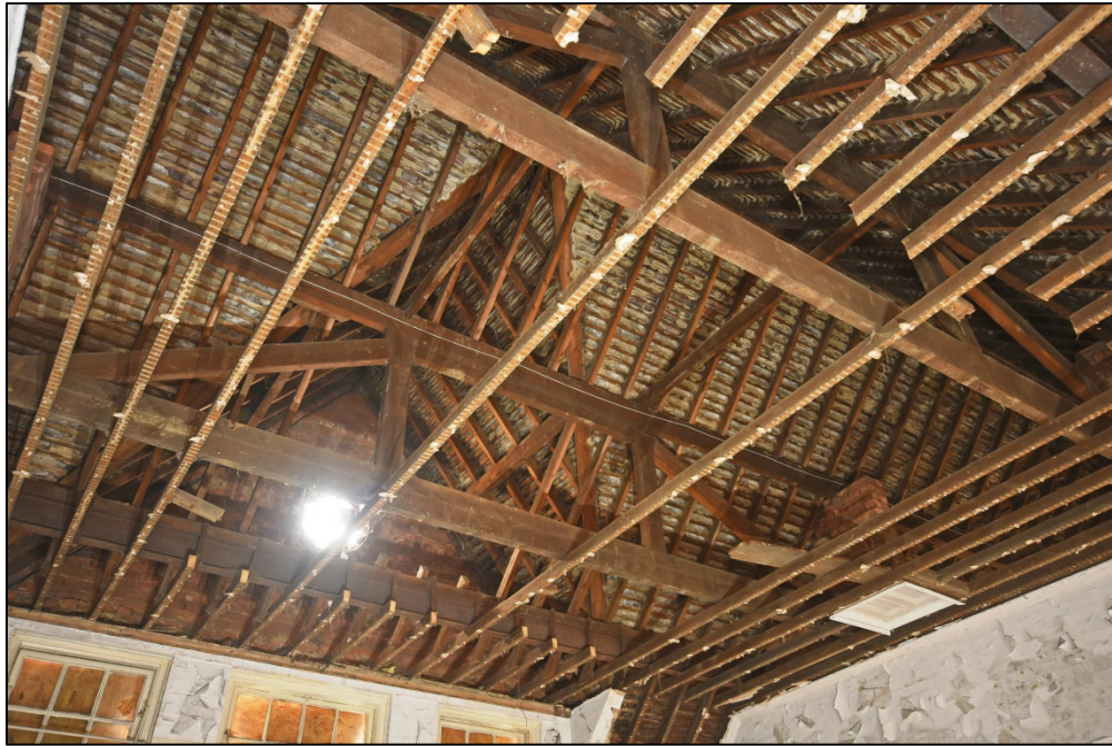
The roof over classroom 9, showing gable arrangement and queen post purlin supports Fig 94
