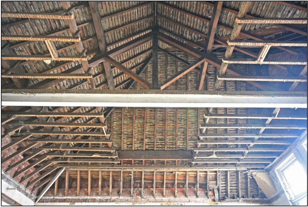
The roof over classroom 7, showing the hip, and the king post truss carried on an RSJ Fig 92
