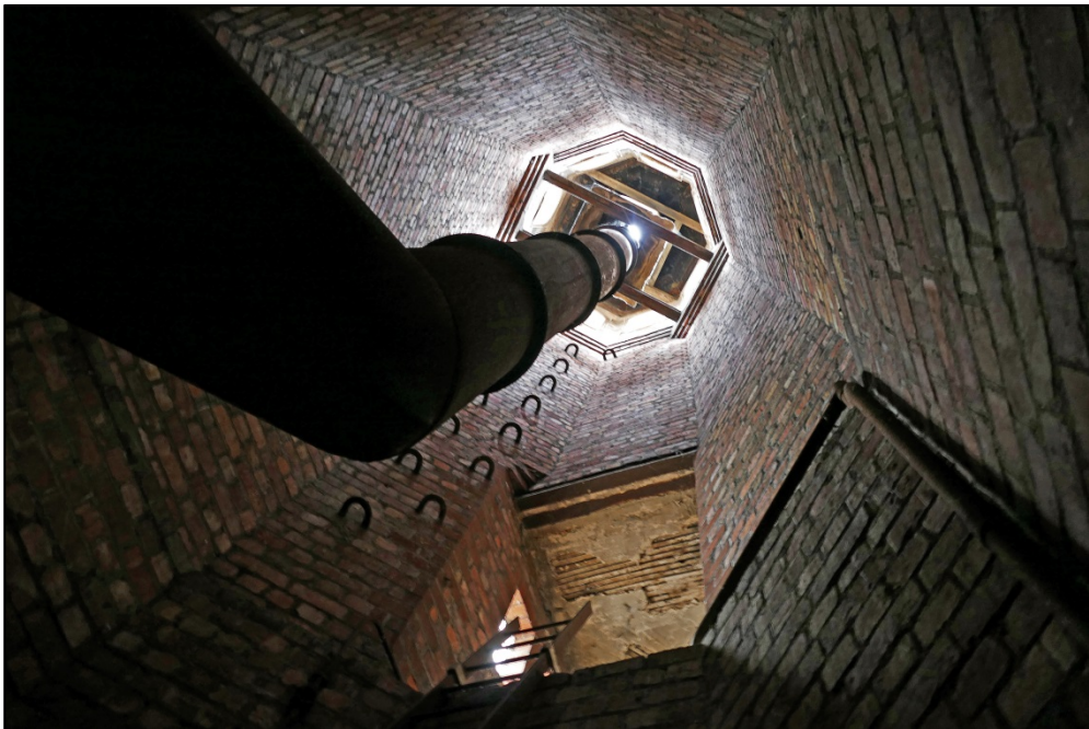
The interior of the tower, also showing entrance to hall roof access Fig 37
