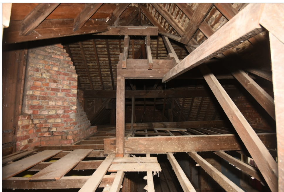
The roof over the first floor rooms, looking north, with tower base to the left Fig 52
