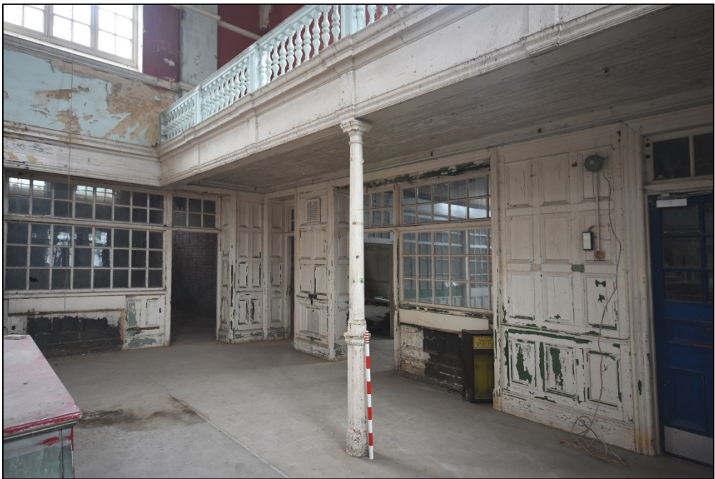
The mezzanine balcony with supporting column at the west of the hall Fig 59
