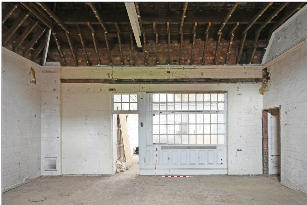
Classroom 10, looking south, note vent in corner, and RSJ supporting the roof truss Fig 95
