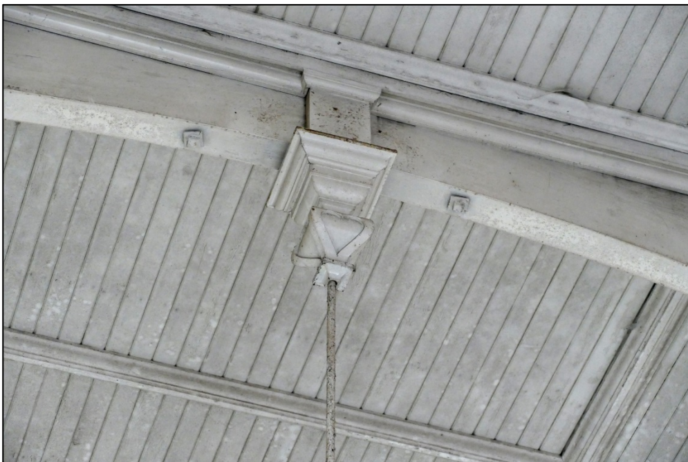
Detail of truss base / ceiling apex, with truss rod and decorative drop finial Fig 67
