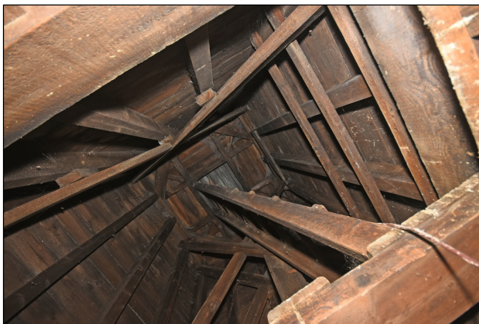
The bellcote, looking up at the trapdoor from the base stair Fig 32
