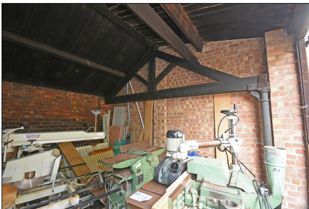
The central shed, showing defunct roof structure Fig 113
