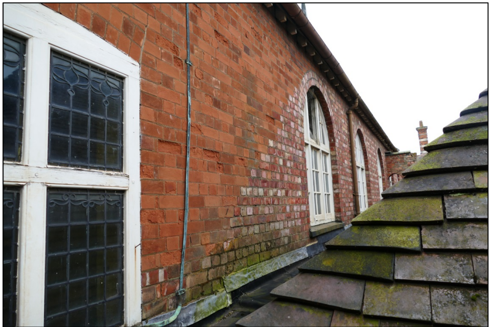
External view of the southern clerestory windows; note change of brick type Fig 61
