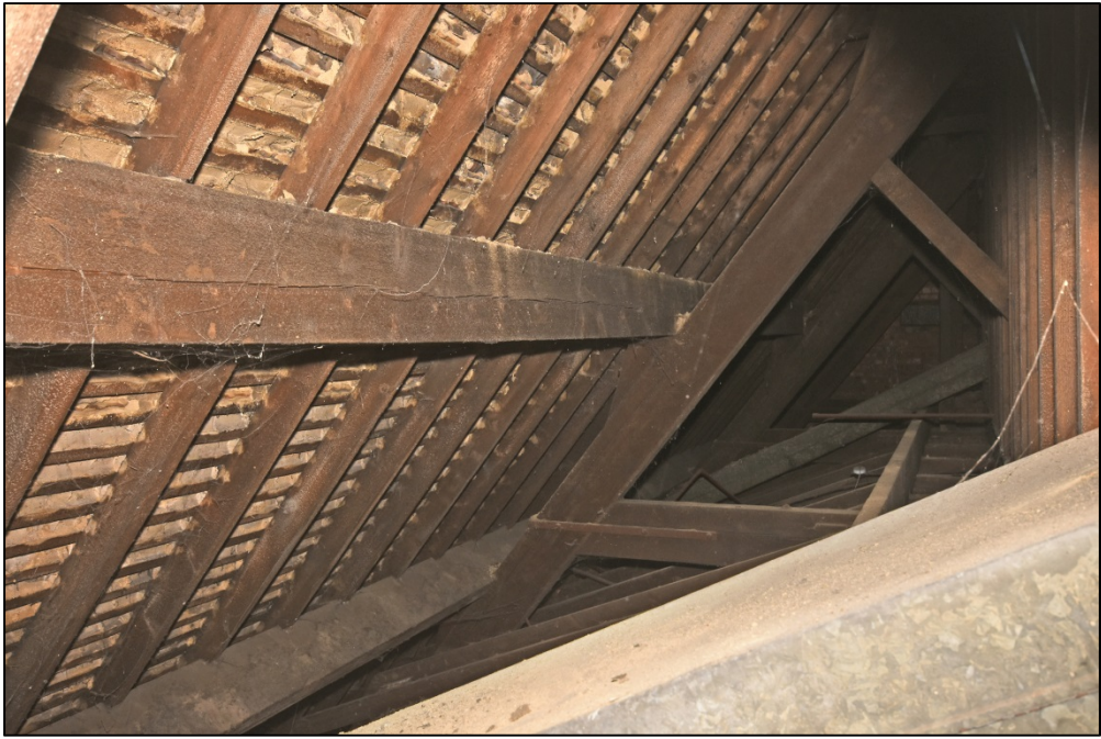
The roof structure of the hall, looking west along the side of the roof walkway Fig 68
