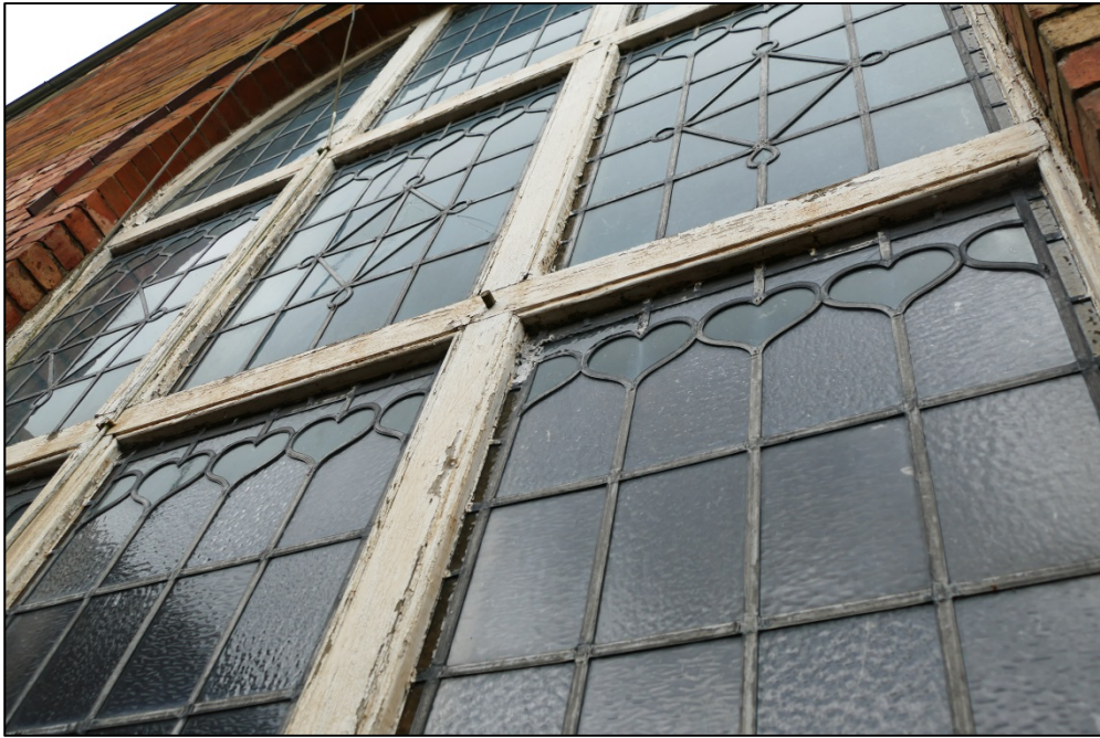
Exterior view of the leadwork and frame of the western hall window Fig 64
