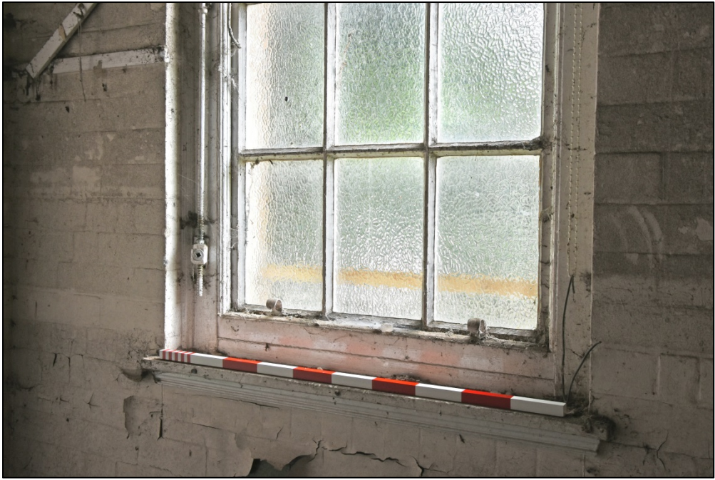
Detail of the base of the window, showing the winding mechanism Fig 74
