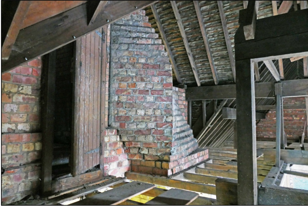
The spiralling brickwork of the tower support, and door to tower landing Fig 36
