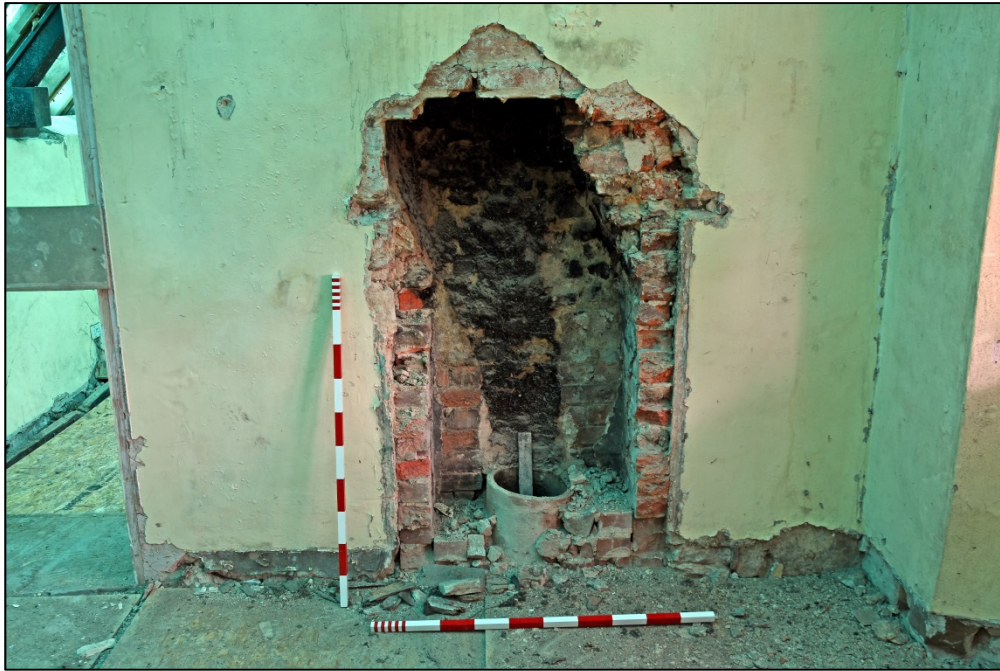
Detail of chimney flue in the east wall of room F1 Fig 40
