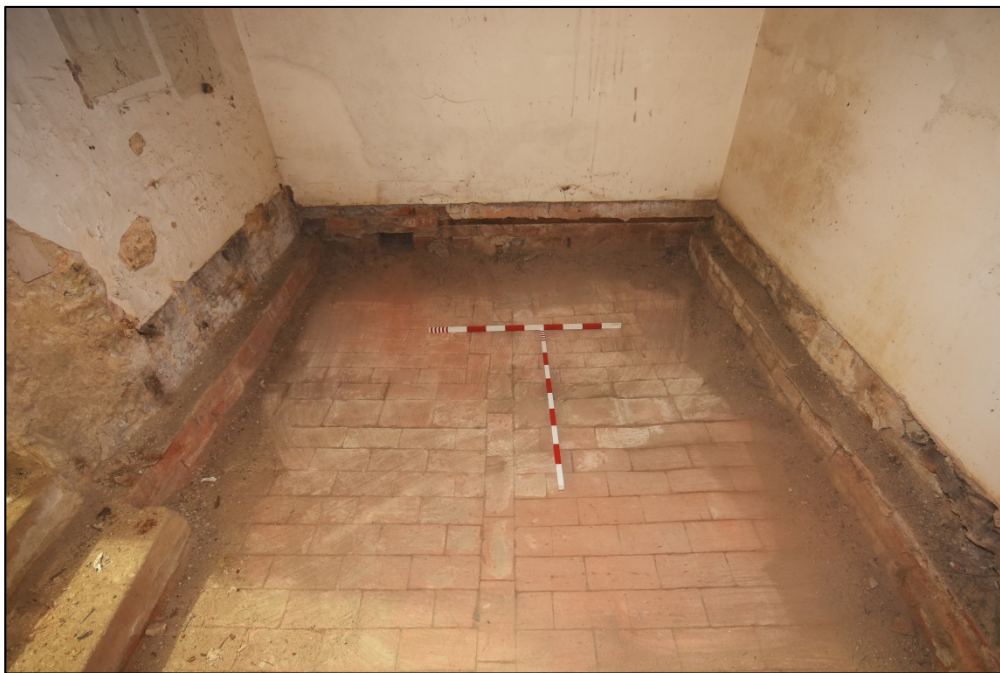
The floor of room G2, showing the brick plinth relating to the lowering of the floor Fig 25
