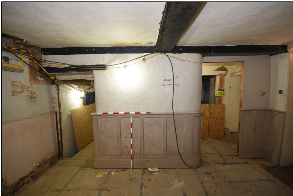
Room G1, looking east, showing 19th-century wainscoting and doors to the stair landing and corridor Fig 21
