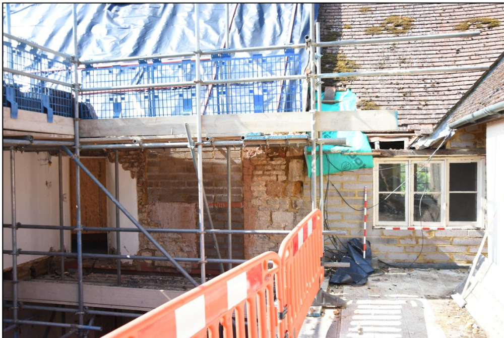
Detail of first floor remediation works, south wall of F3 and F5 Fig 65
