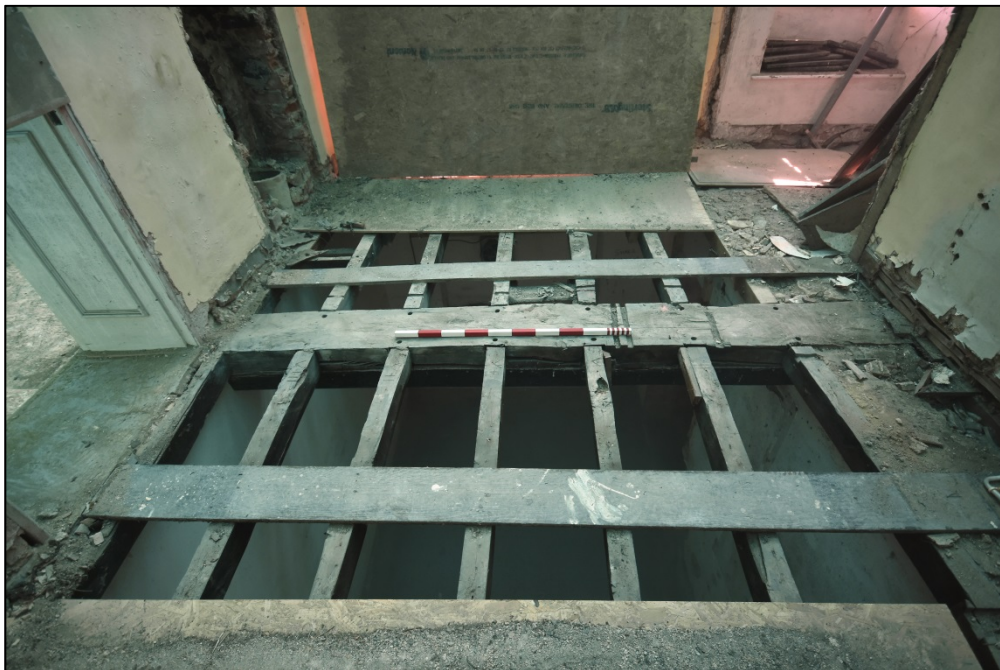
Overhead view of the spine beam and joists of room G2 Fig 23
