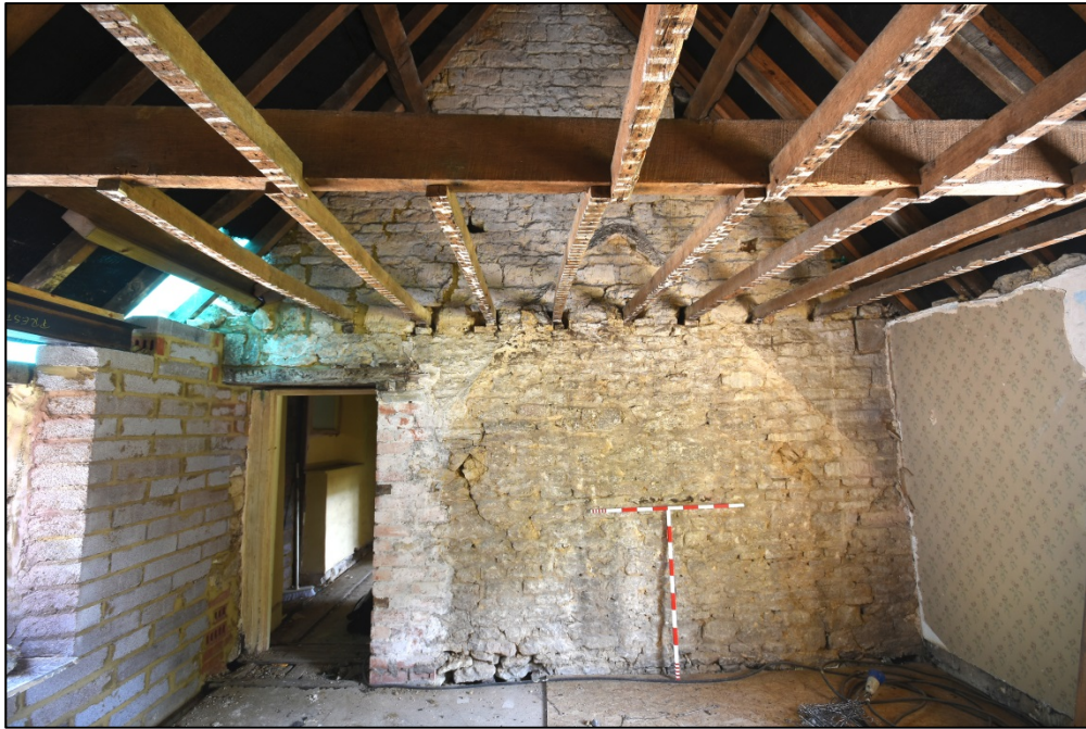
East wall of room F5, showing the mark of a former gable Fig 52
