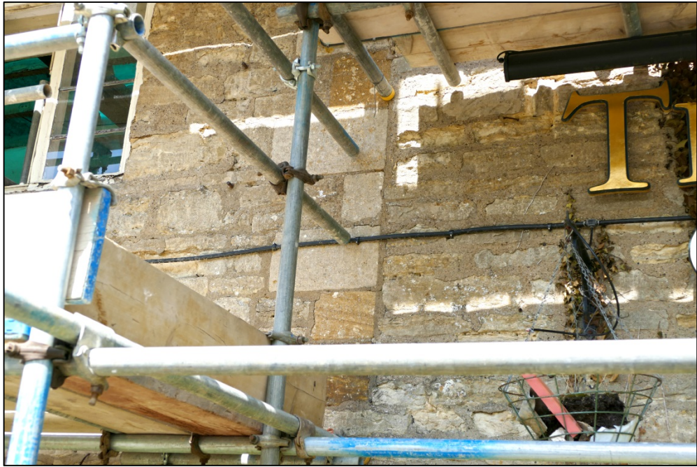
Detail of quoins at first floor level, showing join between the east and central blocks Fig 12
