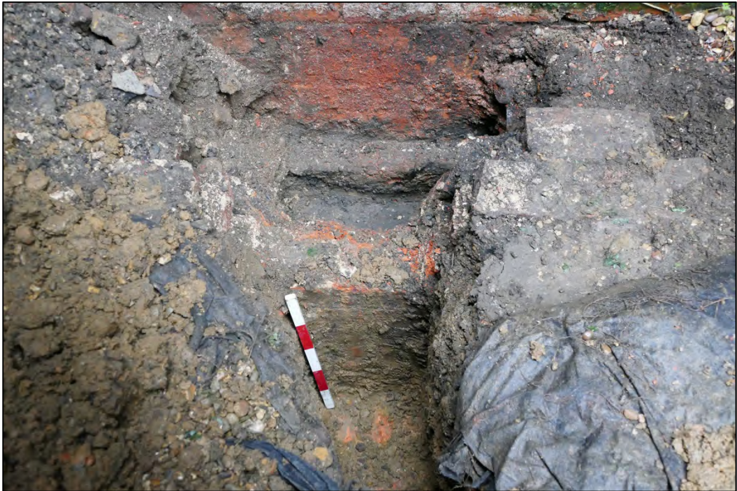
Foundation trench 3, showing the brick gully with pipe adjacent to the wall Fig 148
