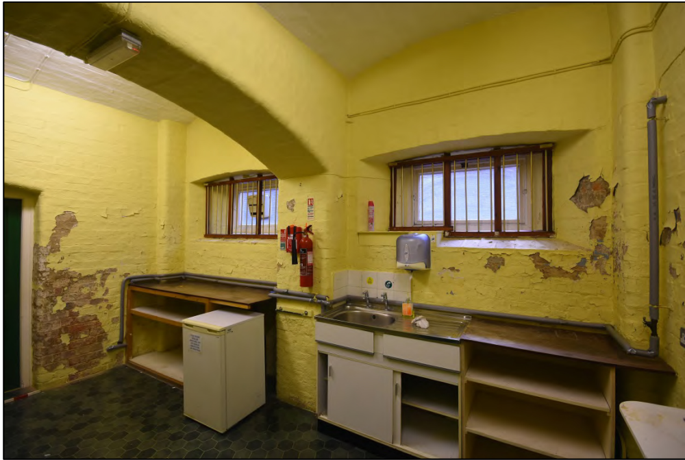
The museum basement, former kitchen with jack vaulted ceiling and arch between former cells Fig 38
