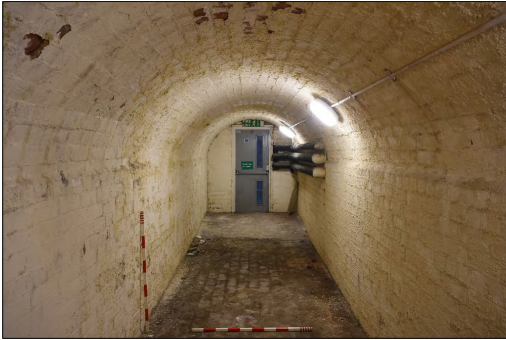
The brick arched passageway at the north-east of the west gaol wing Fig 88
