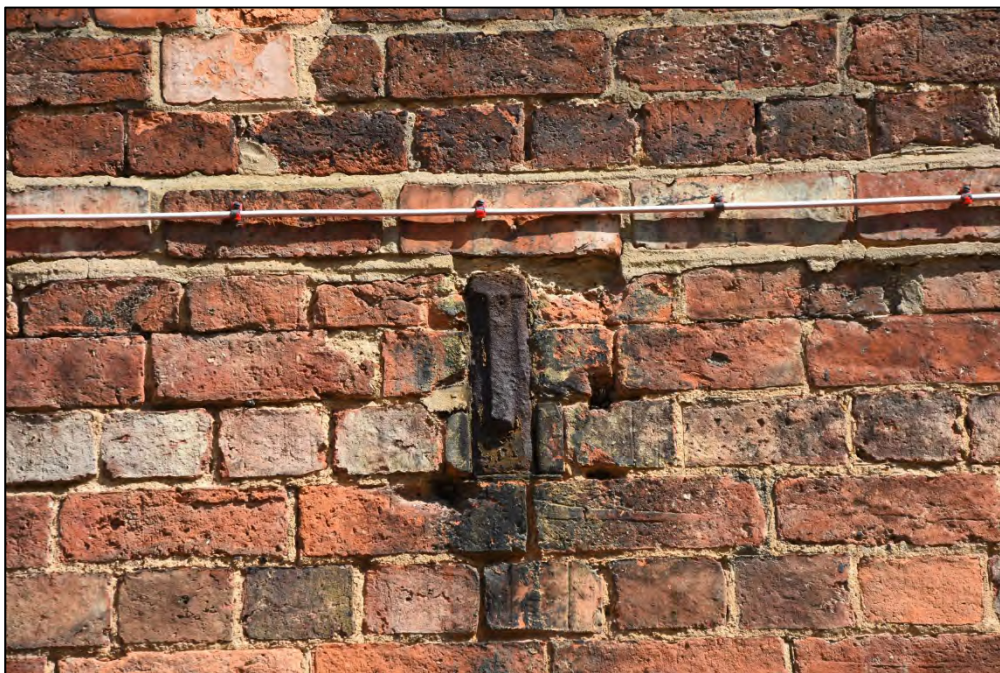
Detail of truncated supporting bracket for the former elevated platform Fig 63
