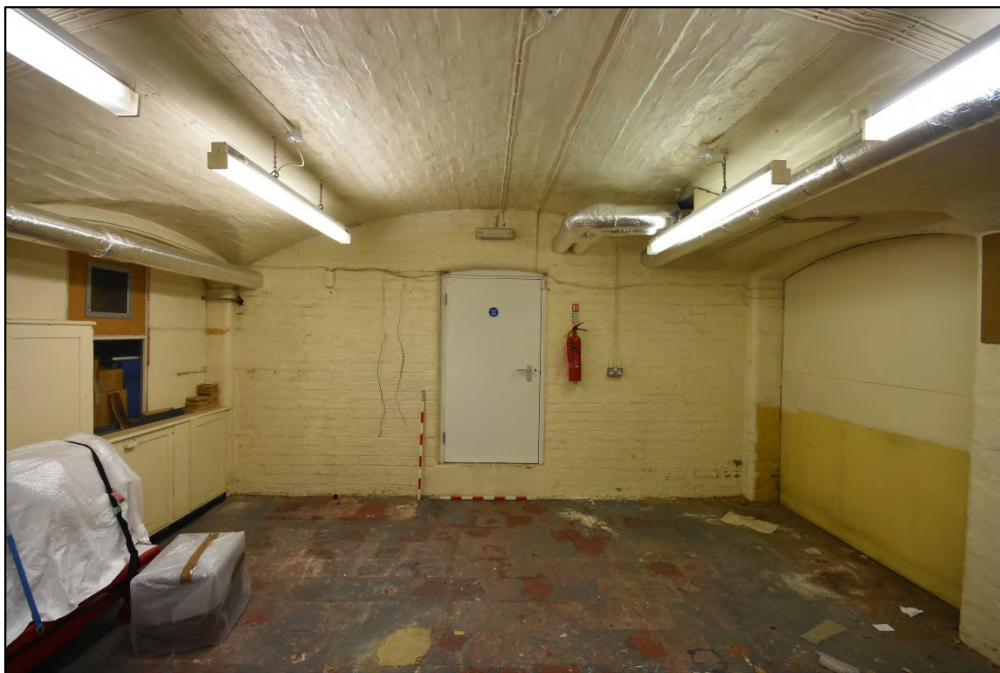
The basement, central corridor looking west, with door to the boiler room Fig 39
