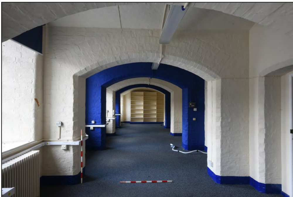
The former cells at the western side of the lower ground floor, looking north Fig 83
