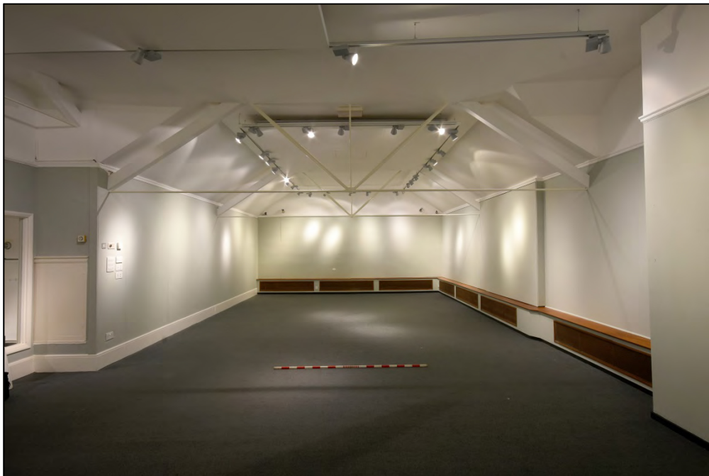
General view of the first floor rooms, looking west, showing steel roof trusses Fig 49
