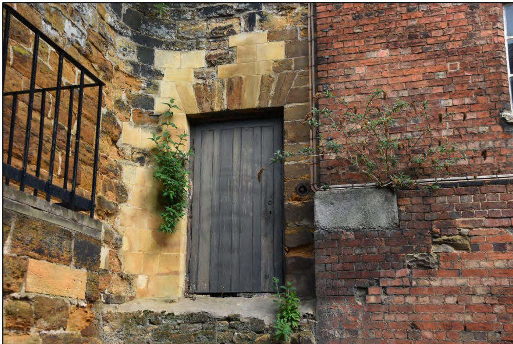
Blocked door formerly leading to the north entrance of the gaol. Note bell pull adjacent to door Fig 65
