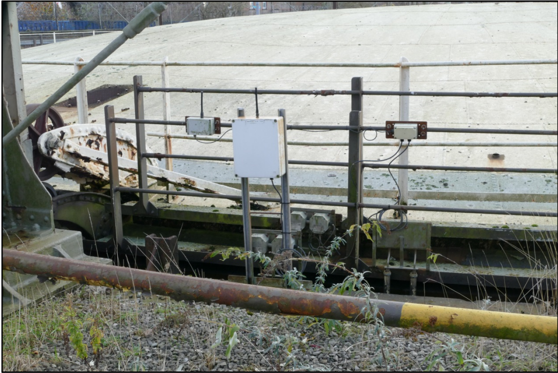
Detail of telemetry and electrical fittings, Gasholder 3 Fig 25
