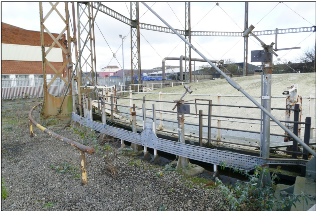
Detail of hammer switches, electrical cable trays and anti-freeze pipe, Gasholder 3 Fig 26
