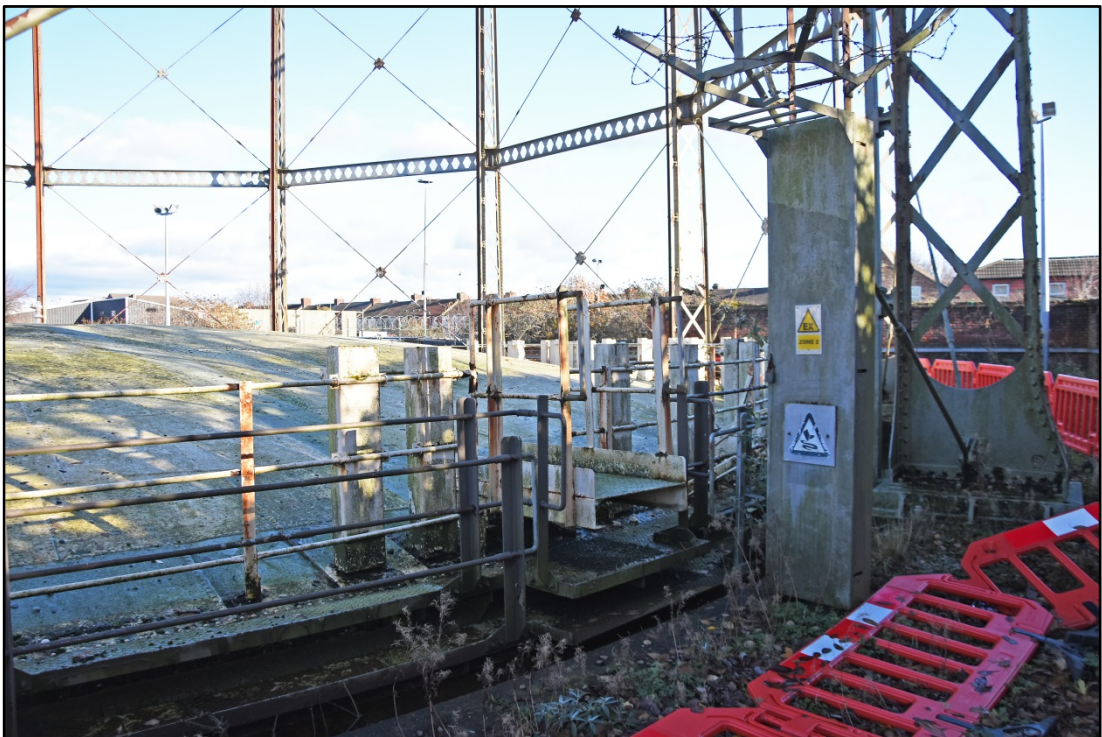
Crown walkway and ladder access, Gasholder 1. Note adjacent concrete filled boxes Fig 22
