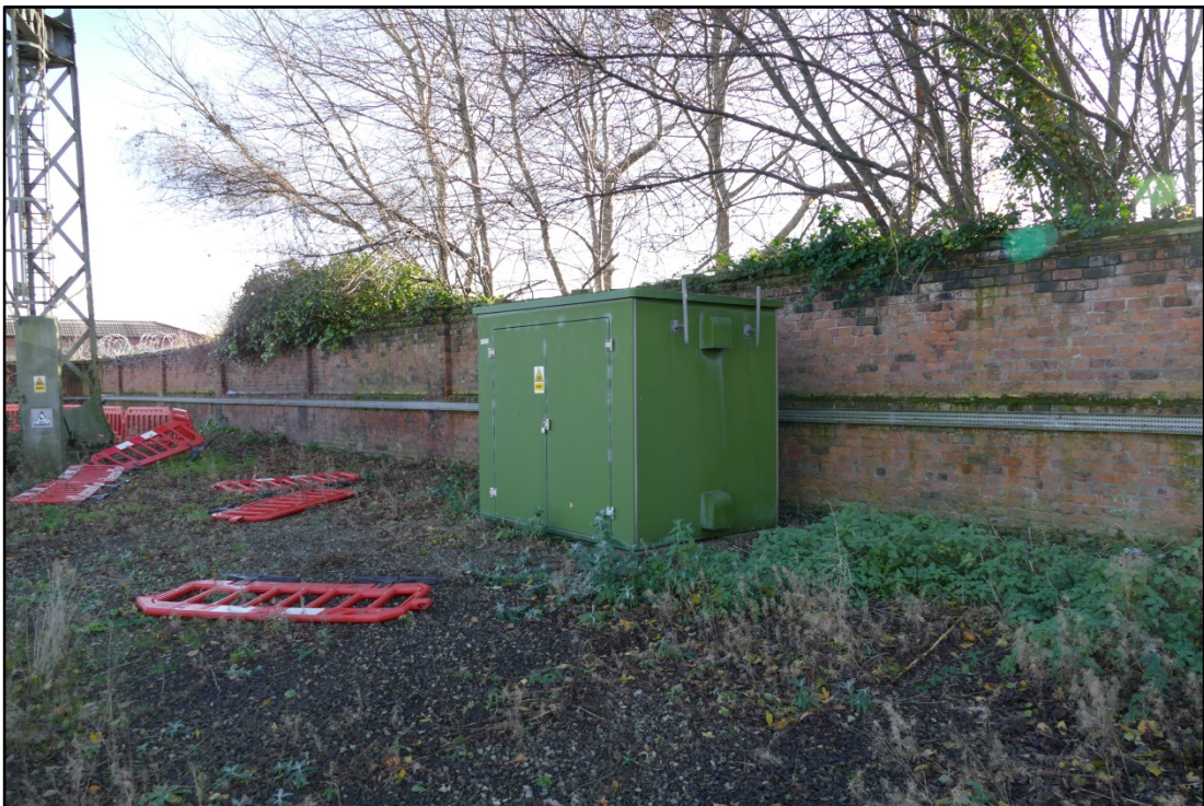
The Pressure Reducing Station Fig 50
