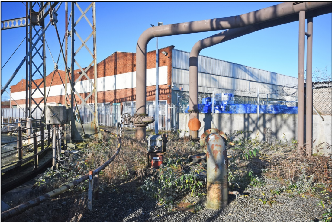
Defunct elevated mains and other pipes at the north-east side of Gasholder 3 Fig 28
