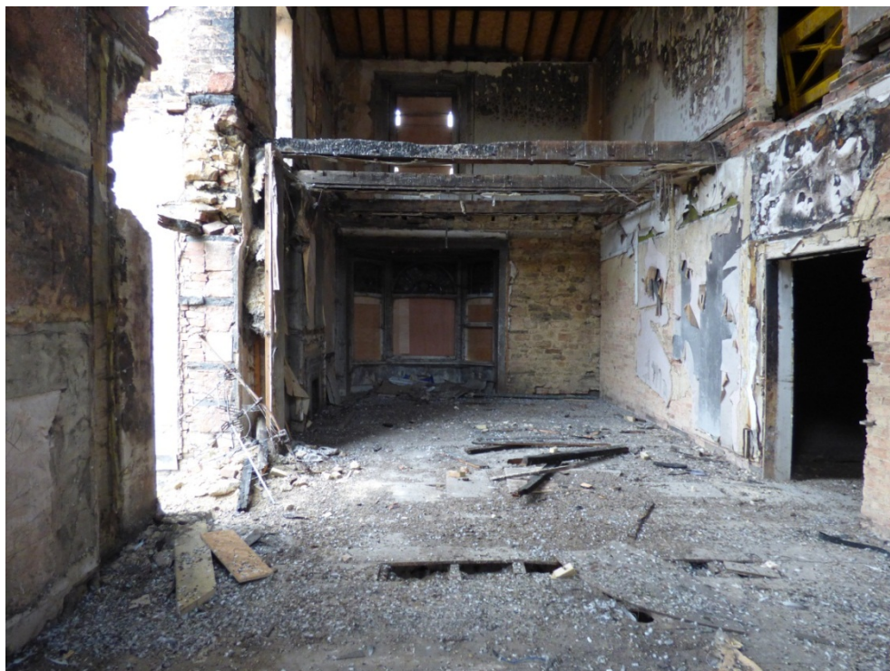
View of bay window and fire damage on the first floor over Balloon Bar, looking west towards Bridge Street Fig 7
