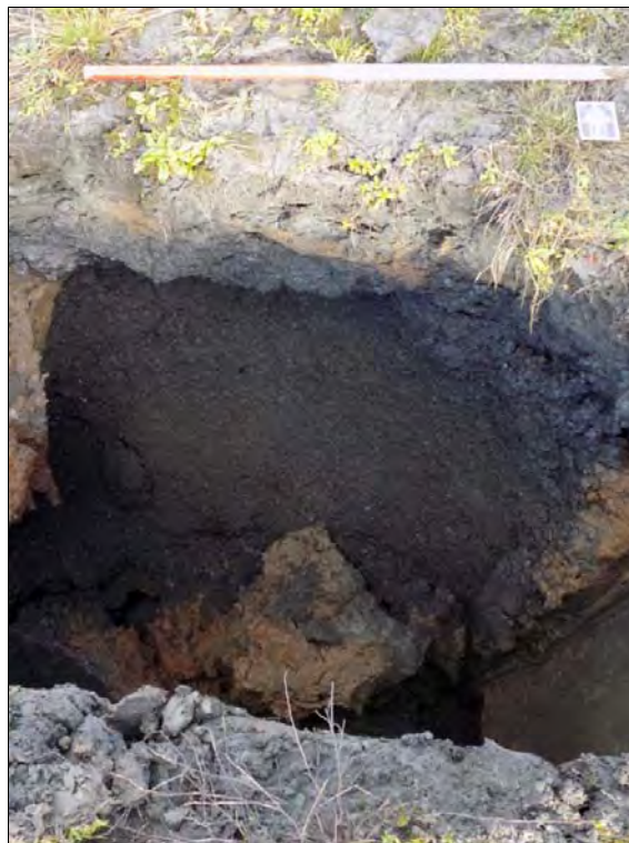
TP 113, Large bell pit with unstable sides, looking north Fig 19
