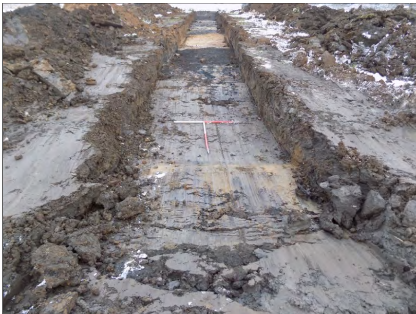
Trench 21, Extensive open-pit cuts, [2105] and [2106], on both ends of the trench, looking east Fig 24
