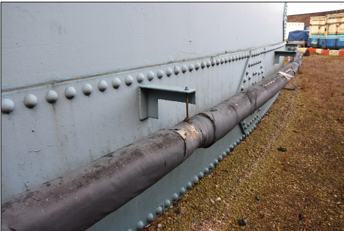
Detail of brackets carrying lagged pipes Fig 14
