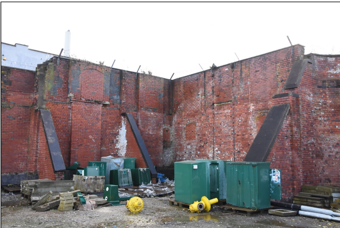
General view of the wall at the corner of Sussex Street and Sussex Road Fig 36
