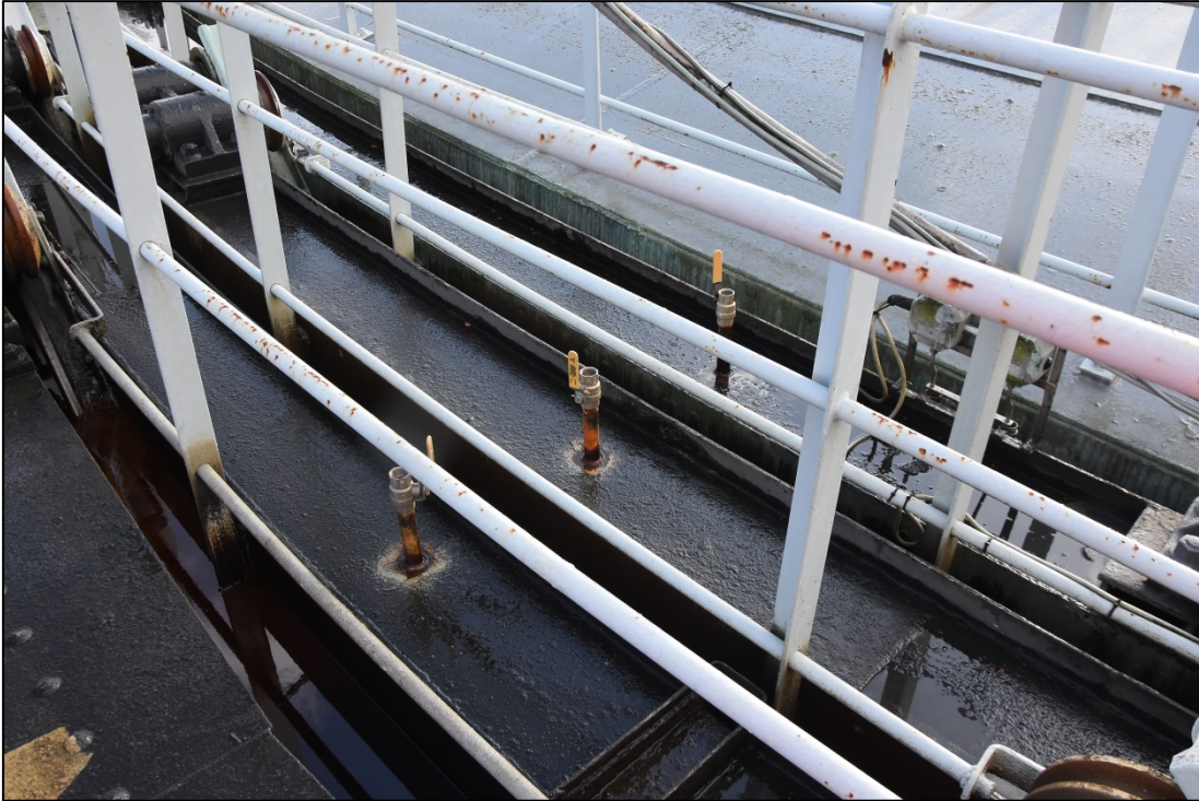
Detail of the lift grips with valved pipes protruding through (recent additions?) Fig 29
