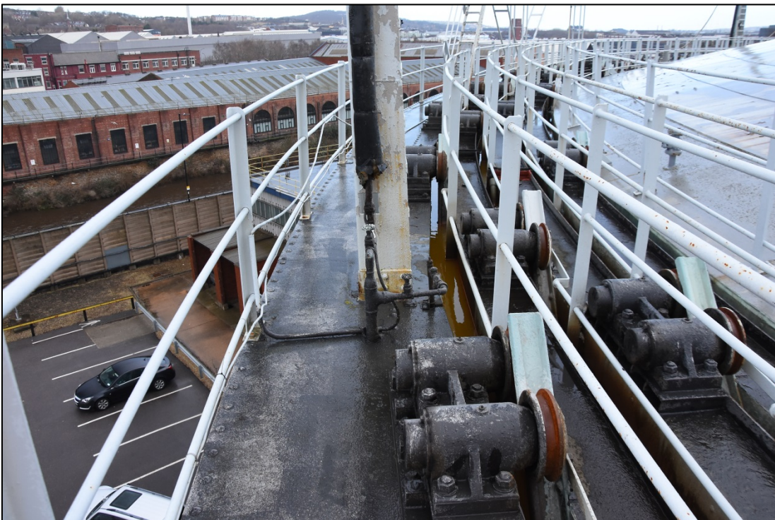
The arrangement of roller carriages, also showing manual valve controls on an antifreeze pylon Fig 28
