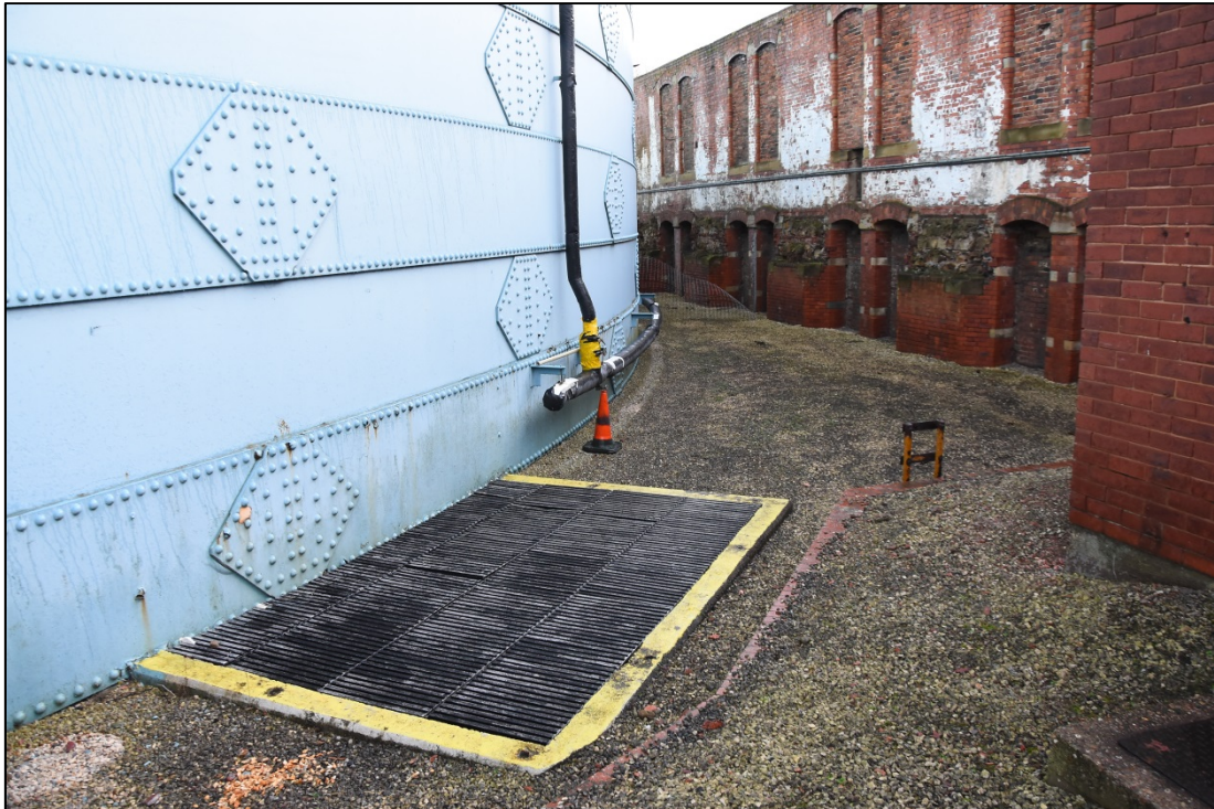
The sump pit over the blanked inlet and outlet pipes at the south-west side of the gasholder Fig 33
