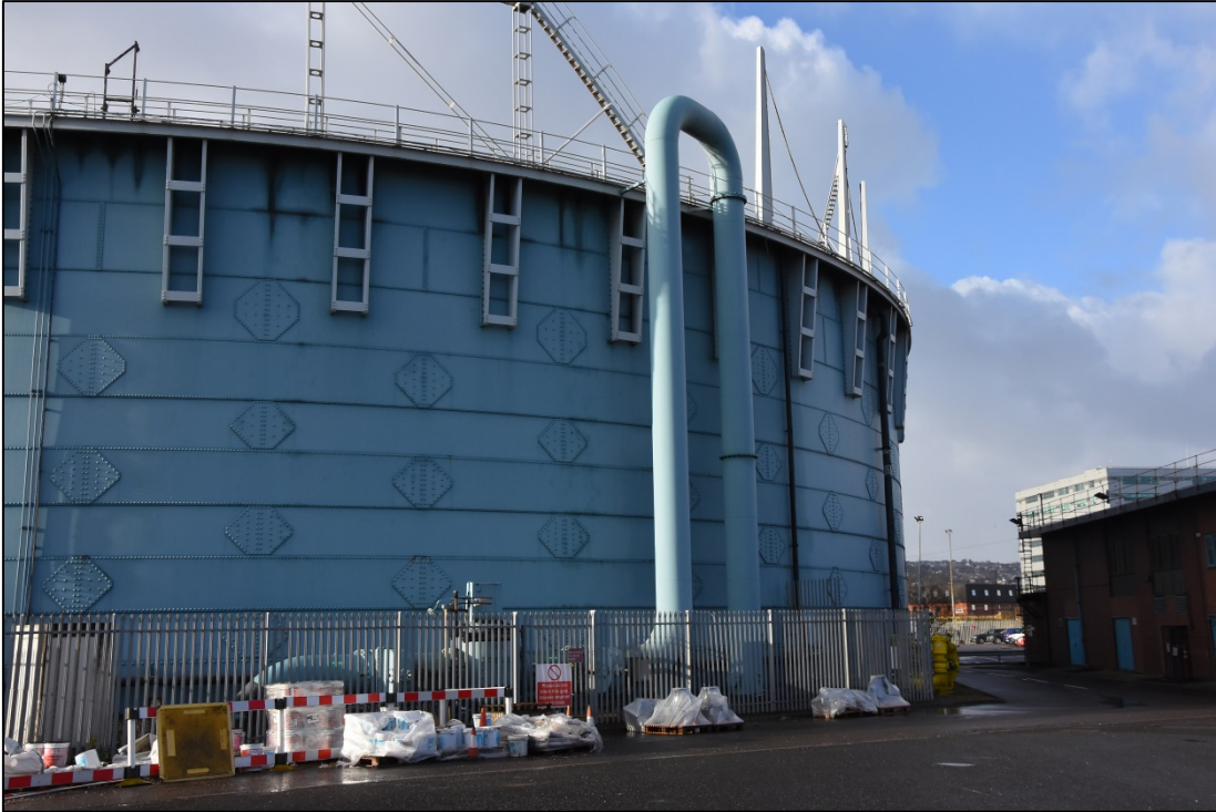
The common inlet and outlet pipes at the north-east side of the gasholder Fig 31
