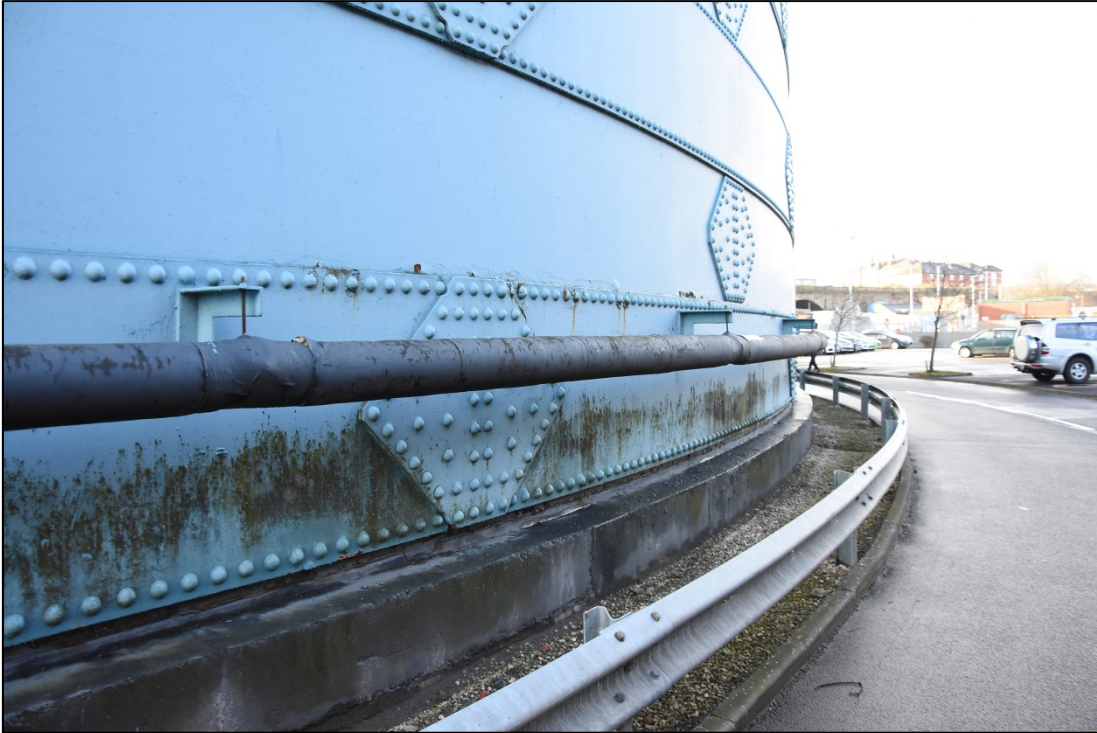
The concrete base exposed at the north-west side of the gasholder Fig 15
