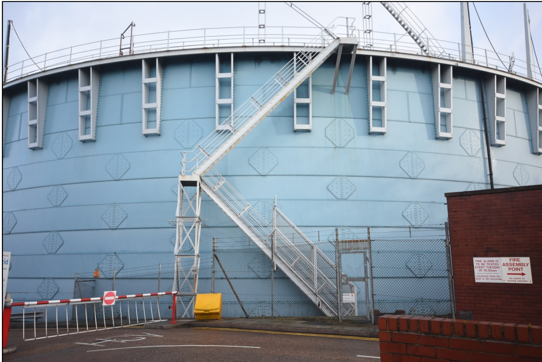
The main stair located at the south-west side of the gasholder Fig 17
