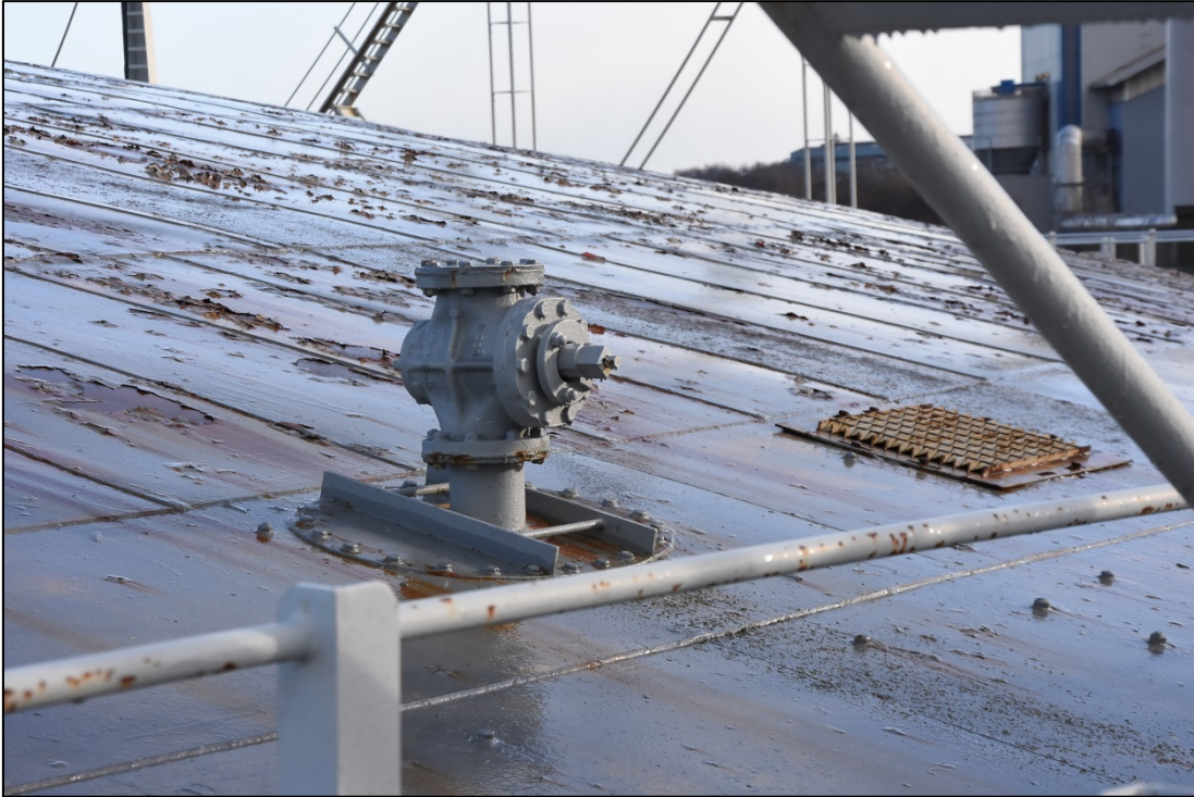
Gas valve and manhole at the south side of the crown Fig 21
