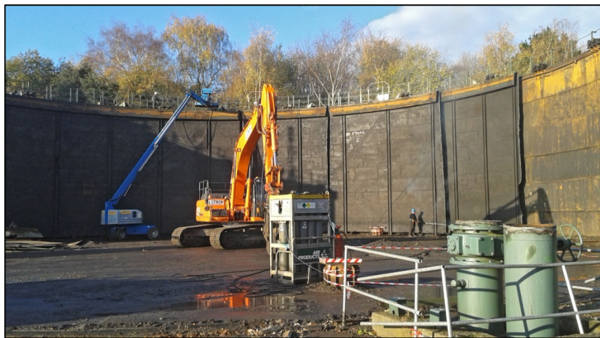
The gas holder during dismantling, note inlet and outlet pipes in foreground Fig 23
