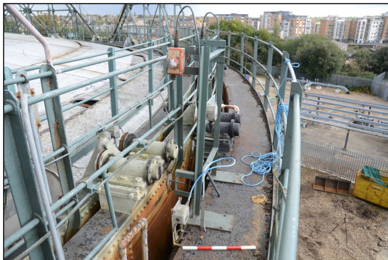
Detail of holder height controls at the south side of the gasholder Fig 20
