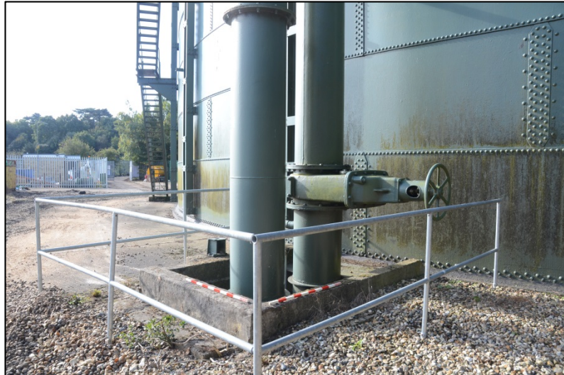
The inlet / outlet pipes and dry well Fig 13
