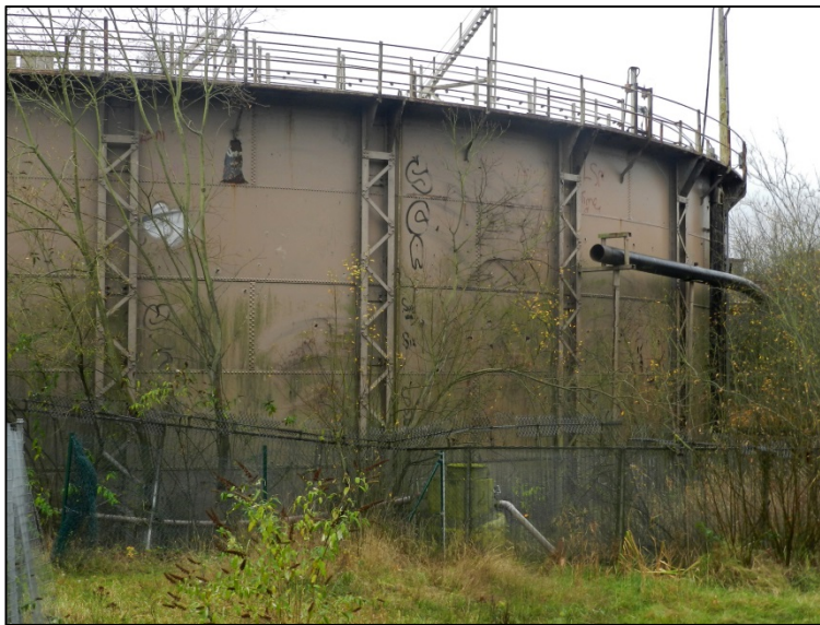
View of the tank and pilasters, also showing truncated gas pipe Fig 6
