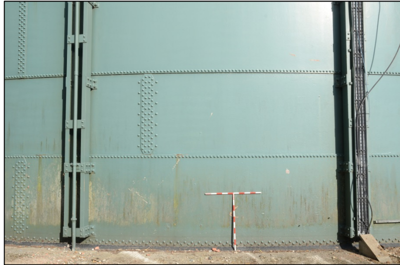
Detail of the tank sheeting, note electric cables and pipes on the pilasters Fig 10
