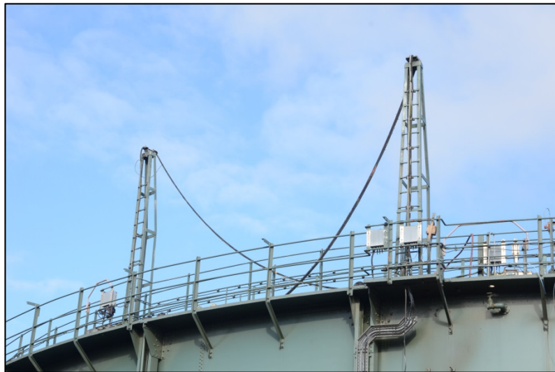
The anti-freeze pipes and pylons at the south side of the gasholder Fig 14
