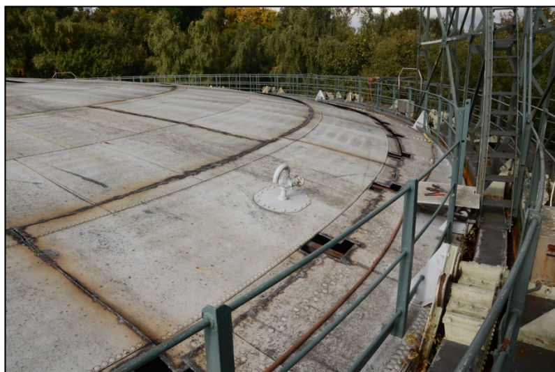
View of the crown top curb, also showing valve and manhole Fig 21
