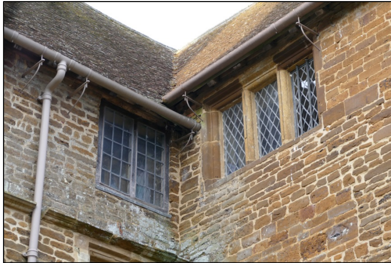
The misaligned eaves level between the north and west ranges Fig 53
