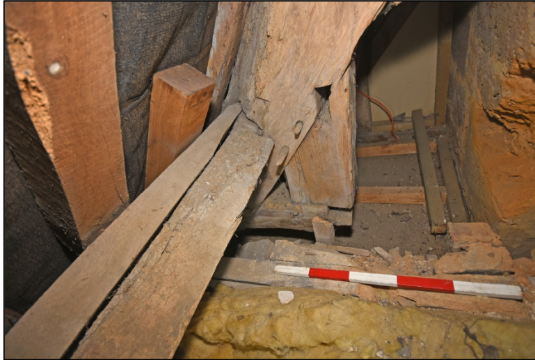
Ceiling framing timbers surviving on Truss N2, with chimney breast to the right Fig 248
