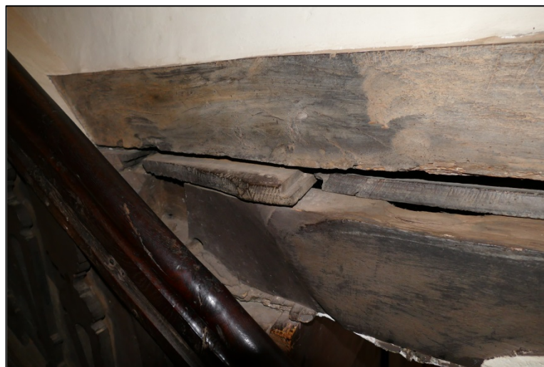
Truncated floorboards below the stairwell wall, viewed from the stair Fig 177
