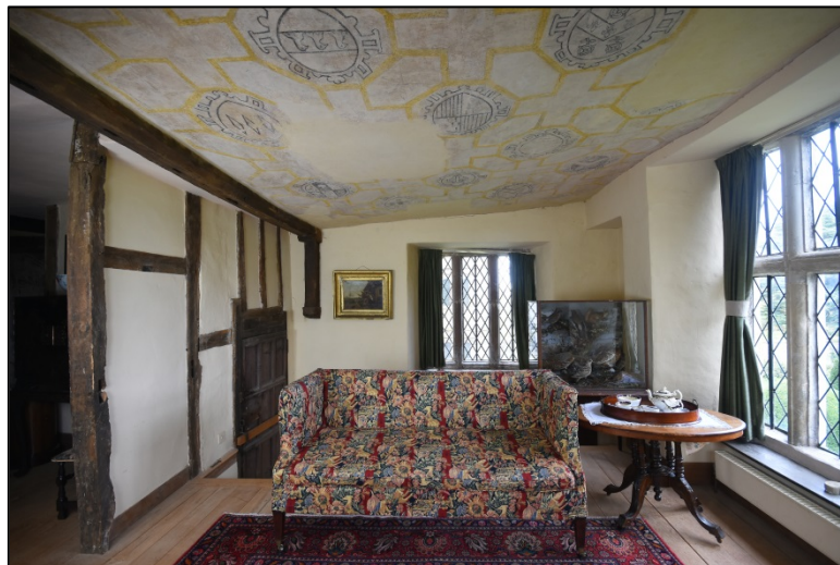
The Sitting Room, looking south; showing the extent of sloping of the ceiling Fig 179
