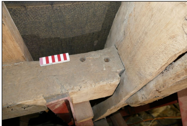
Truss N3, detail of bridle scarfed purlin with empty double peg holes Fig 252
