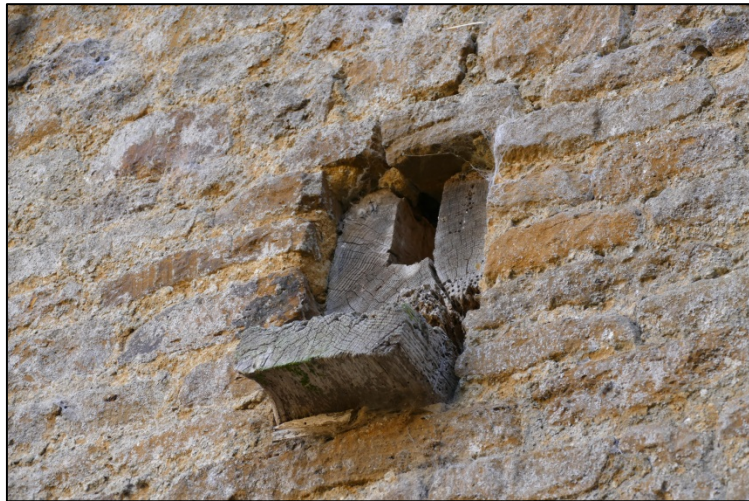
The exposed end of a tie beam with footing for a raised cruck, Truss E2 Fig 61
