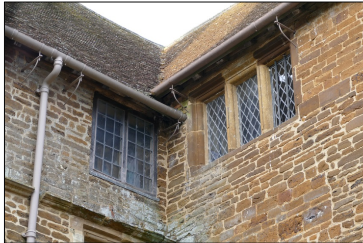
The misaligned eaves level between the west and north ranges Fig 78
