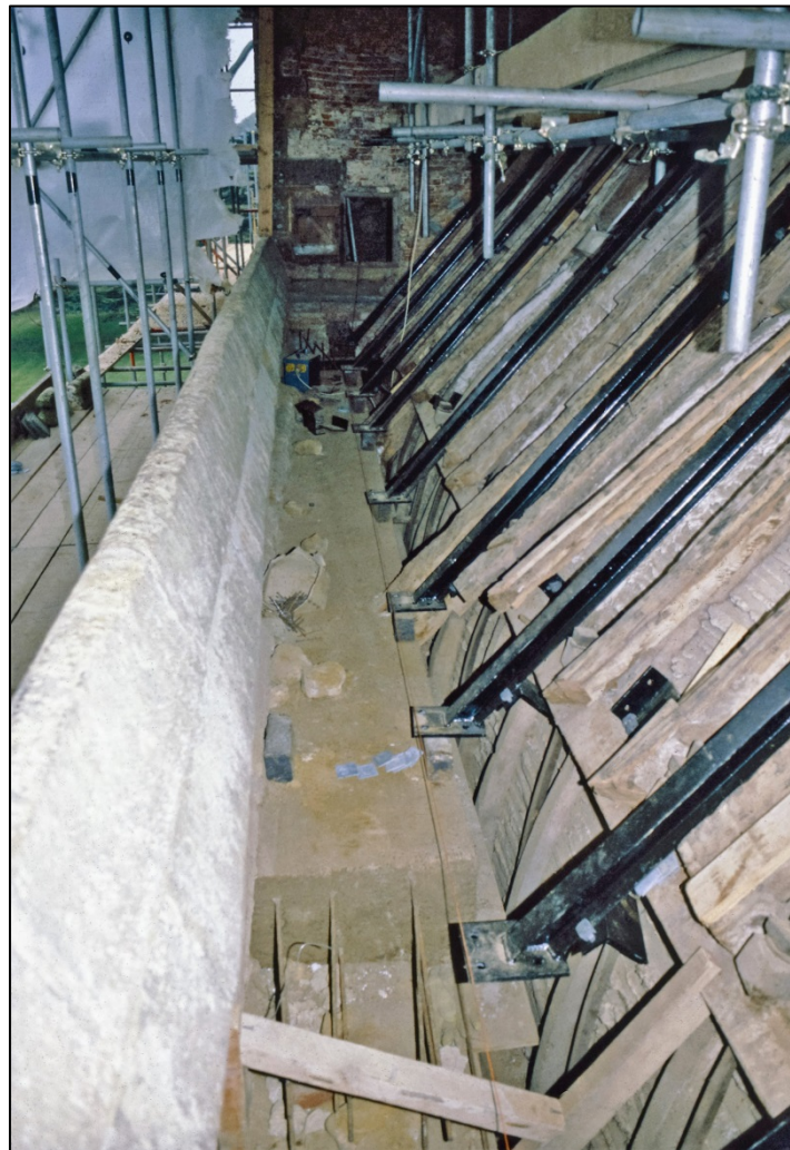
1980s view of the Drawing Room ceiling and rafters with parapet leadwork removed (CANT35RED) Fig 279
