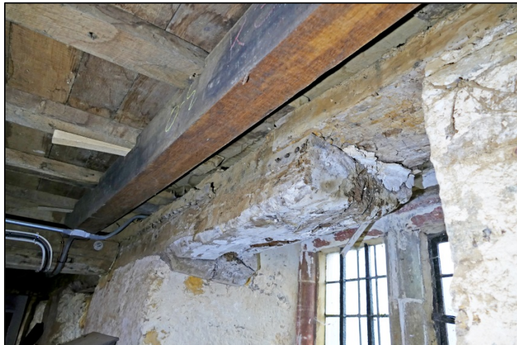
Beam embedded in the south wall to support the bridging beams and joists Fig 91
