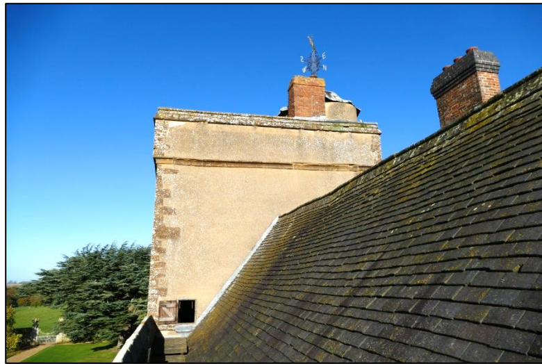
The eastern elevation of the tower with hatch access from the Sitting Room Fig 221
