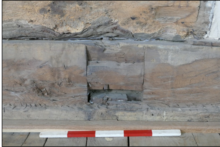
Defunct double tenon joint on lower beam Fig 158
