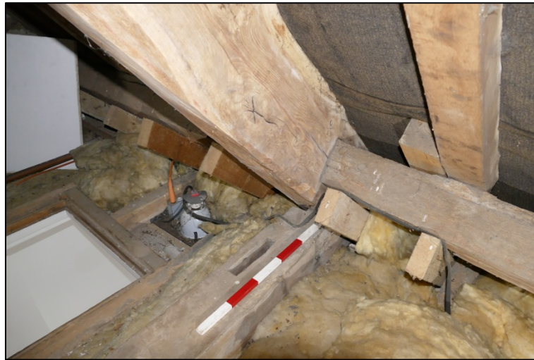
Detail of the lower north side of Truss N4; note defunct mortice on collar Fig 254
