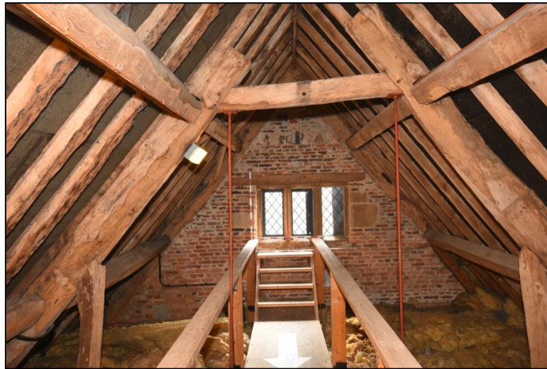
The brick gable at the south side of the west range roof Fig 269
