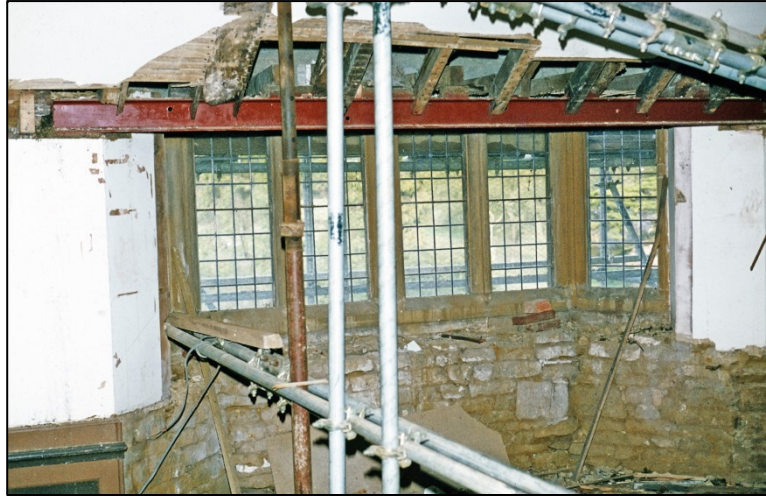
The north wall window during conservation works, showing the wall fabric (CANT58GN) Fig 207
