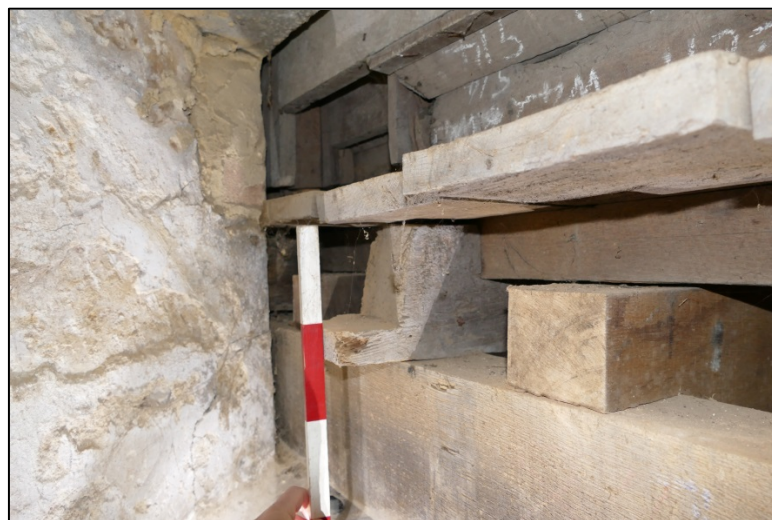
View of the back of the panelling from the cellar, Room C6 Fig 114
