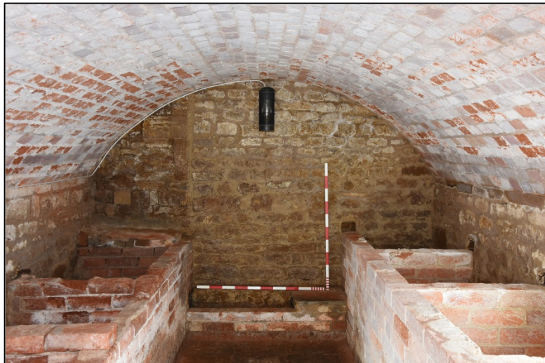
Vertical joint in the west wall of Room C10 Fig 100
