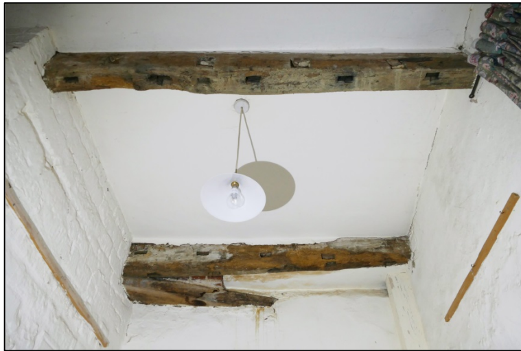
The underside of Truss E4 and adjacent beam; note empty mortices on sides and underside surfaces Fig 110
