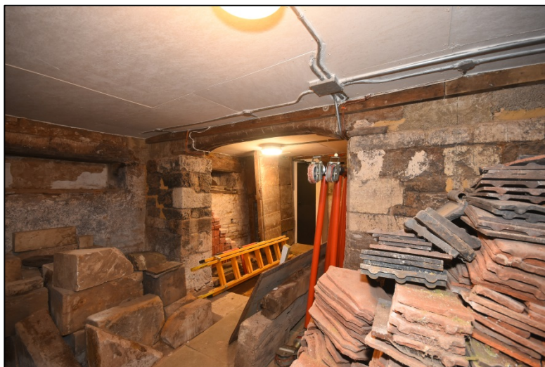
Masonry wall and timber beam at the west side of the tower Fig 94
