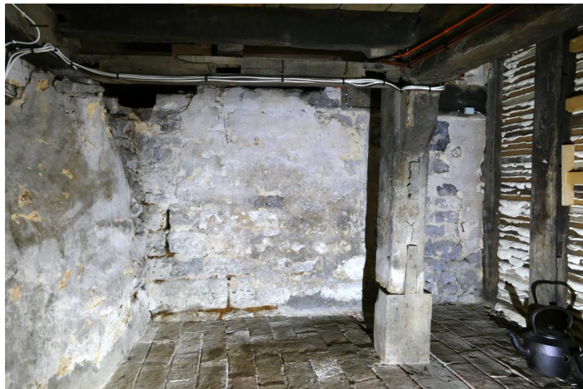
The under-stair space; note stone walls and defunct joints in supporting post Fig 187
