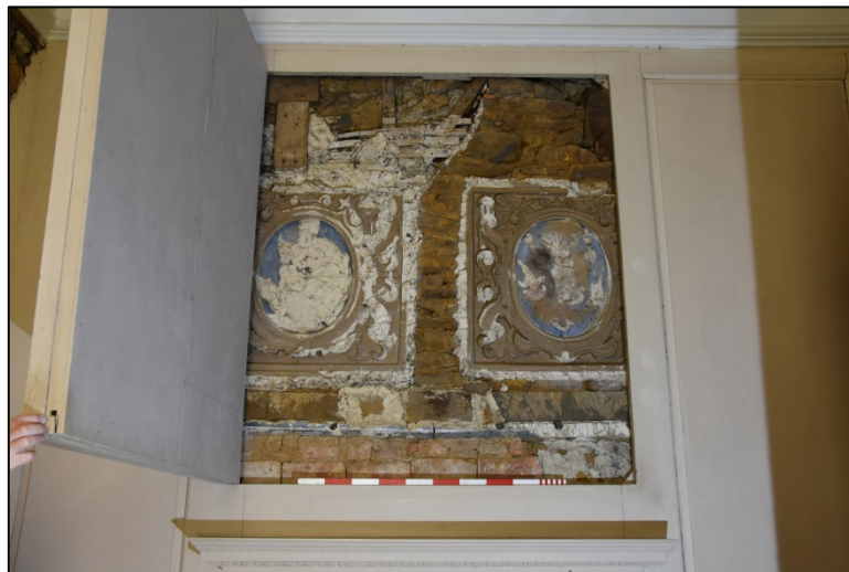
Brickwork and plaster panels behind the panelling of the north wall Fig 160
