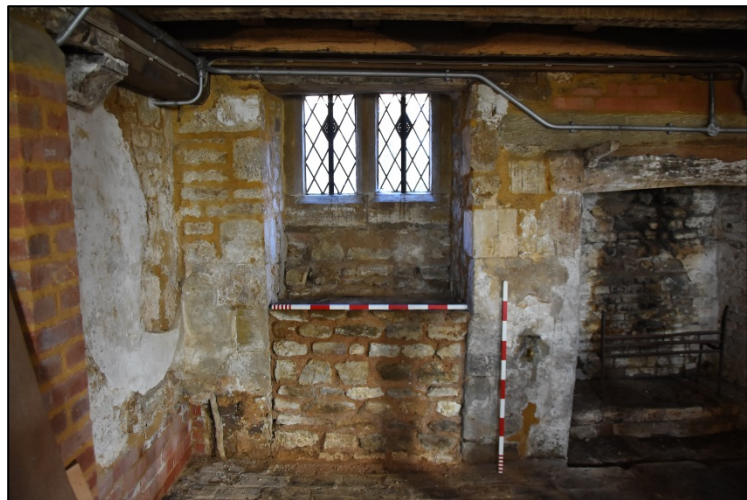
Blocked door in Room C3 Fig 88
