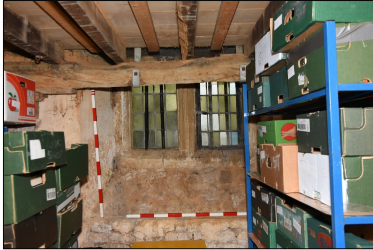
The lowered joist rail at the south side of the room Fig 83
