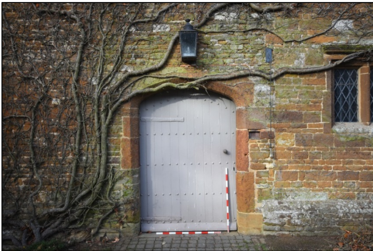
The passageway door. Note vertical and horizontal joins and change in fabric Fig 44
