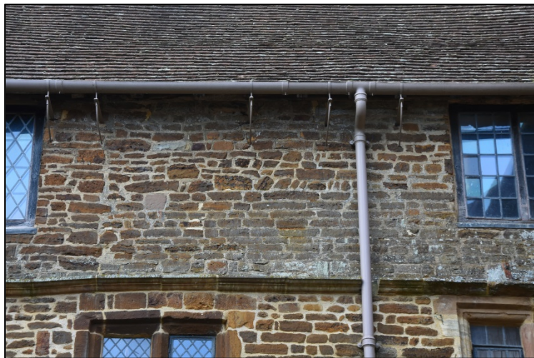
Probable change in fabric between the former farmhouse and the west range Fig 76
