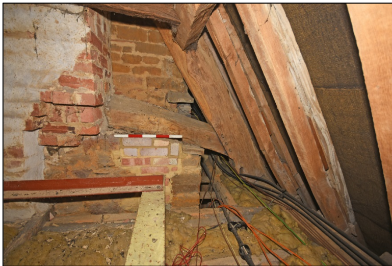
The south side of Truss N2; note furring of rafters and brick flue added to the chimney stack Fig 249
