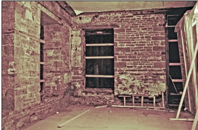
The south-west corner of the Dining Room with panelling removed (CANT30GN) Fig 113
