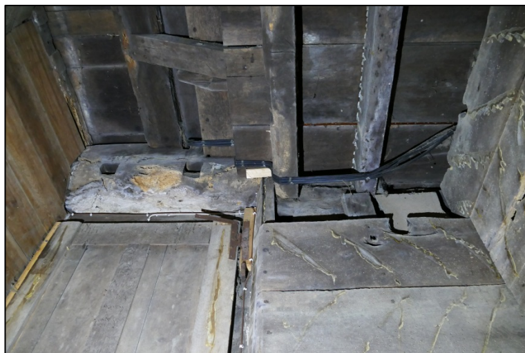
The underside of the stair landing; note defunct joist slots on beam over door Fig 212
