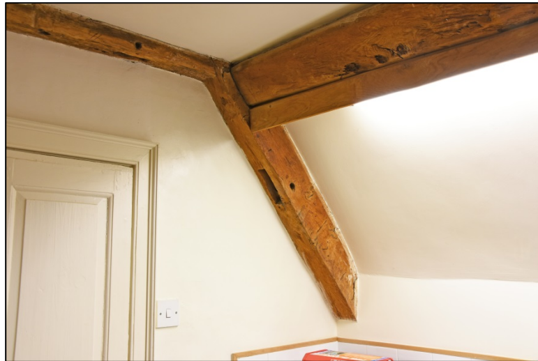
Detail of the rafter, purlin and collar arrangement; note empty pegged slot for middle missing collar Fig 274
