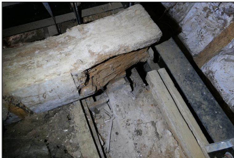
The exposed end of defunct bridging beam; note truncated double mortice Fig 281
