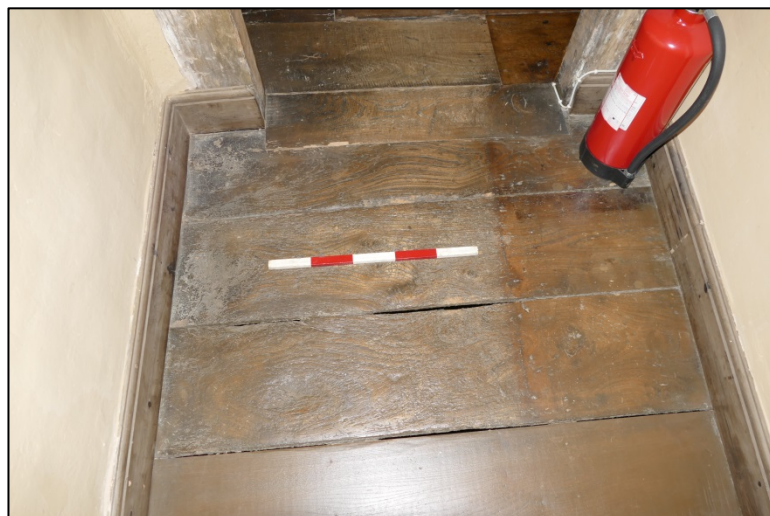
Differential weathering on floorboards suggesting former partition arrangement Fig 170
