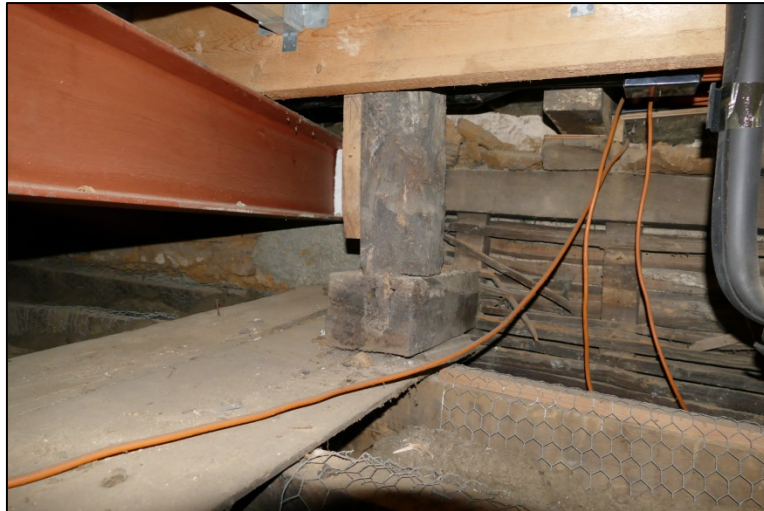
View under the floor; showing the truncated beam under the partition, lath and plaster partition beyond, and the bridging beam and floor board Fig 181
