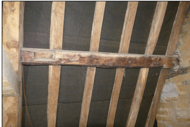
Smoke-blackened timber re-used as a purlin, note defunct joint on the left side Fig 257
