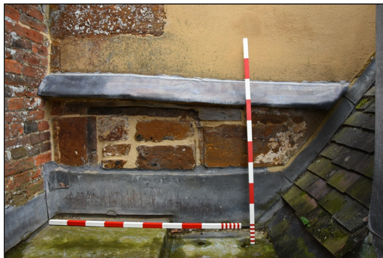
Blocked window in the west elevation of the tower adjacent to the end gable of the west range Fig 222
