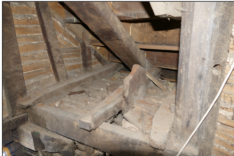
The underside of the mezzanine stair, viewed from within the void over the buffet Fig 148
