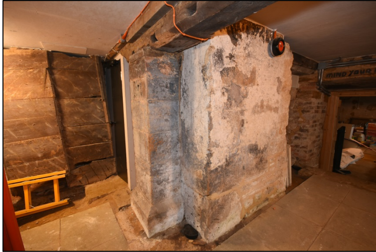
Masonry pier in Room C4. Note defunct mortice slots on bridging beam Fig 92
