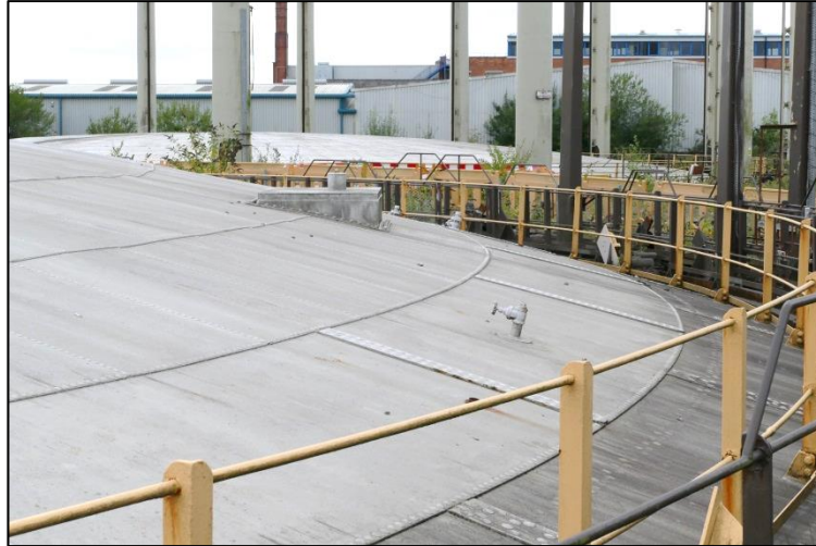
View of the crown, showing Livesey hydraulic access and small vents Fig 12
