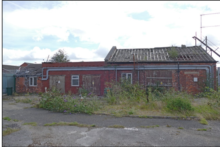
The Governor House and electrical switch room, looking south-east Fig 29
