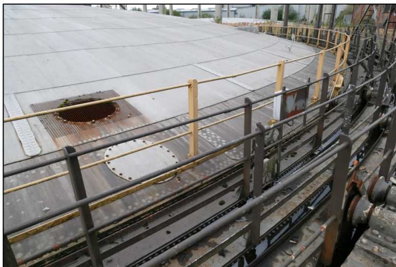
View of the lift grips and crown, also showing flat lid manhole Fig 11
