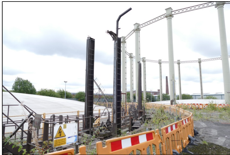
The anti-freeze supporting pylons with adjacent lift platform Fig 13
