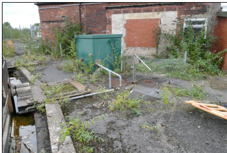
The dry well with overflow pipes leading to the interceptor Fig 17
