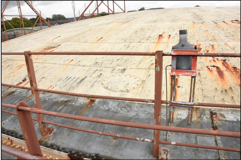
Detail of the crown and top curb, also showing one of the access lids and an oil film applicator Fig 28
