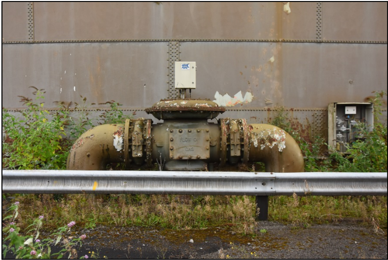
Pipework and adjacent control box at the north-west side of the tank Fig 24
