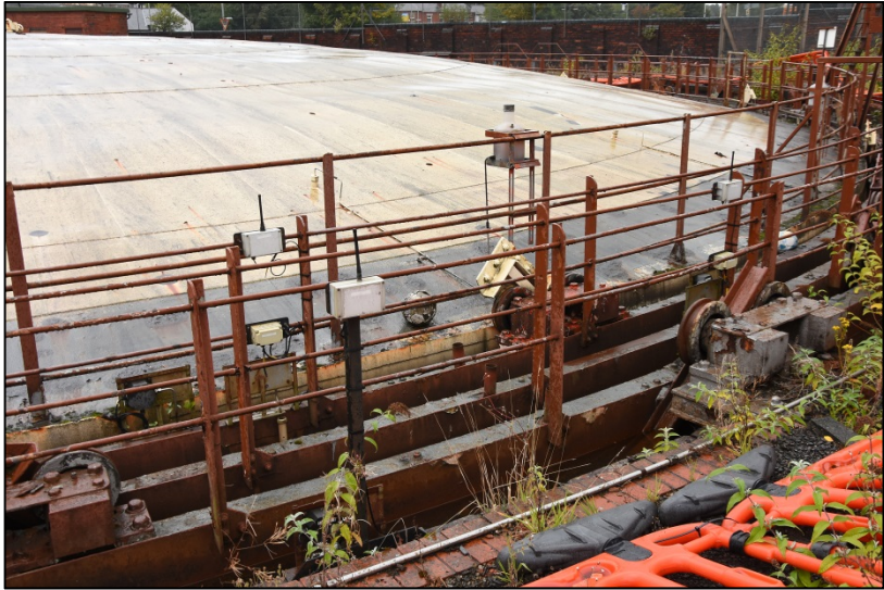
The lifts and hand rails, showing various electrical and telemetry and an oil applicator Fig 10
