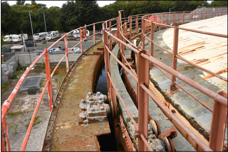
View of the lifts and crown, note 'balancing weights' installed on the 1st and 2nd lift grips Fig 27
