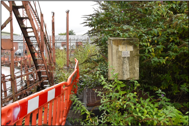
Dry well and pressure controls at the south side of the gasholder Fig 16
