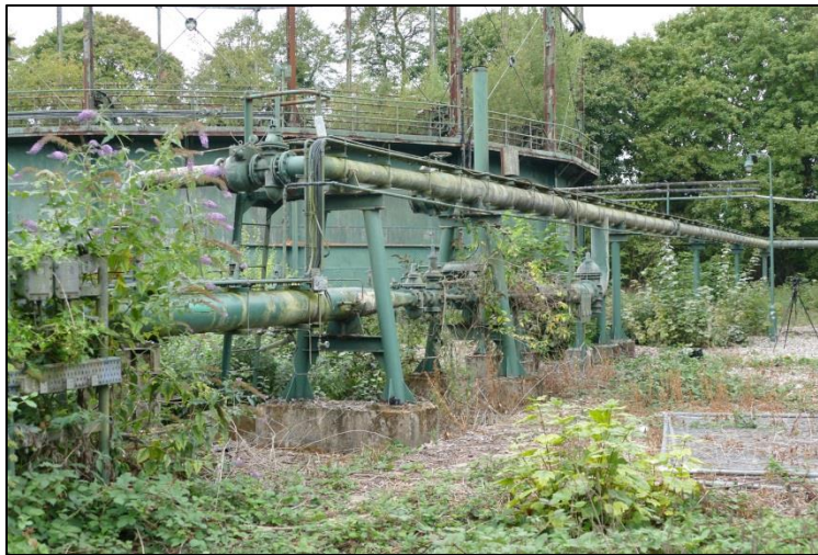
View of the pipes adjacent to the gasholders Fig 28
