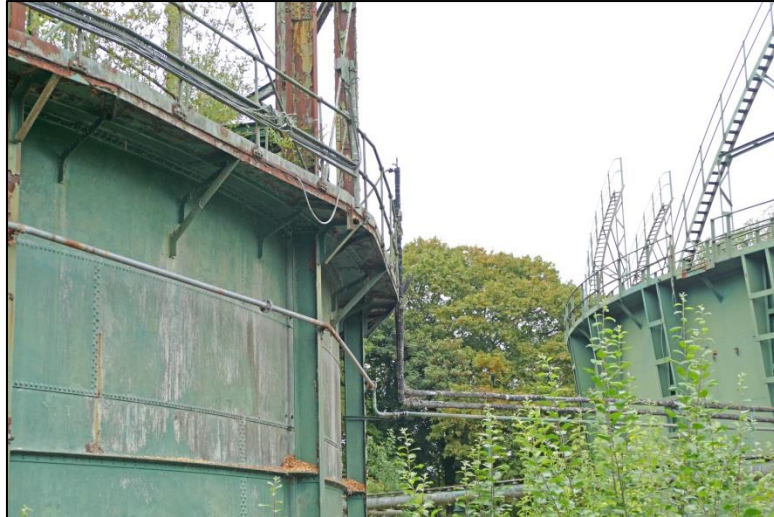
Detail of lagged pipes and overflow pipes Fig 19
