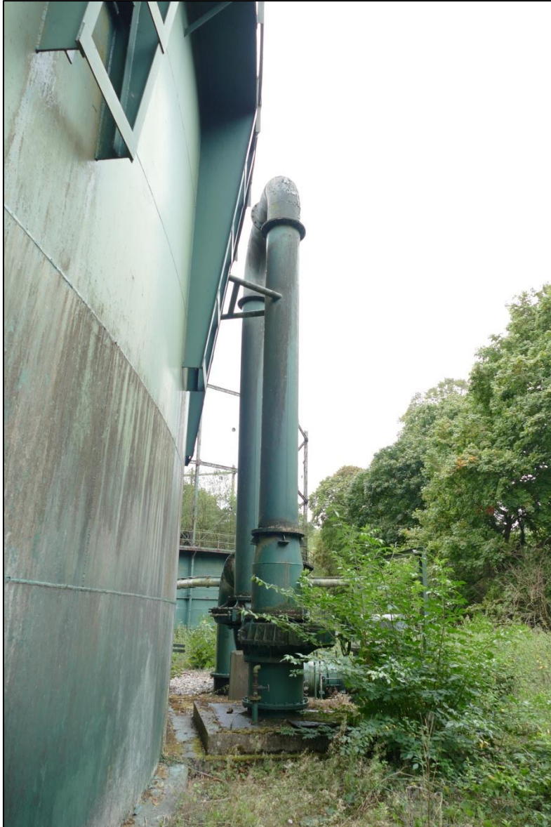
The inlet and outlet and pipes Fig 25
