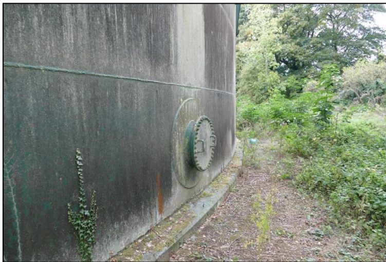
Access point on the north-east side of the gasholder, also showing the concrete base Fig 23
