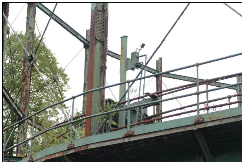
Hammer switches on the tank; note also overlap plate between the framing members Fig 18
