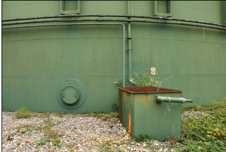
Lagged pipes, overflow pipes and interceptor; note adjacent access point Fig 22
