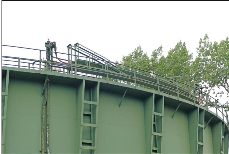
Detail of anti-freeze valves and supporting trays Fig 27
