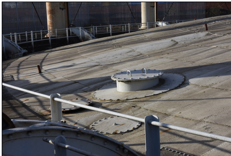
Paired flat lids and adjacent manhole over the inlet and outlet pipes Fig 43
