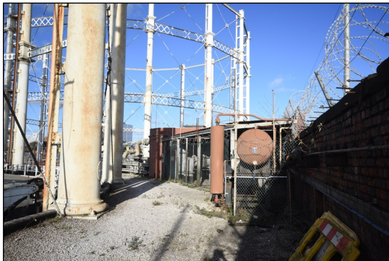
View of pipework and Generator House with MEG tank in foreground Fig 55
