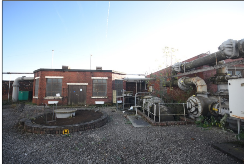
The Booster House and Generator House, looking east Fig 53
