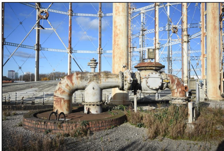
The inlet and outlet pipes, valves, and dry well at the south-east side of Gasholder 4 Fig 44
