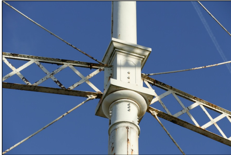
Example of the middle tier junctions, showing entablature box and girders Fig 14
