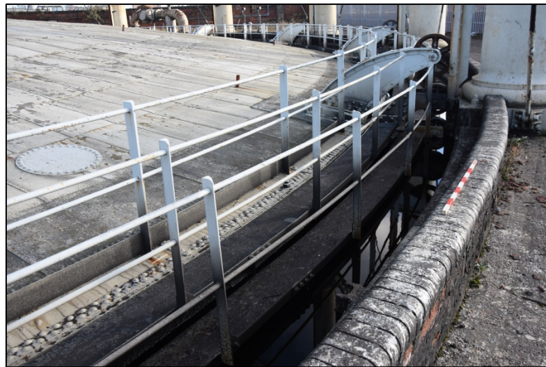
View of the tank kerb and the lift walkways and handrails Fig 40
