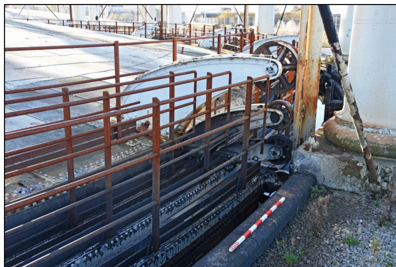
The roller carriages, also showing the tank kerb and lifts Fig 16
