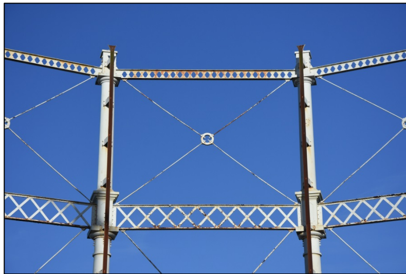
View of the inner face of the upper framing of Gasholder 3 Fig 9
