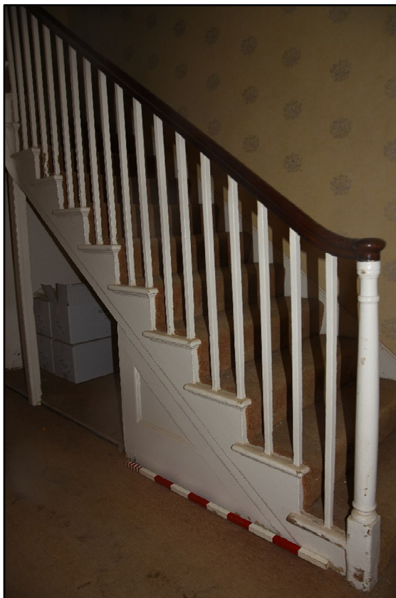
Staircase in GF01 giving access to the first floor, looking north Fig 22
