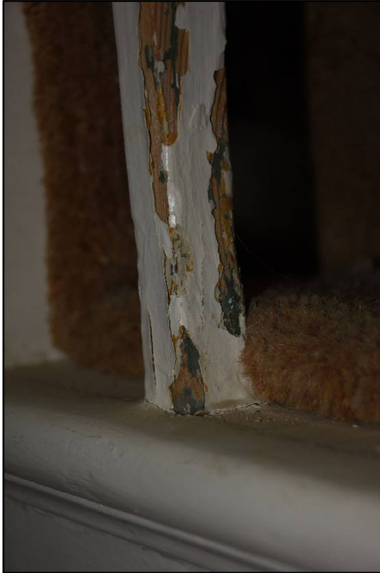
Evidence of paint on the stair balusters in GF01, looking north Fig 23
