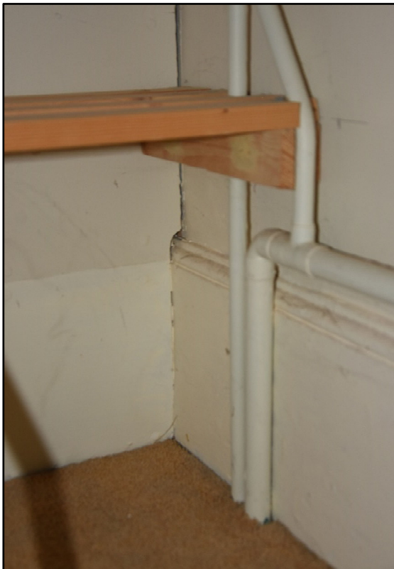
Detail of inserted east wall in FF01a cut around original skirting, looking south-east Fig 74
