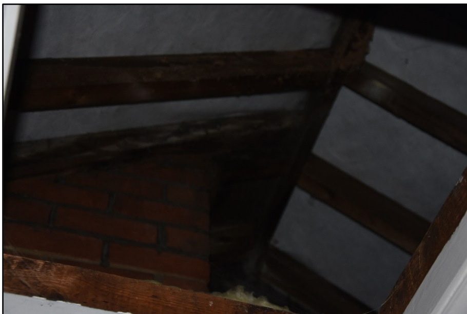
Roof structure over the rear range, accessed from FF09, looking east Fig 115
