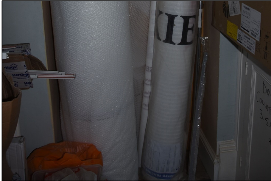
Detail of the skirting to the blocked aperture in GF02, looking north-west Fig 28
