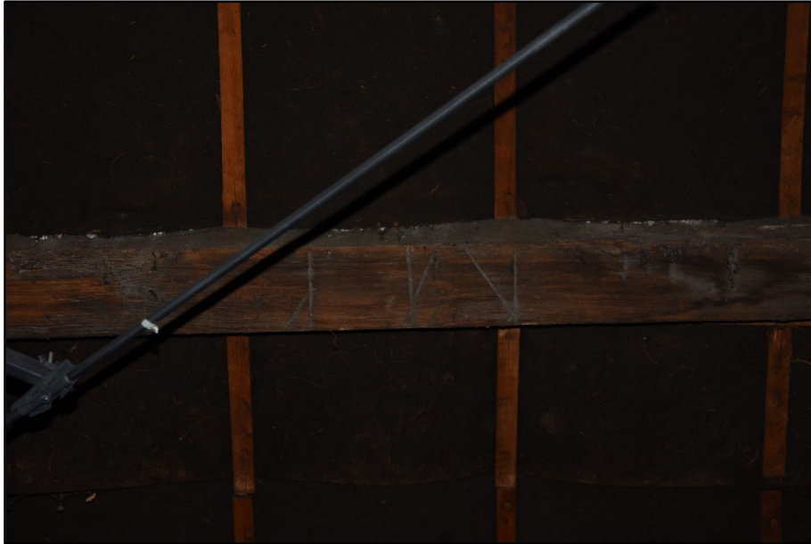
Suspected Baltic mark in the roof structure over the main range, looking north
