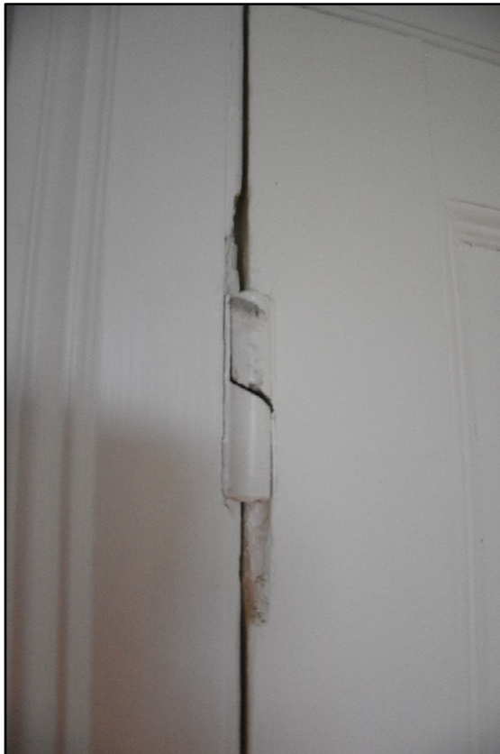
Swivel hinges on the door to FF03, looking north Fig 78
