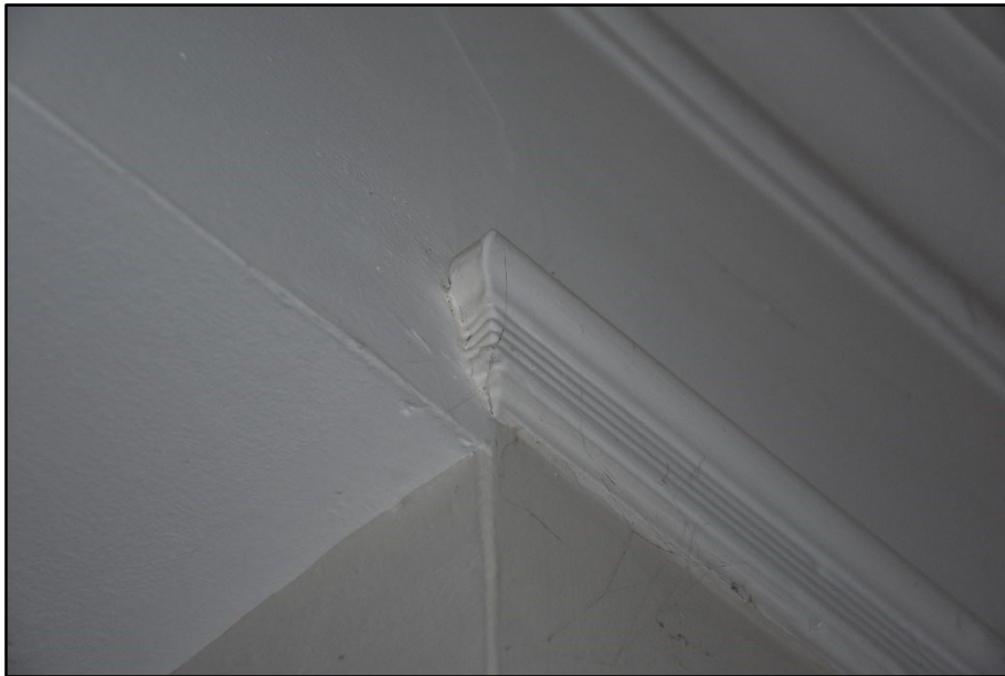
Picture rail returning along the partition between GF04 and GF05, looking west
