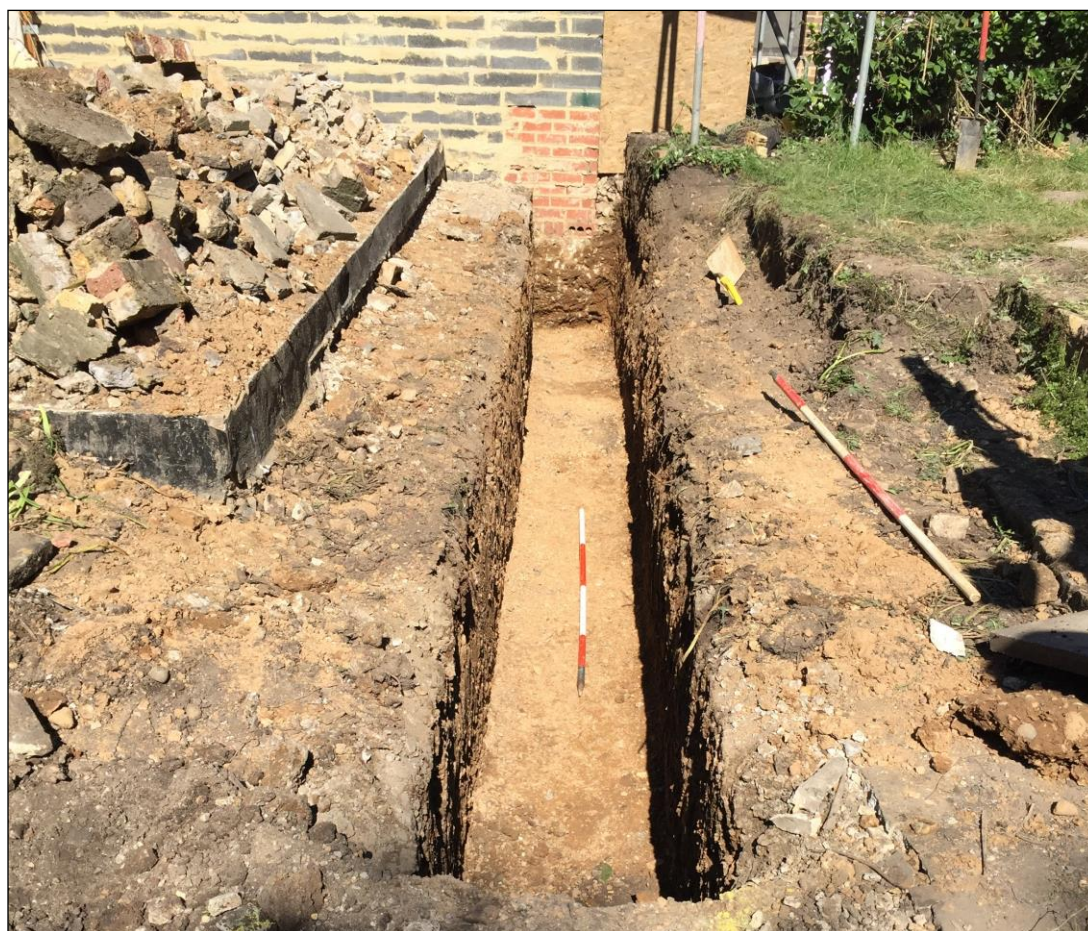
Figure 4. Footings in the east. The natural deposits in the trench showed no traces of archaeological remains. North facing photo.
