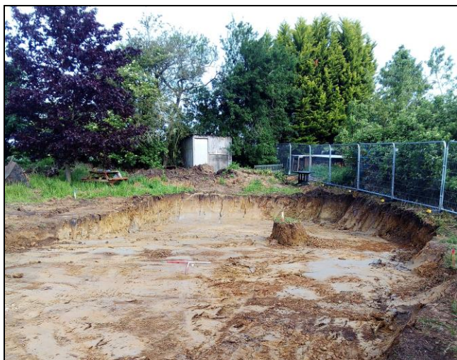
Figure 4. The ground in the northern parts of the development area was slightly higher, and in order to level the ground it was necessary to dig up to 1m into the natural deposits. Plot 1 from south.
