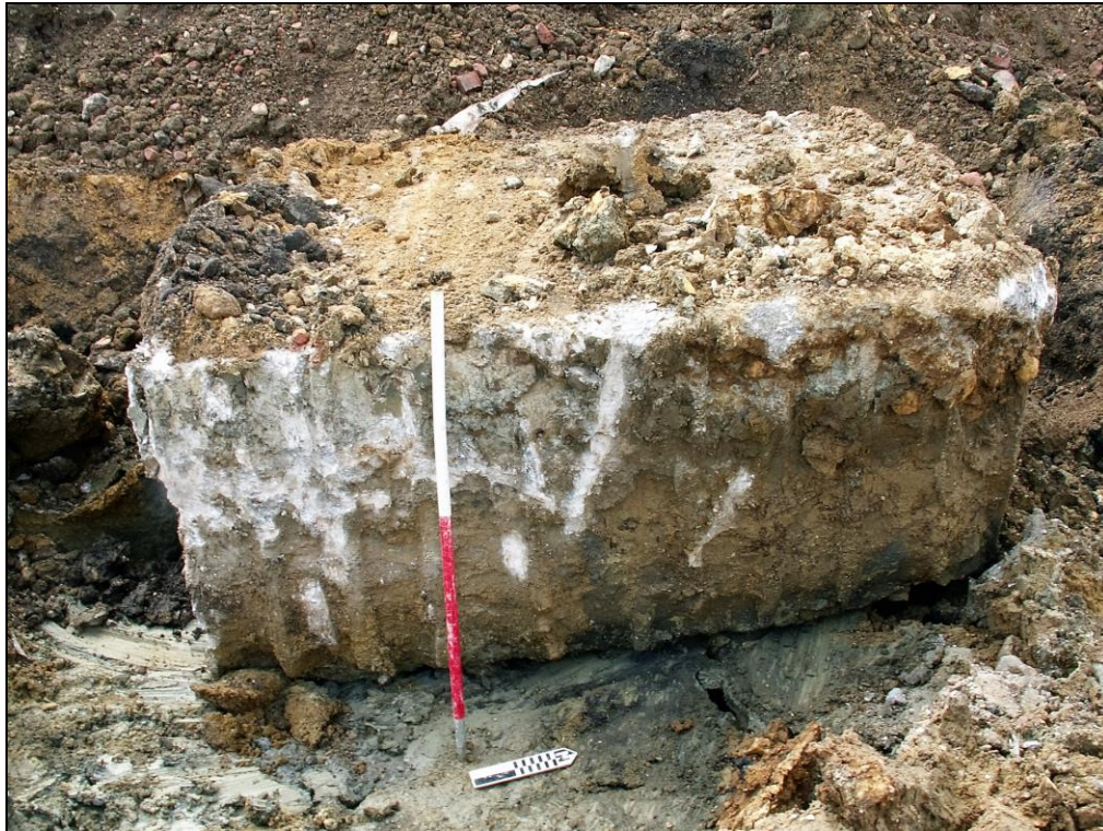
Figure 8. Massive pieces of concrete from the demolished warehouse were sometimes reaching far into the natural deposits of the site.
