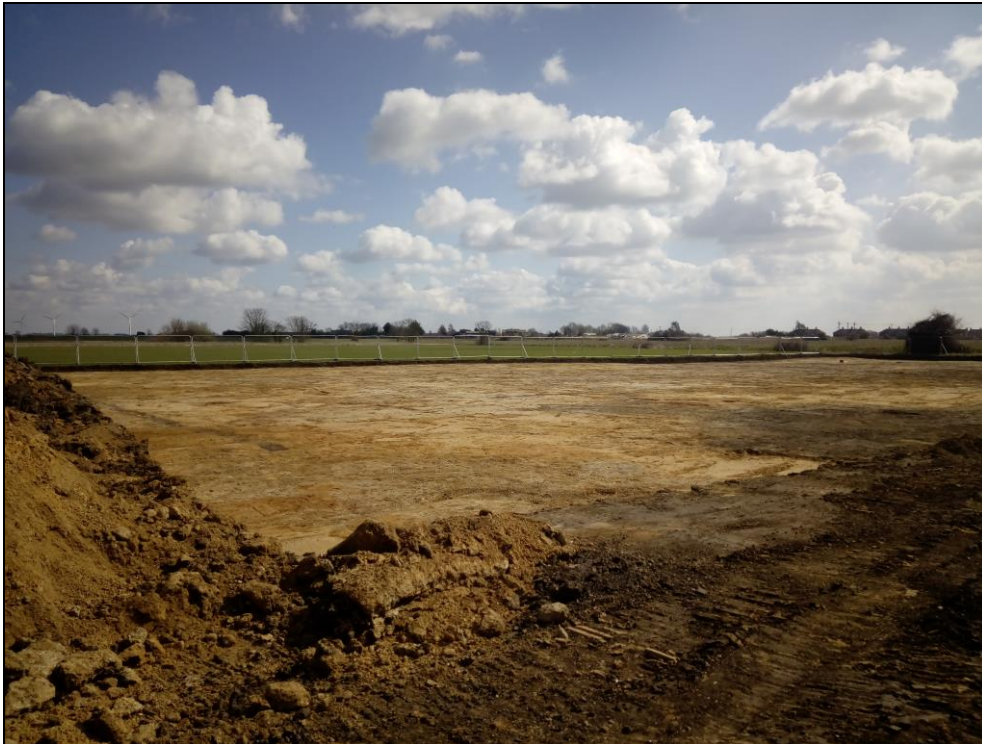
Figure 3. Overview of the southern part of the site after stripping. This part of the site contained a large number of pits, ditches and some ponds.
