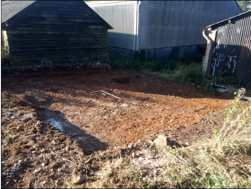
Figure 6. The stripping of overburden in Area 2 revealed the lower parts of a former brick boundary wall and a medieval ditch. Photo from north.
